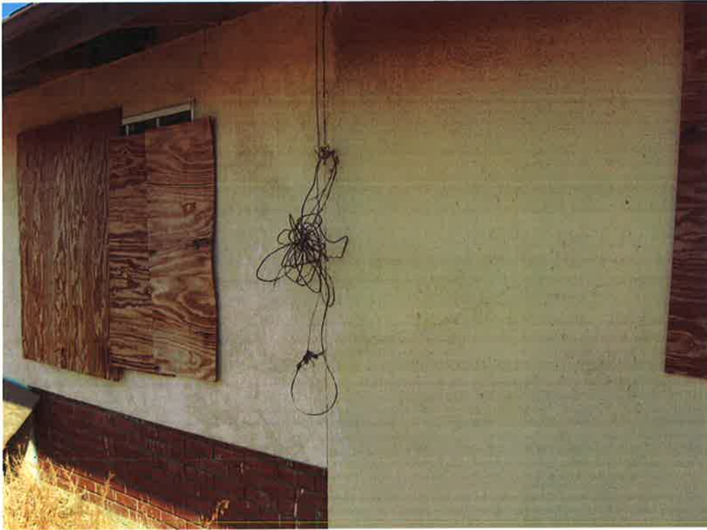
Photo 9: Structure #1 Defects 6,14, 17 Note the bundle of wires hanging on the exterior of the structure
