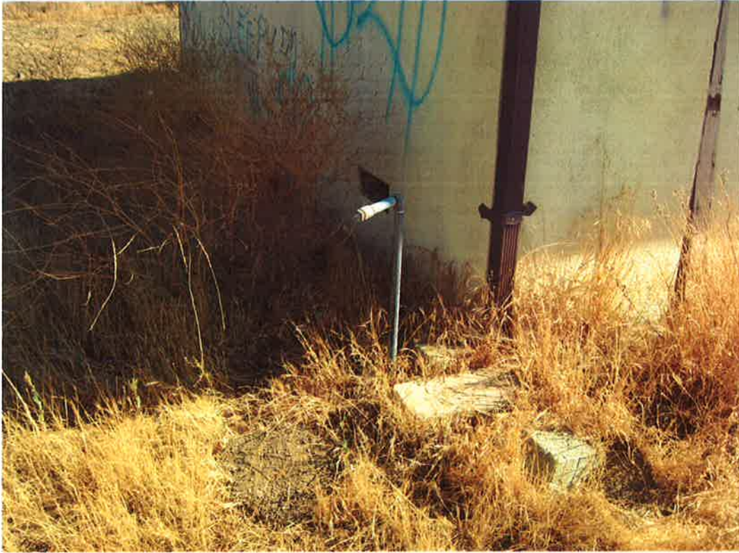
Photo 11: Structure #1 Gas meter appears to have been removed
