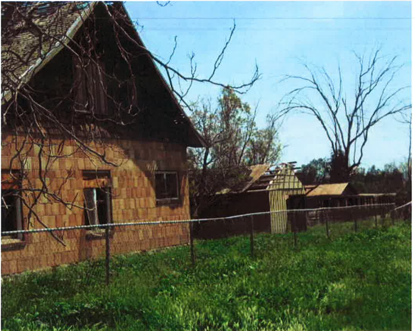
E. Torres; Structure 3 remains in substandard condition - 03/24/2010
