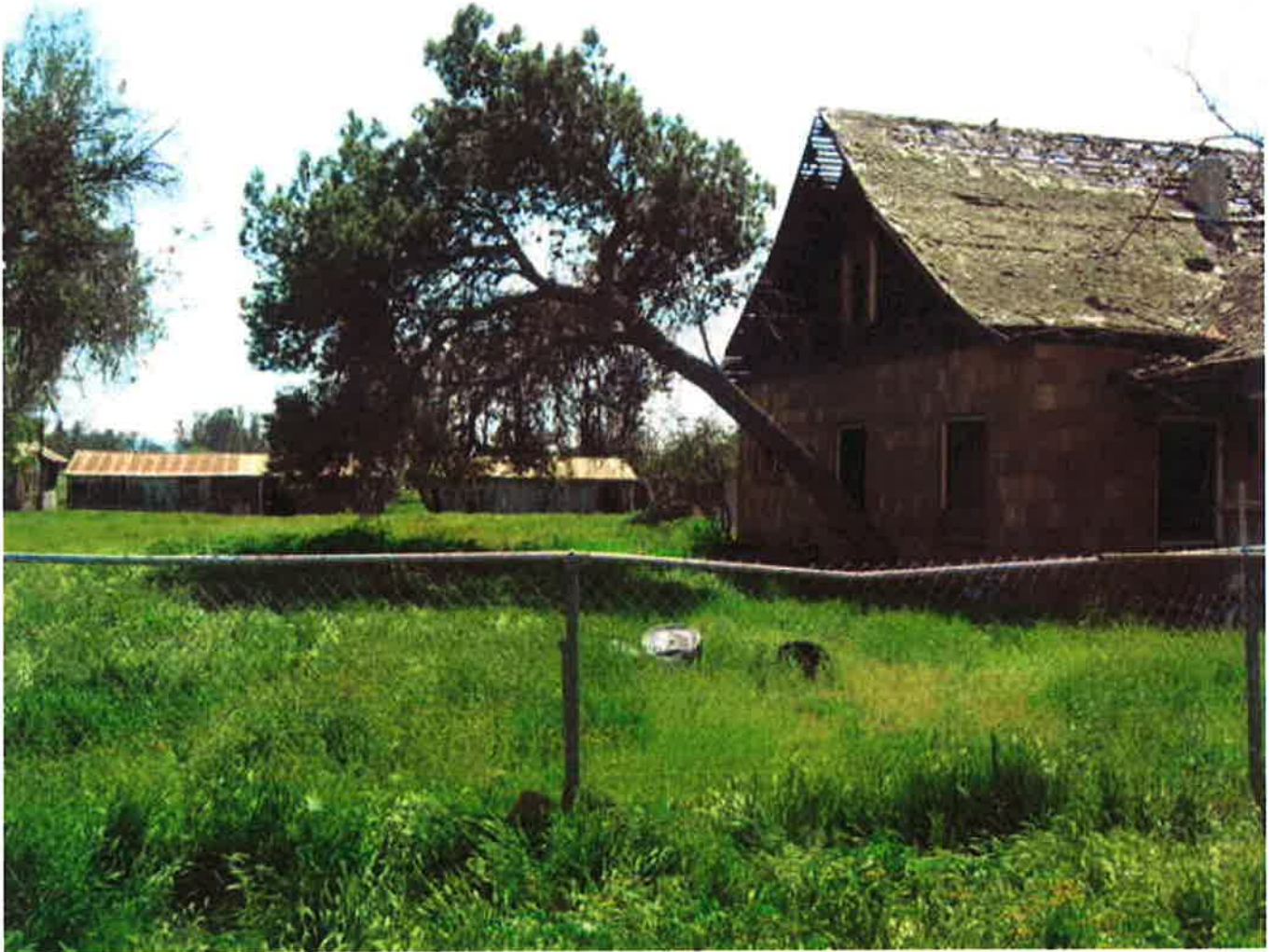
E. Torres; Structure 5 remains in substandard condition - 03/24/2010
