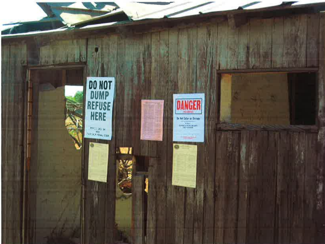
Photo 28: Structure #4 Defects 10, 11, 12, 13, 14, 17 Postings
