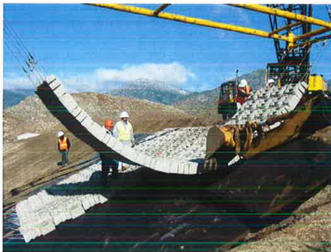
Kern Valley Sanitary Landfill GeoSyntec designed and provided CQA services for the concrete- reticulated block embankment protection system.
