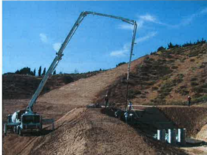
Lebec Landfill GeoSyntec designed, permitted, and provided CQA services for closure of the Lebec Landfill.
