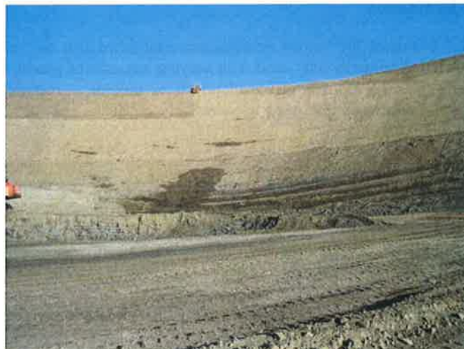
Lamb Canyon Landfill – A Seep was Discovered during In-Grading Monitoring. GeoSyntec assessed Seep Impact on the Composite Liner and subsequently Designed an Underdrain System
