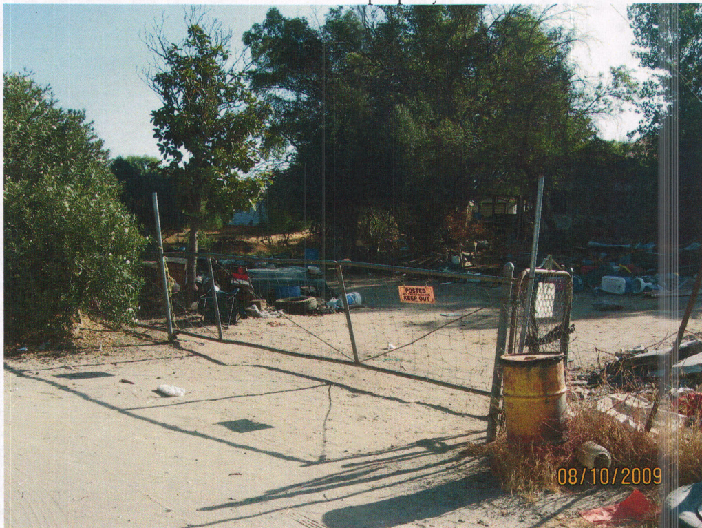
PHOTO # 4 NOTES: Violations remain on the property
