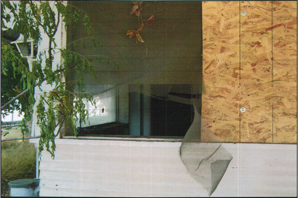
PHOTO #1 Open window on S side of dwelling.
