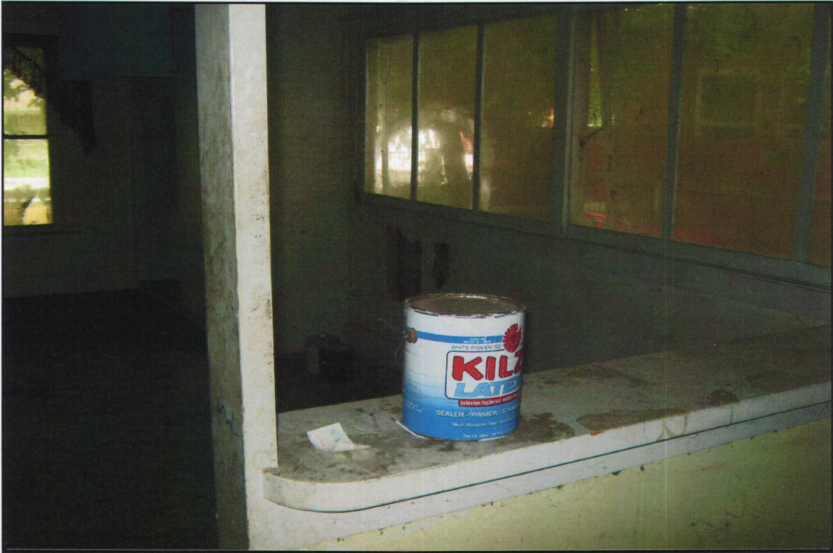
PHOTO #5 Condition #10, Members of walls split.
