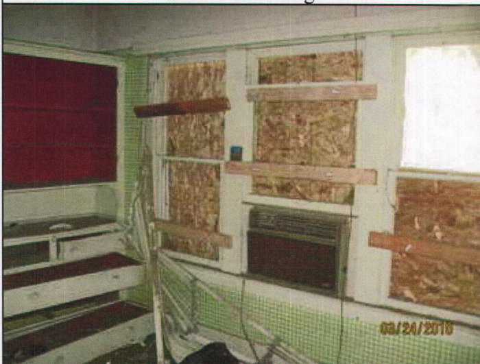
M Sanders 024510 SSS # 1 - missing windows
