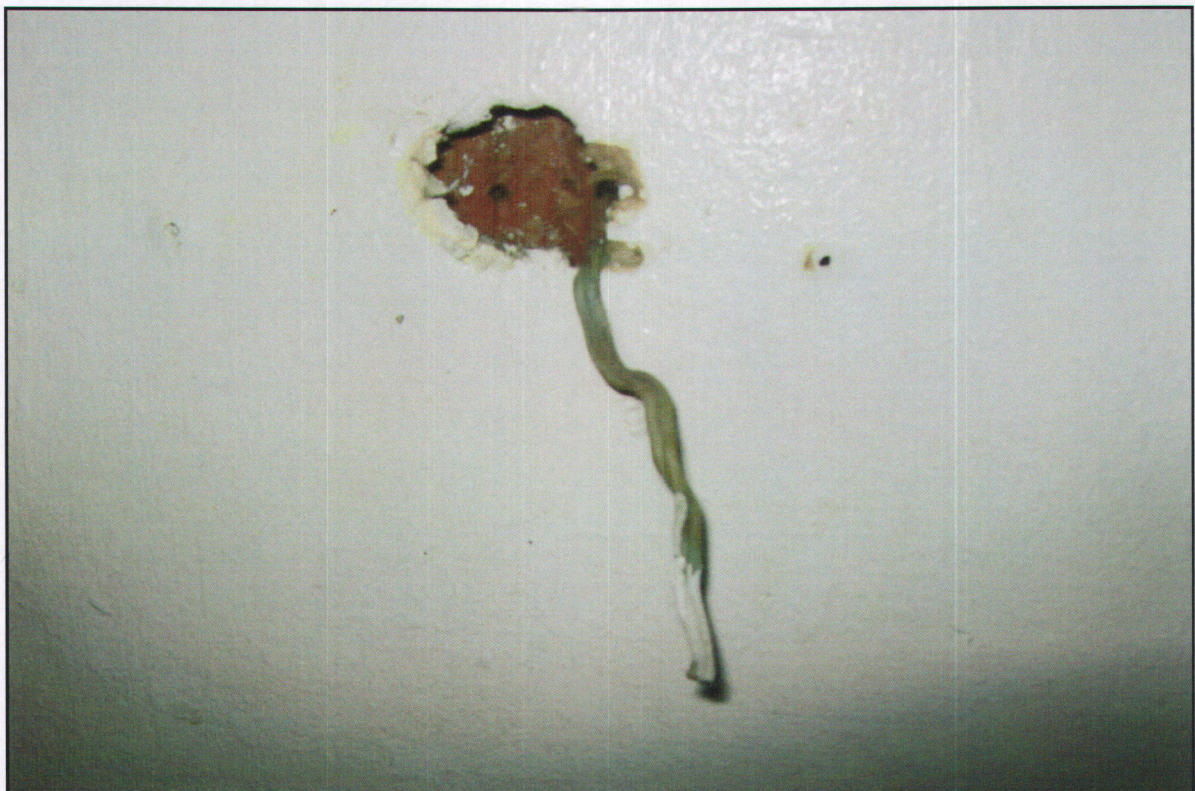
PHOTO #4 Condition #6, Hazardous wiring.
