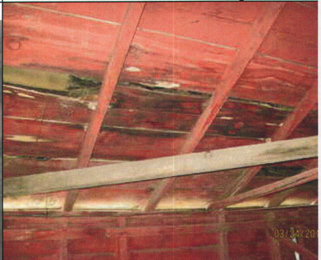
M Sanders 024510 SSS # 2 - faulty weather protection damage roof members
