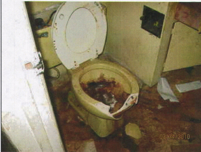
M Sanders 024510 SSS # 1 - vandalized toilet
