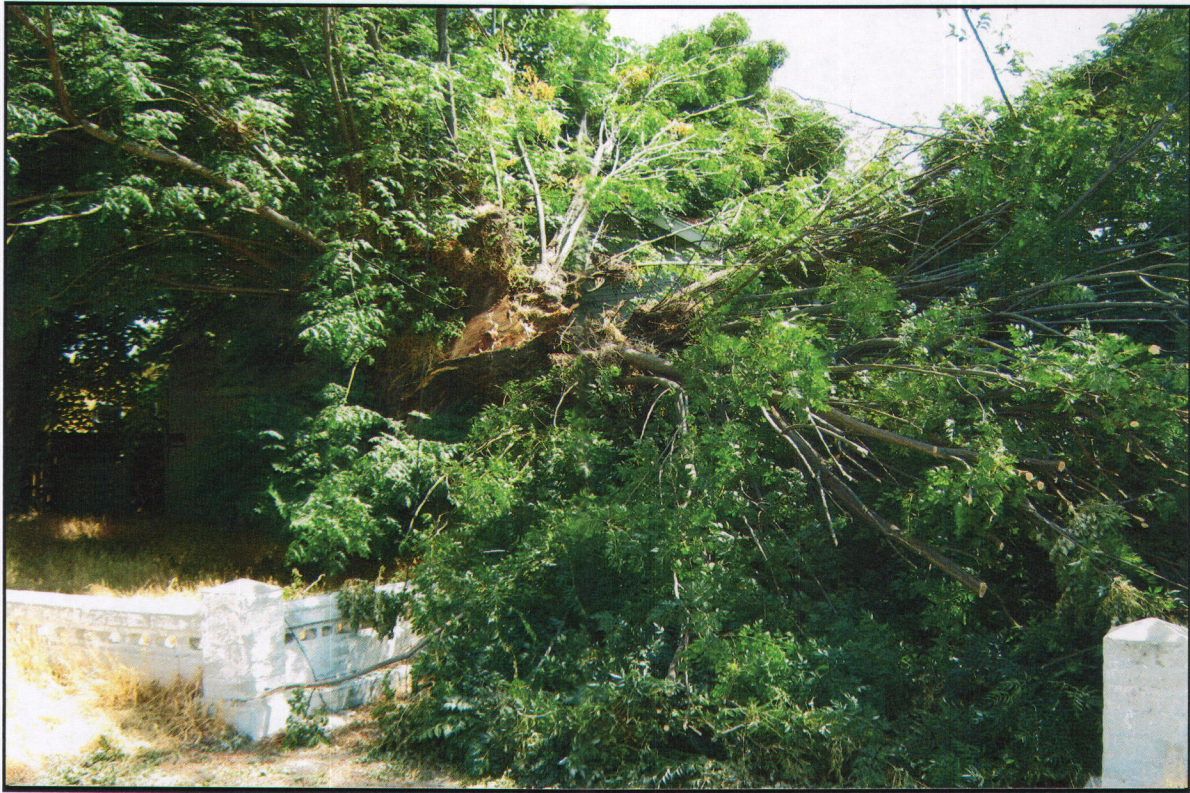
PHOTO #7 Split tree fallen in front yard and roof of dwelling.
