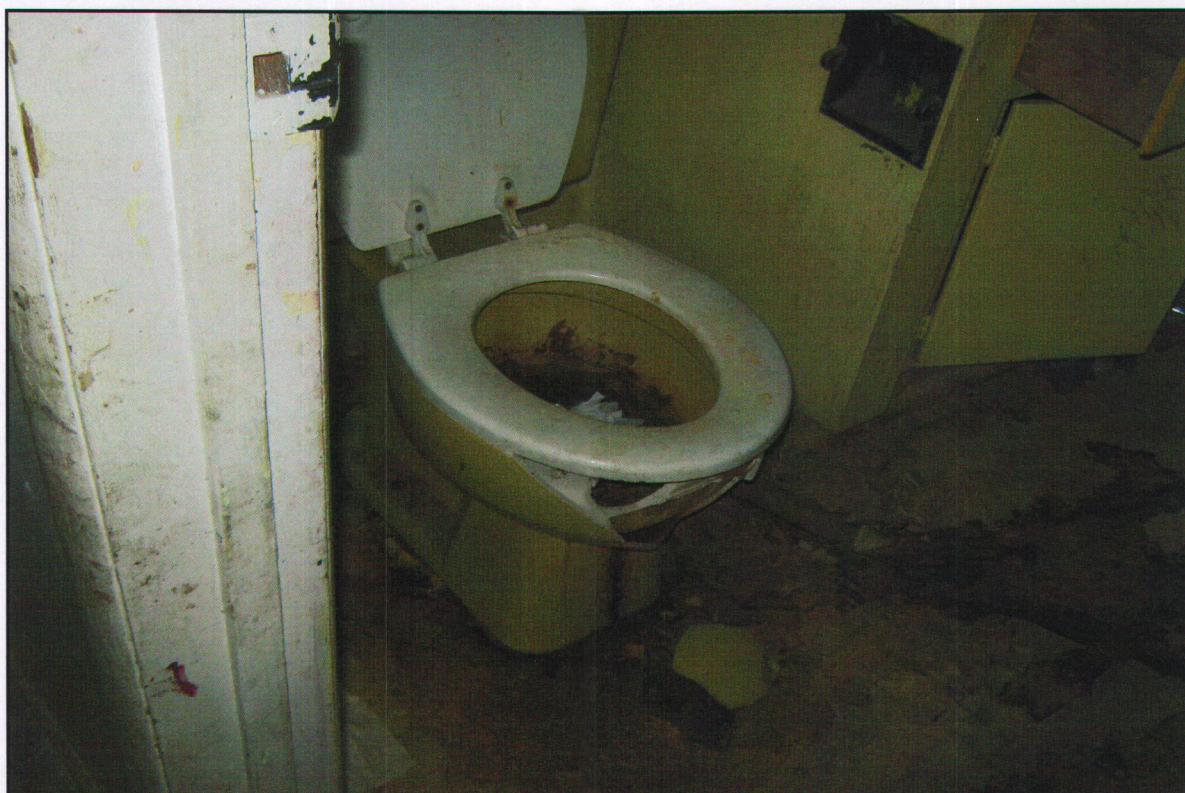
PHOTO #2 Condition #1, Improper lavatory.
