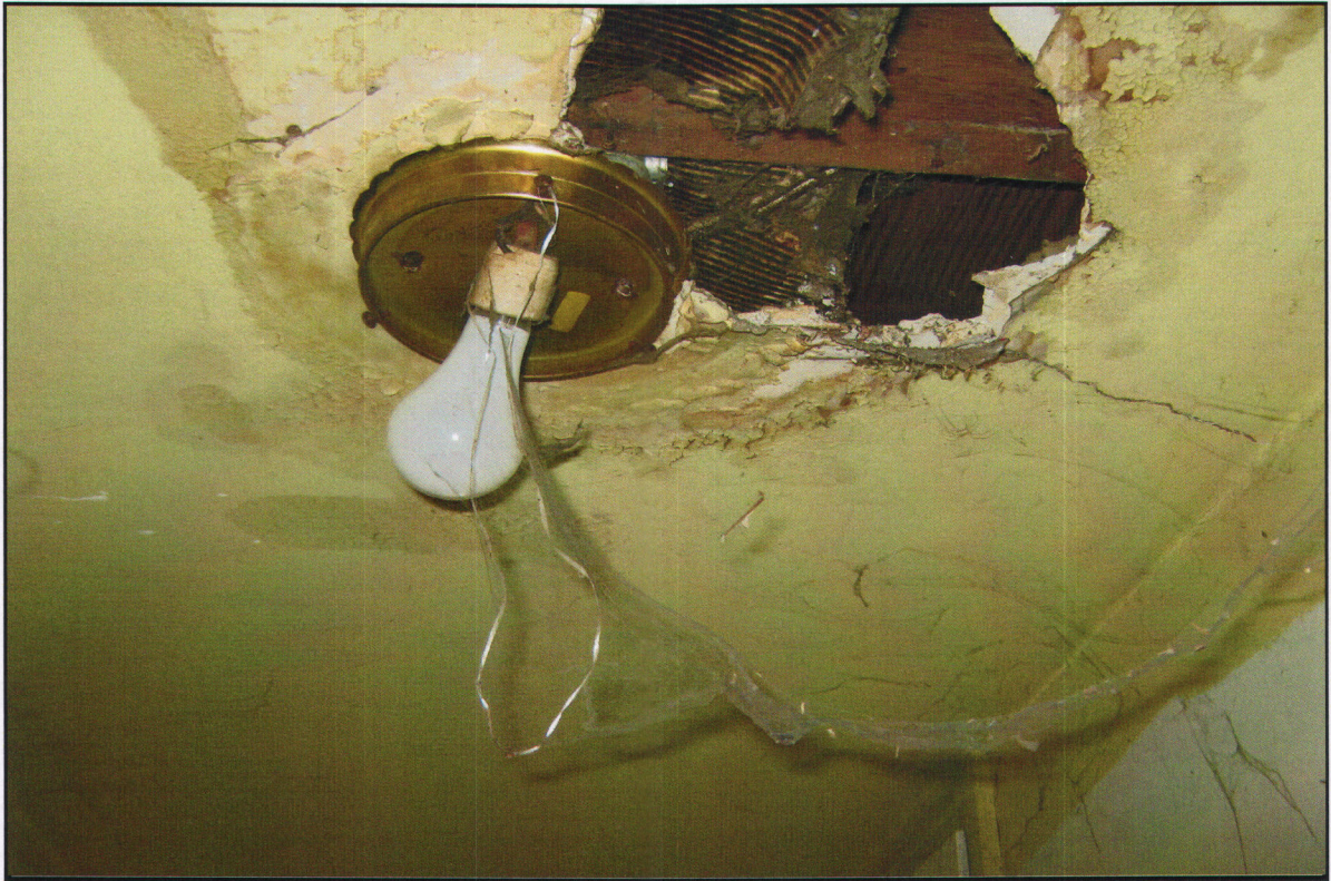
PHOTO #3 Condition #5, Lack of required electrical lighting.
