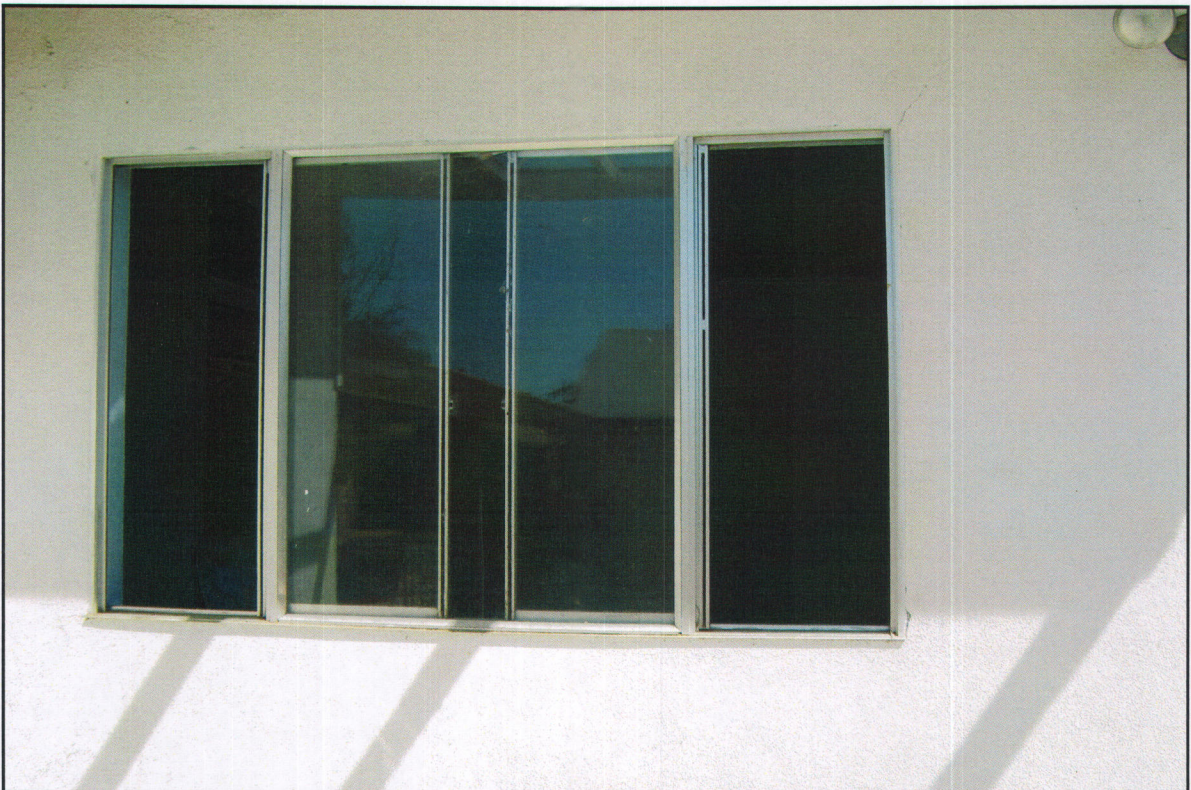
PHOTO #2 Open window on S side of dwelling.
