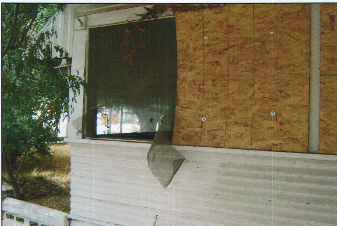
PHOTO #8 Condition # 13, Faulty weather protection, broken windows.
