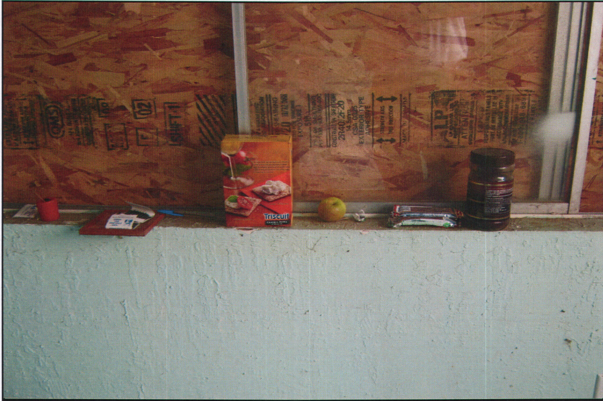
PHOTO #9 Condition #15, Fire hazard; note matches on window ledge.
