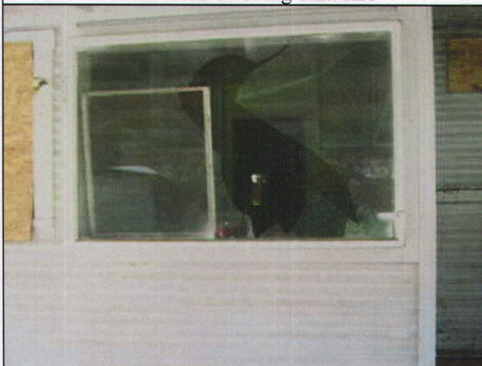
Broken window on rear of dwelling unit. KR
