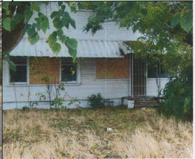
More broken windows in front of dwelling unit.
