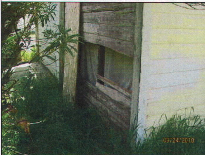
M Sanders 024510 SSS # 2 - missing horizontal members of exterior wall
