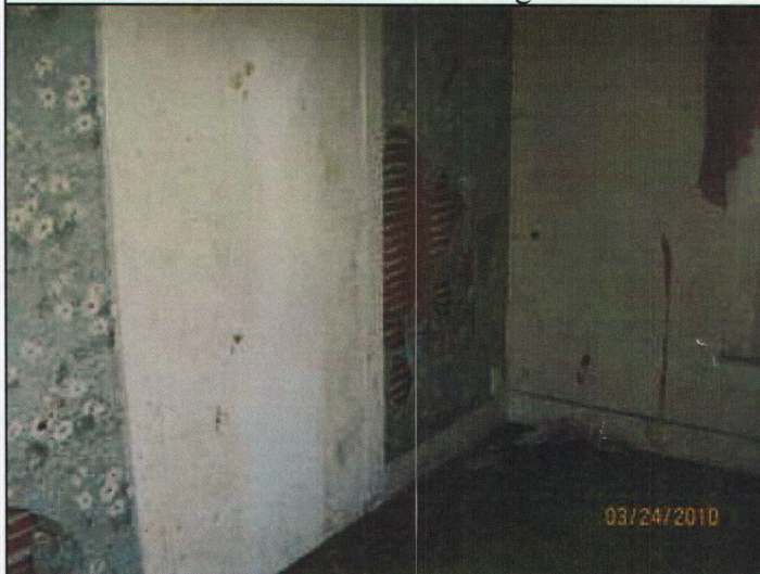
M Sanders 024510 SSS # 1 - additional damage to interior wall
