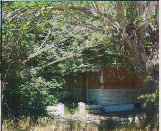
M Sanders 050410 - fallen tree on roof
