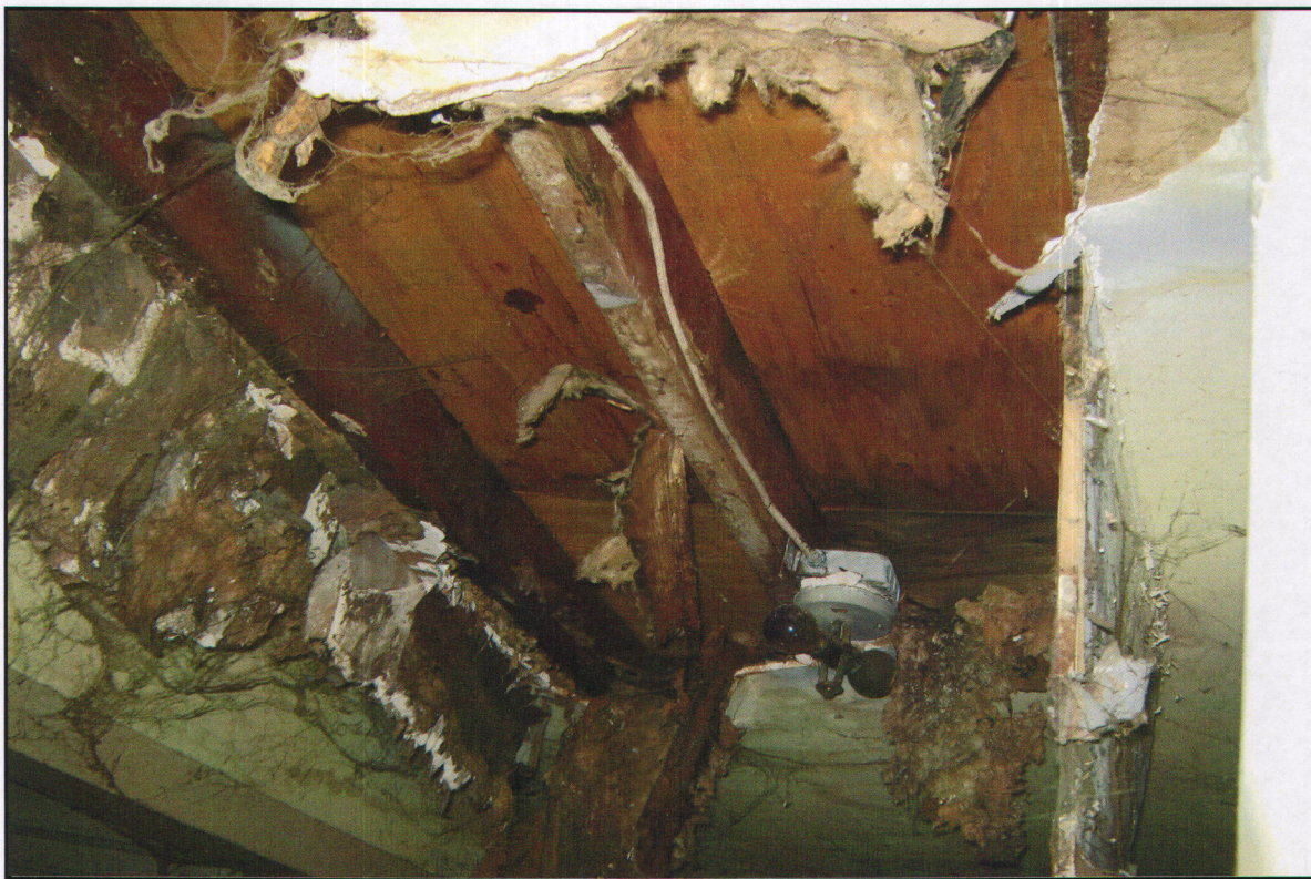
PHOTO #7 Condition #12, Dampness of habitable room.
