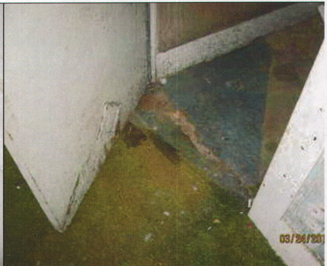
M Sanders 024510 SSS # 1 - deteriorated floor
