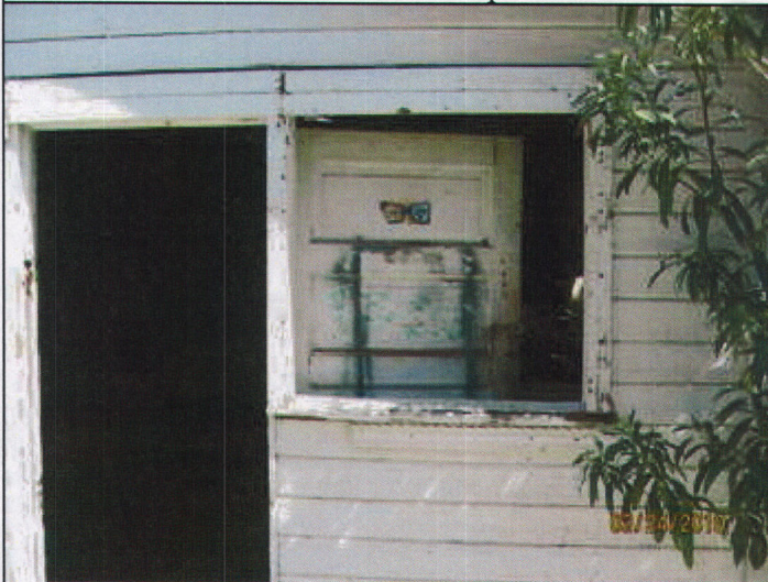
M Sanders 024510 SSS # 2 - missing window and lack of maintenance
