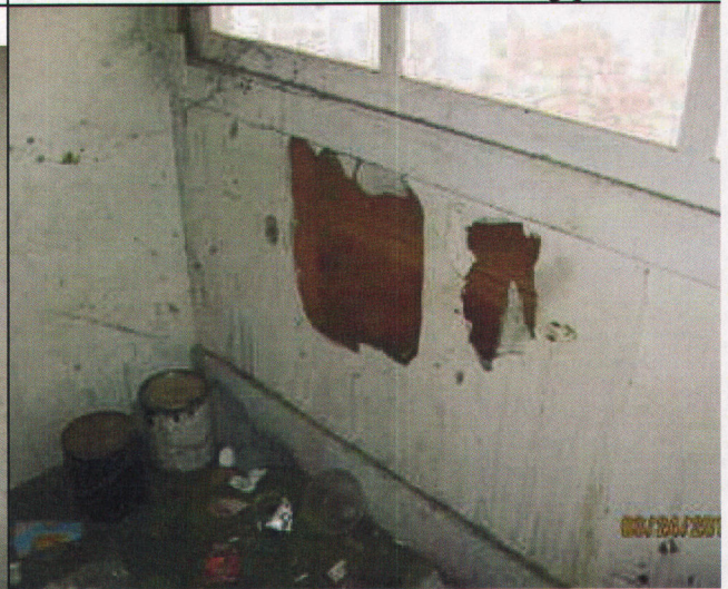
M Sanders 024510 SSS # 1 - additional damage interior wall
