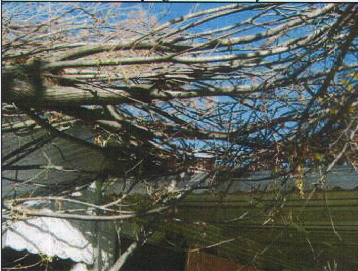
Dying tree limbs resting on roof of dwelling unit. KR
