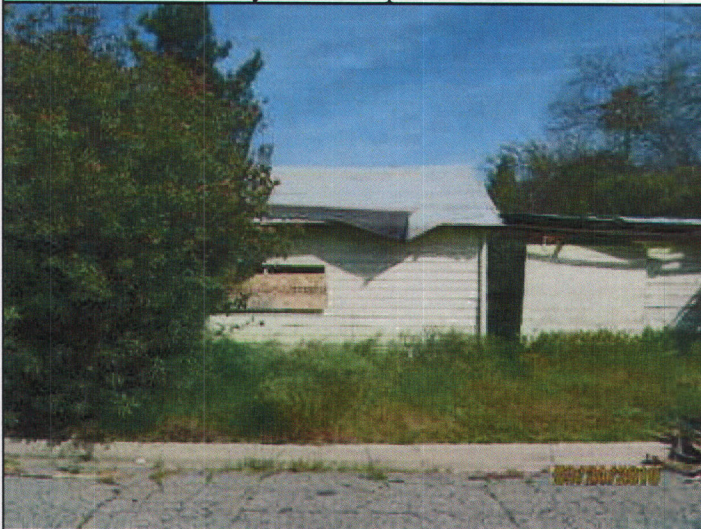
M Sanders 024510 SSS # 1 - dilapidated roof and roofing material
