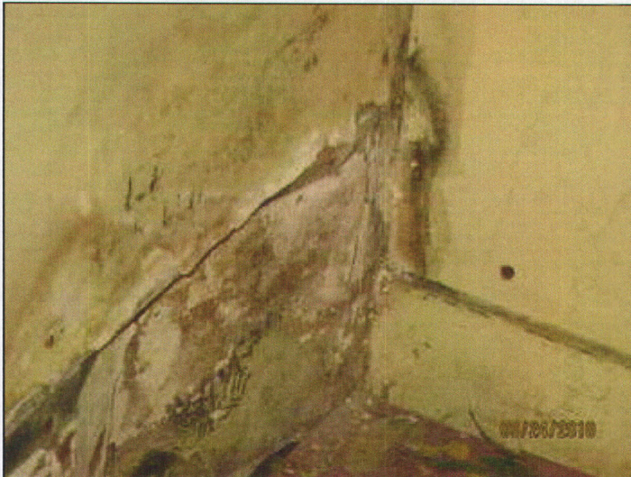
M Sanders 024510 SSS # 1 - water damage and mold
