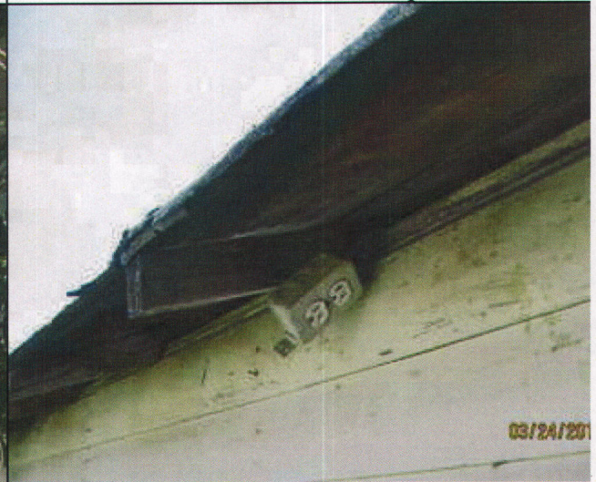
M Sanders 024510 SSS # 2 - unsecured electric outlet, no protective conduit for wiring
