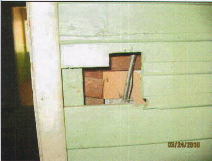
M Sanders 024510 SSS # 1 - damaged wall exposing electrical wiring
