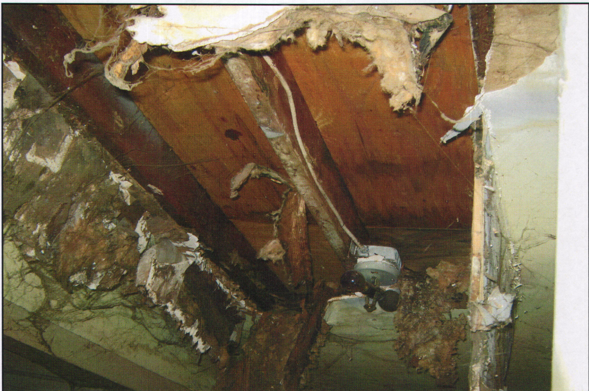
PHOTO #6 Condition #11, Members of ceiling deteriorating.
