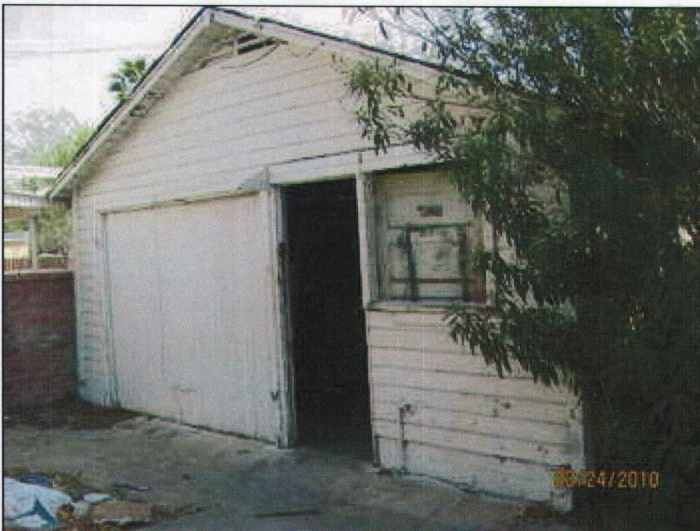
M Sanders 024510 SSS # 2 - unsecured, public and attractive nuisance
