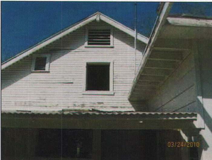
M Sanders 024510 SSS # 1 - missing attic cover, faulty weather protection
