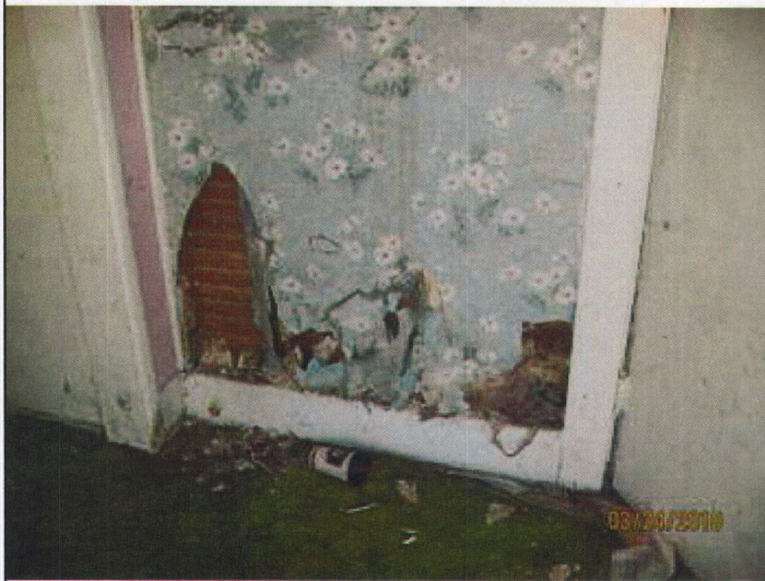
M Sanders 024510 SSS # 1 - damaged interior wall
