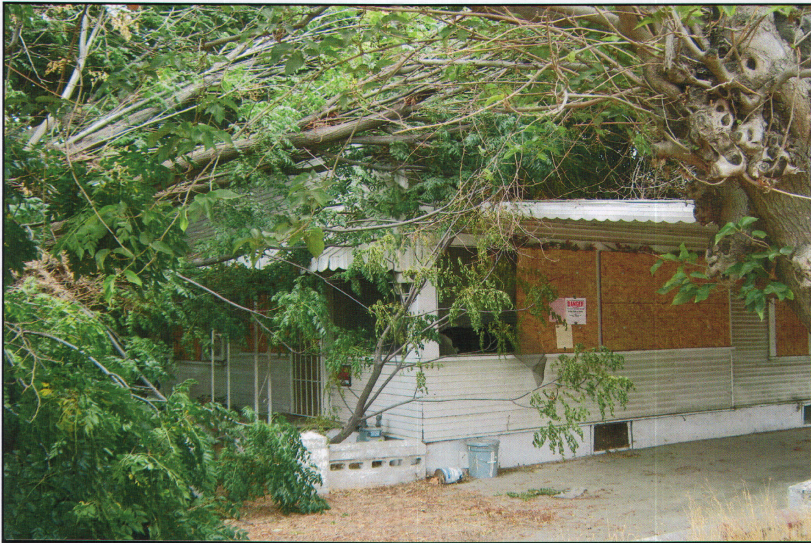
PHOTO #11 Posting of NOV, NOD & DANGER sign.
