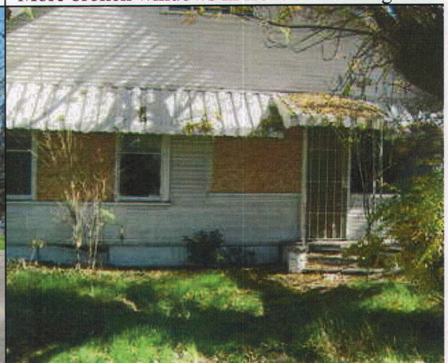
Broken windows in front of dwelling unit. KR
