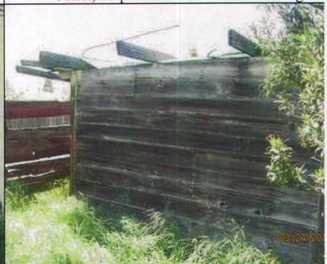
M Sanders 024510 SSS # 2 - deterioration due to of paint
