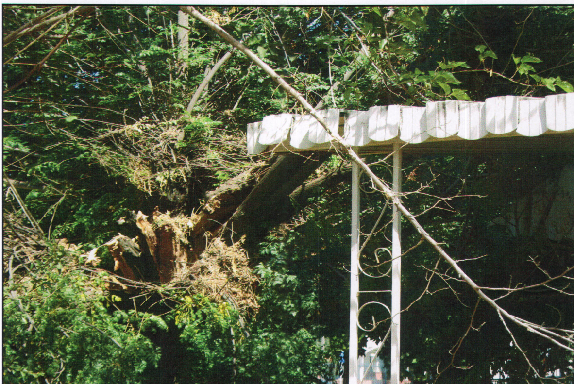
PHOTO #6 Front of dwelling E side with fallen tree on roof.
