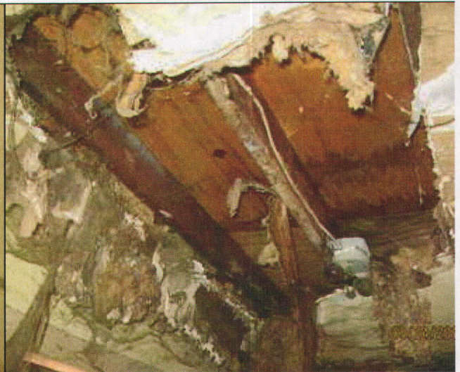
M Sanders 024510 SSS # 1 - ceiling pulled down
