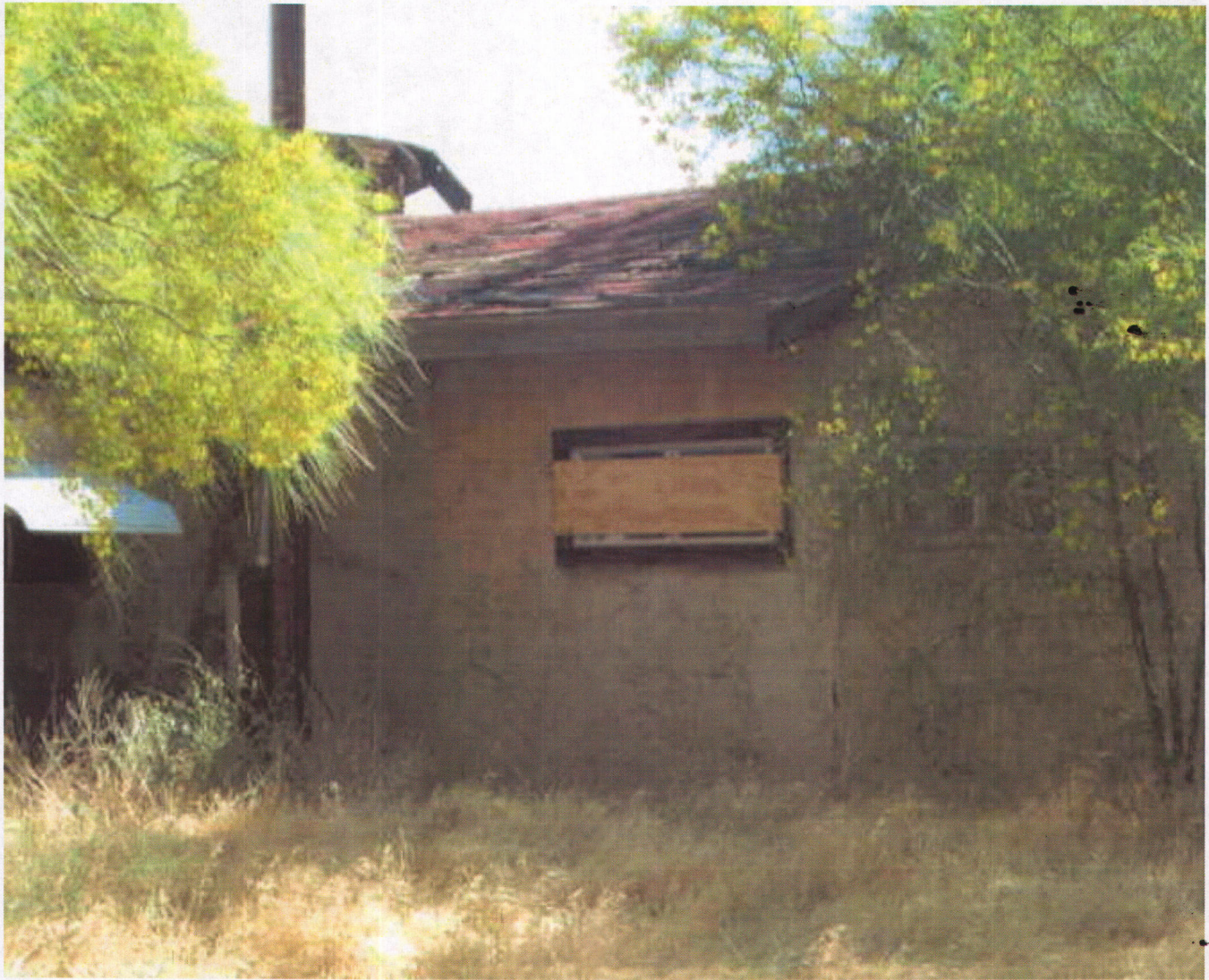
Substandard Structure remains - Taken by R. Keyes 6/3/2010 - 06/03/2010
