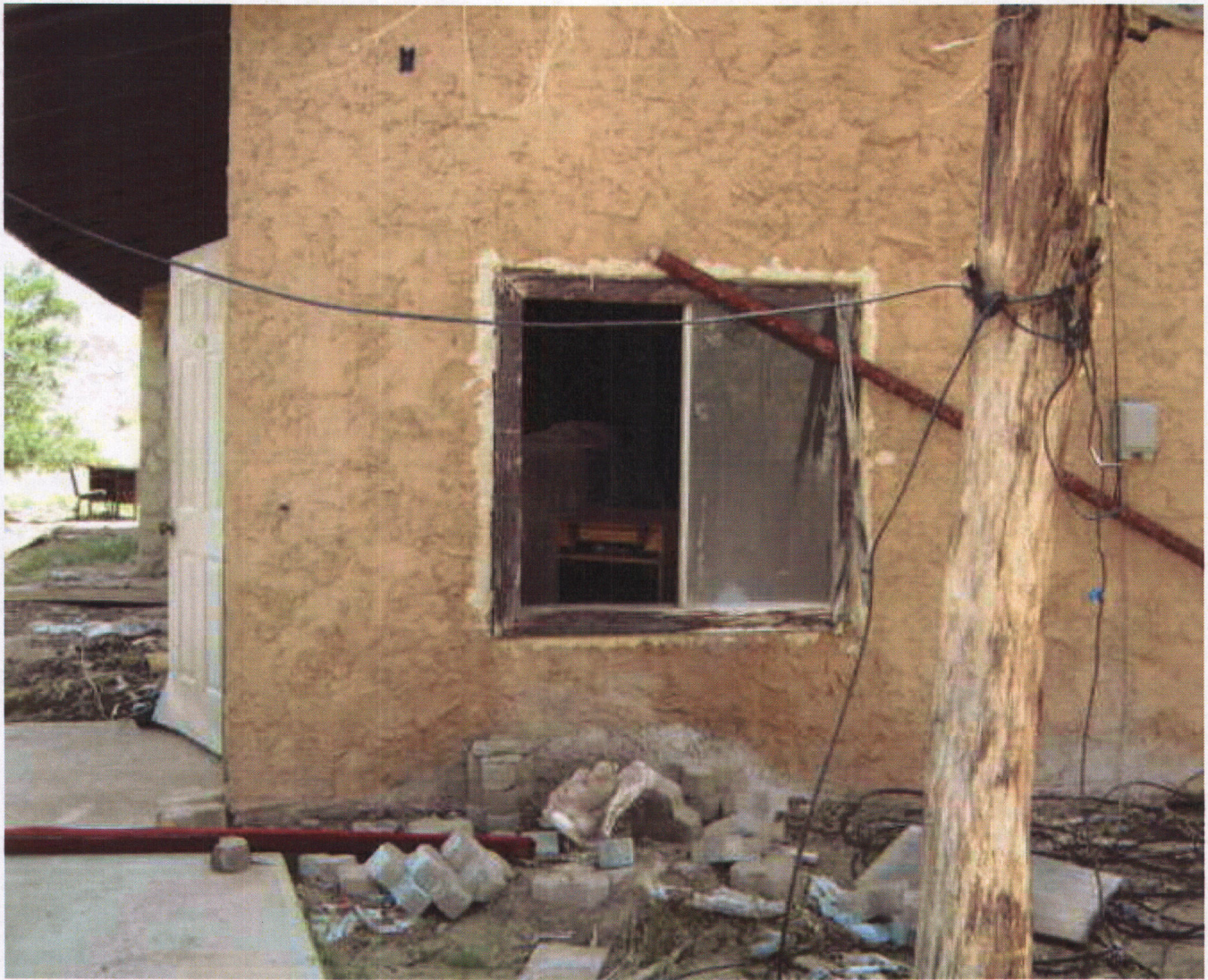
List of Defect # 10, 12, 13, 14, 17 Taken by L. Padilla 4/10/2010 - 04/10/2010
