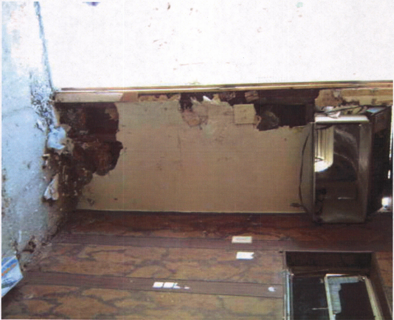
List of Defect # 10, 13, 14, 17 Taken by L. Padilla 4/10/2010 - 04/10/2010
