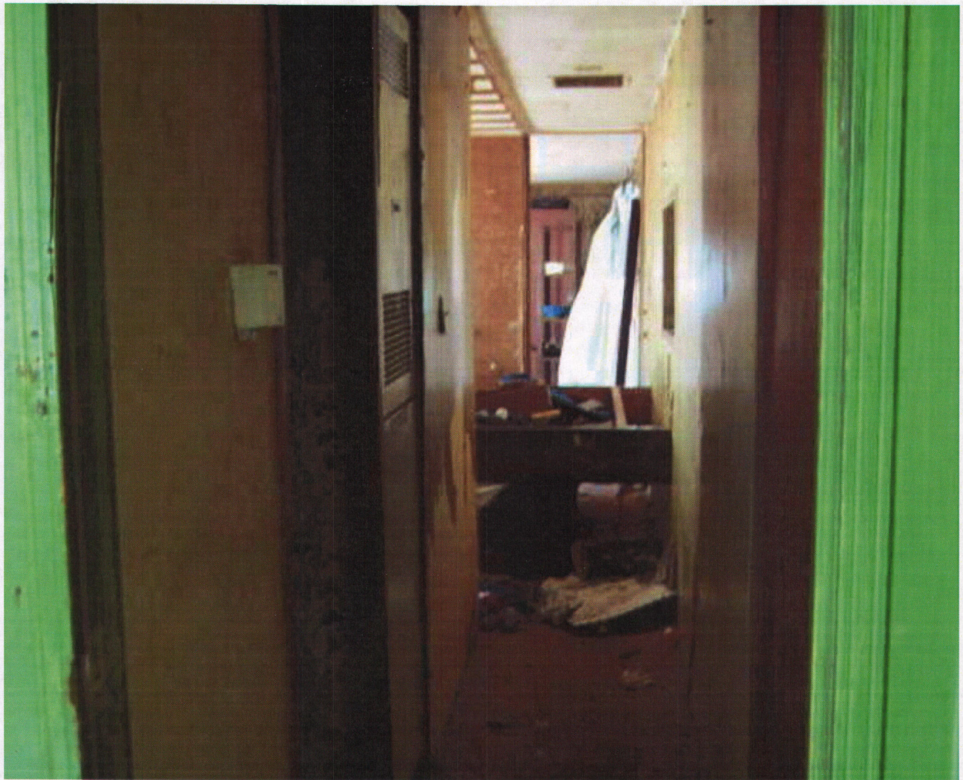
List of Defect # 8, 12, 13, 14, 17 Taken by L. Padilla 4/10/2010 - 04/10/2010
