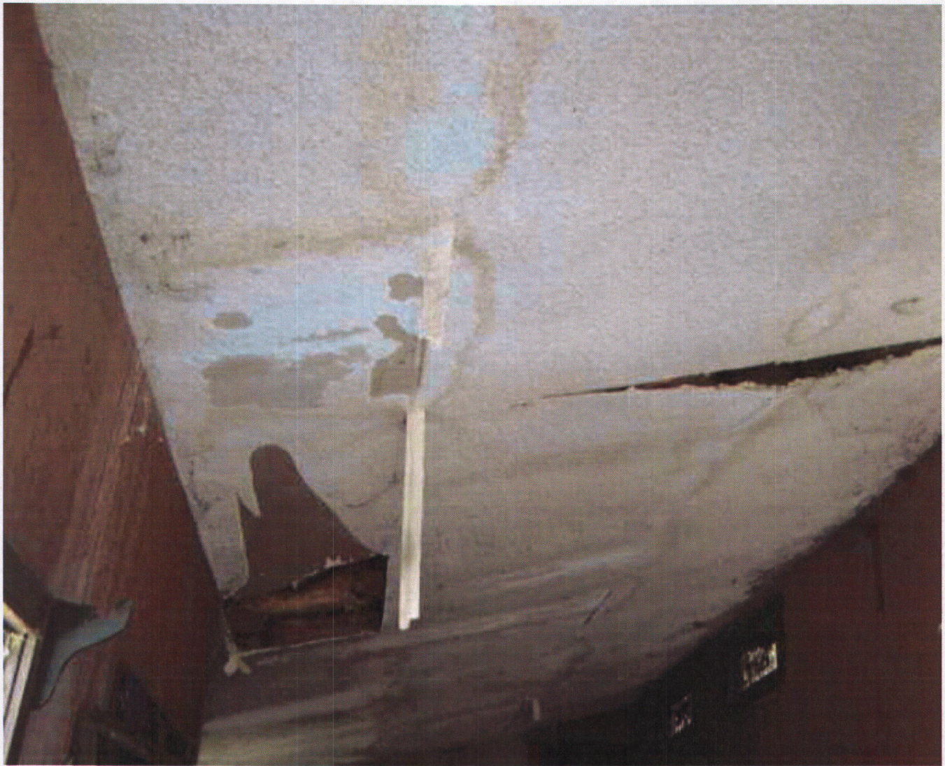
List of Defect # 10, 11 13, 14, 17 Taken by L Padilla 4/10/2010 - 04/10/2010
