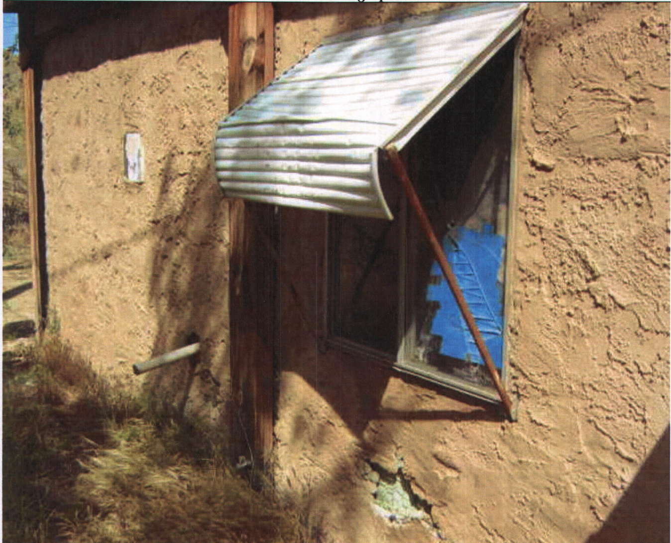
List of Defect # 10, 13,14, 17 Taken by L. Padilla 4/10/2010 - 04/10/2010
