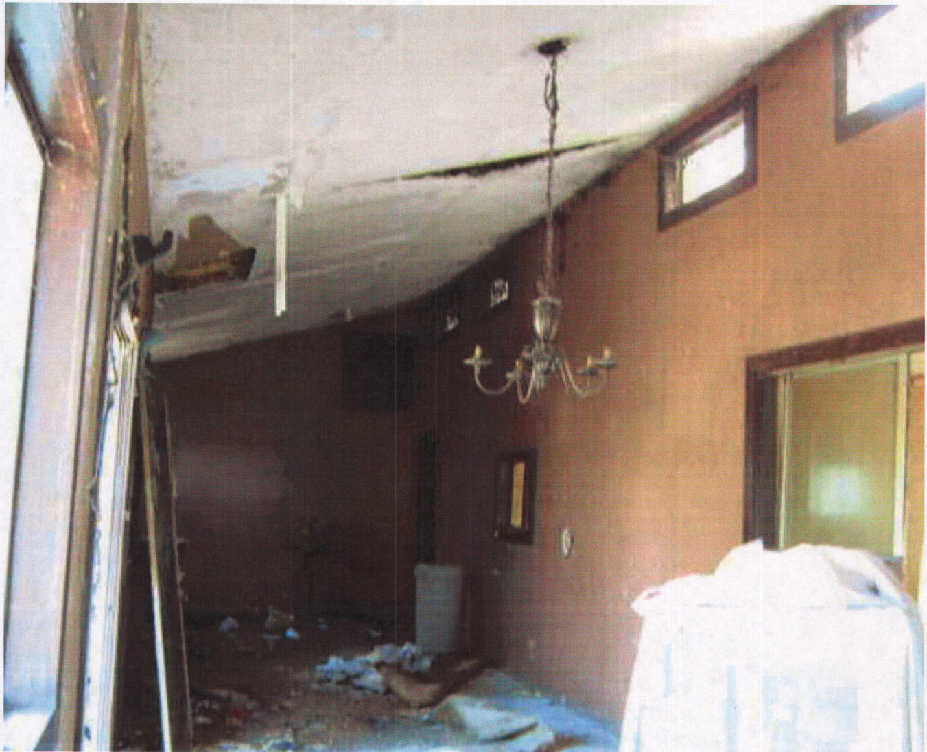
List of Defect # 6,10, 11, 13, 14, 17 Taken by L. Padilla 4/10/2010 - 04/10/2010
