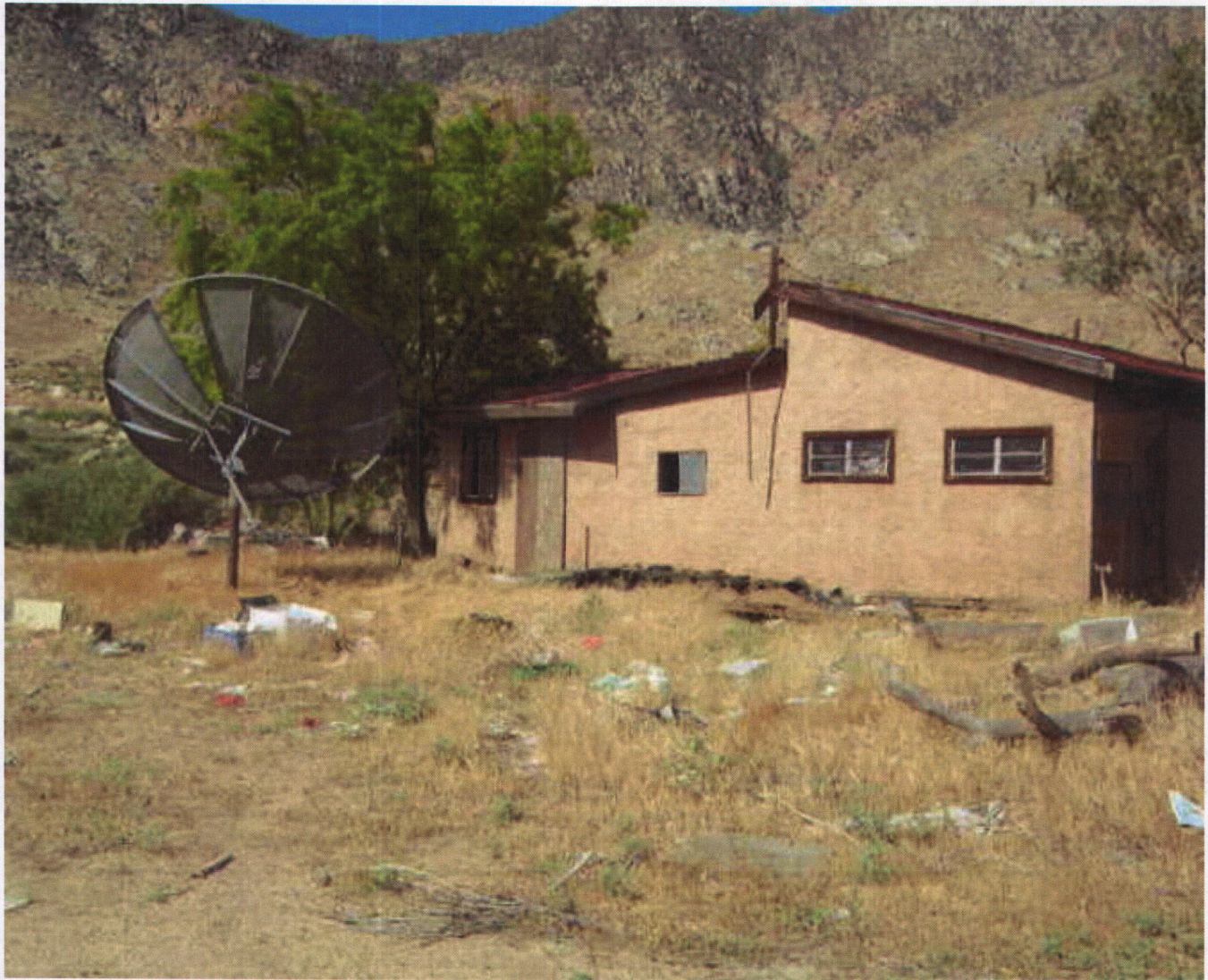
Substandard Structure remains Taken by R. Keyes 6/3/2010 - 06/03/2010
