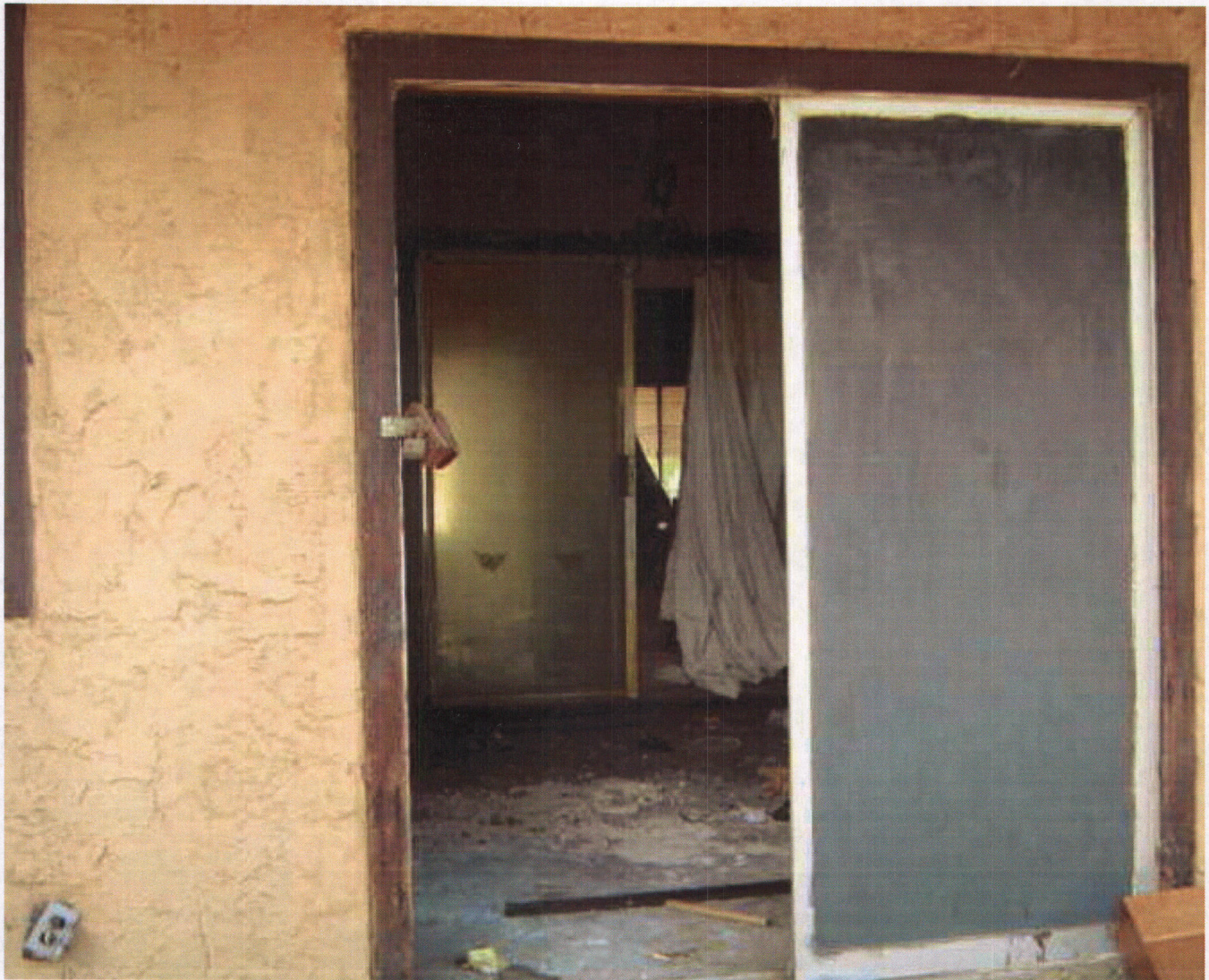
List of Defect # 8, 9, 12,13, 17 Taken by L. Padilla 4/10/2010 - 04/10/2010
