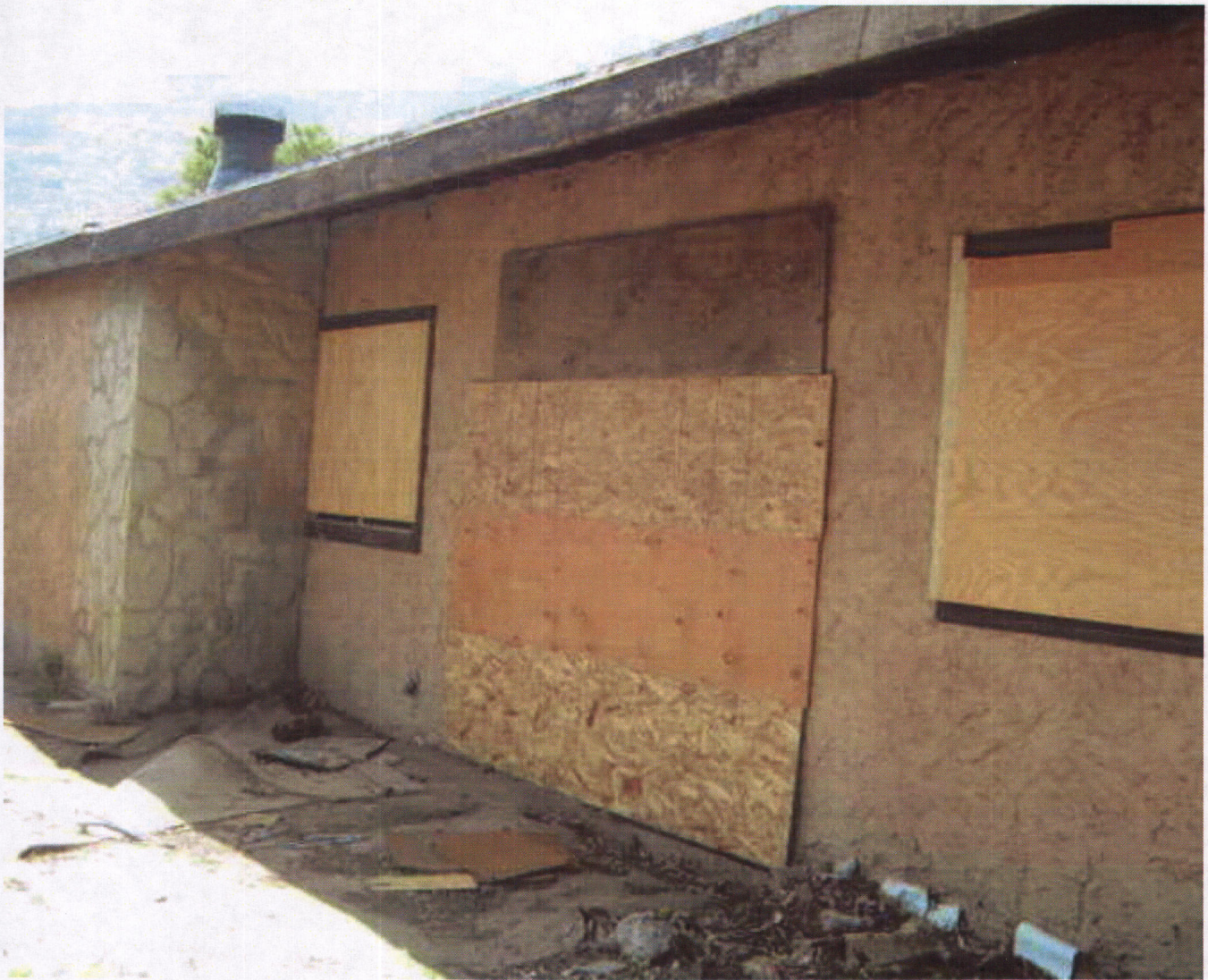
Substandard Structure remains - Taken by R. Keyes 6/3/2010 - 06/04/2010
