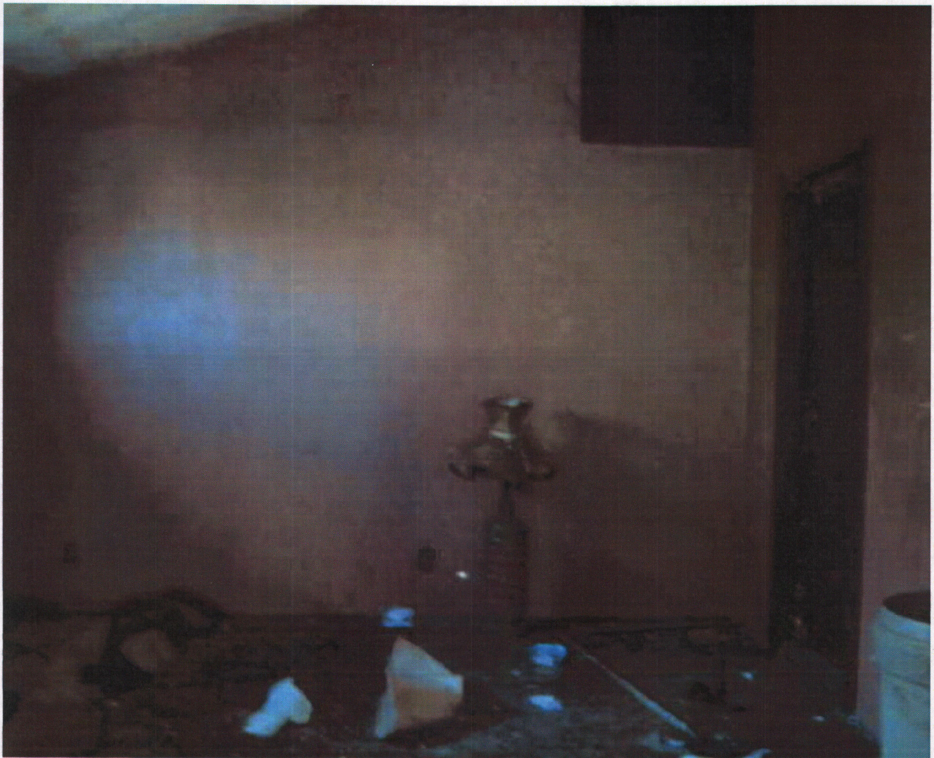
List of Defect # 4, 14, 17 Taken by L. Padilla 4/10/2010 - 04/10/2010
