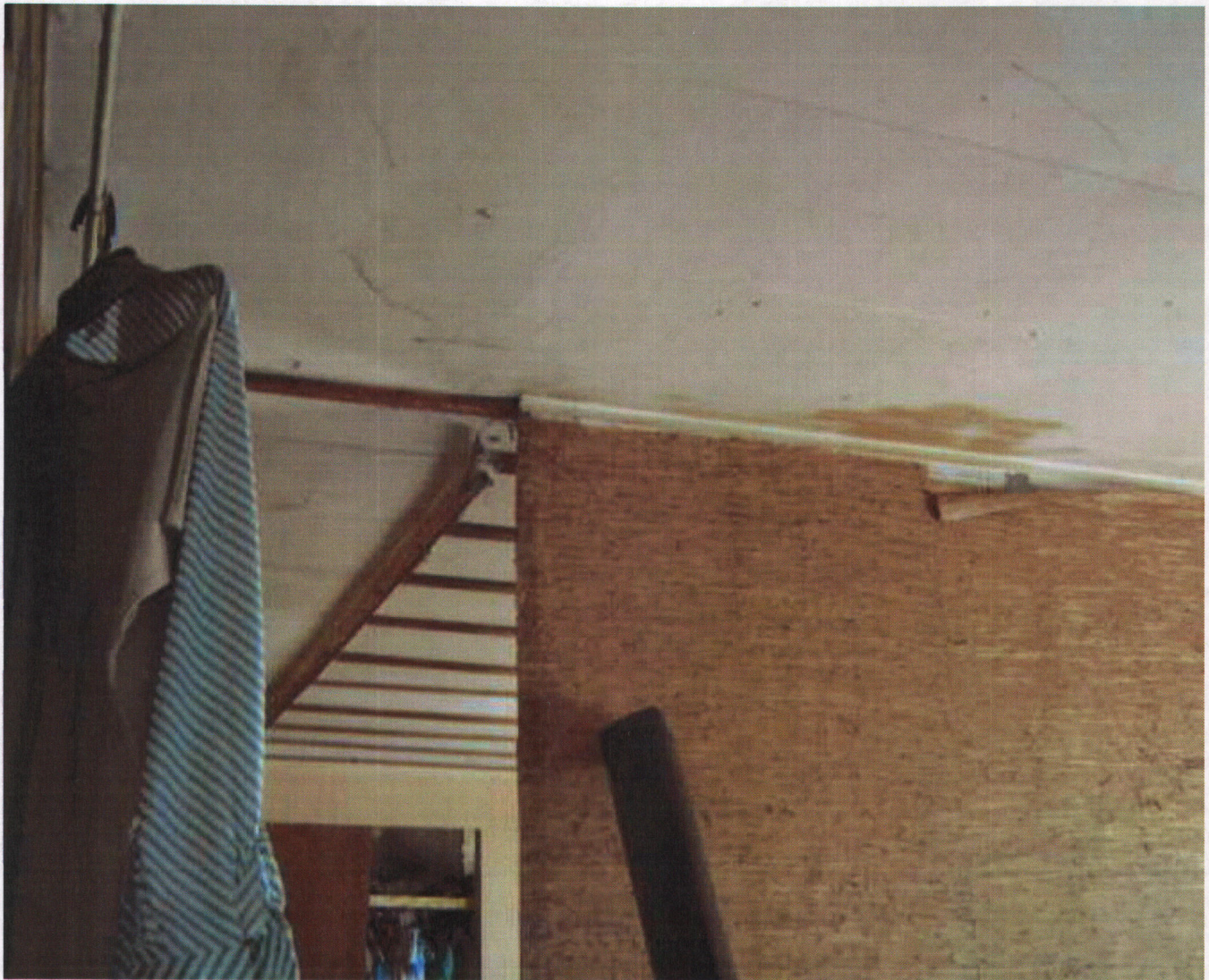
List of Defect # 11, 12, 13, 14, 17 Taken by L. Padilla 4/10/2010 - 04/10/2010
