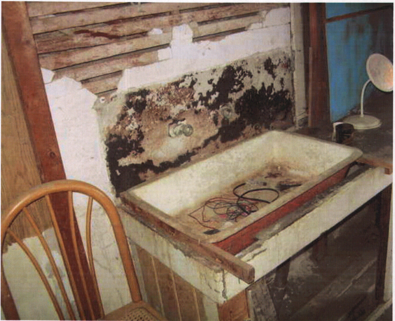
NO SINK. DEFECT #1 & 2. - 12/29/2010
