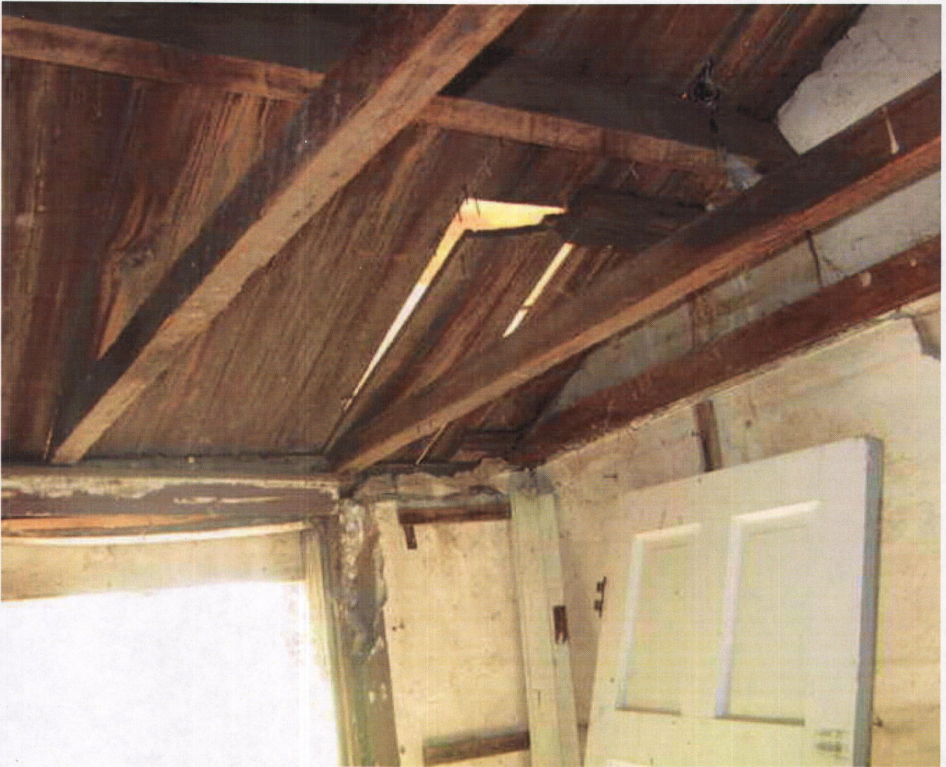
CEILING COMING APART. DEFECT #11. - 12/29/2009
