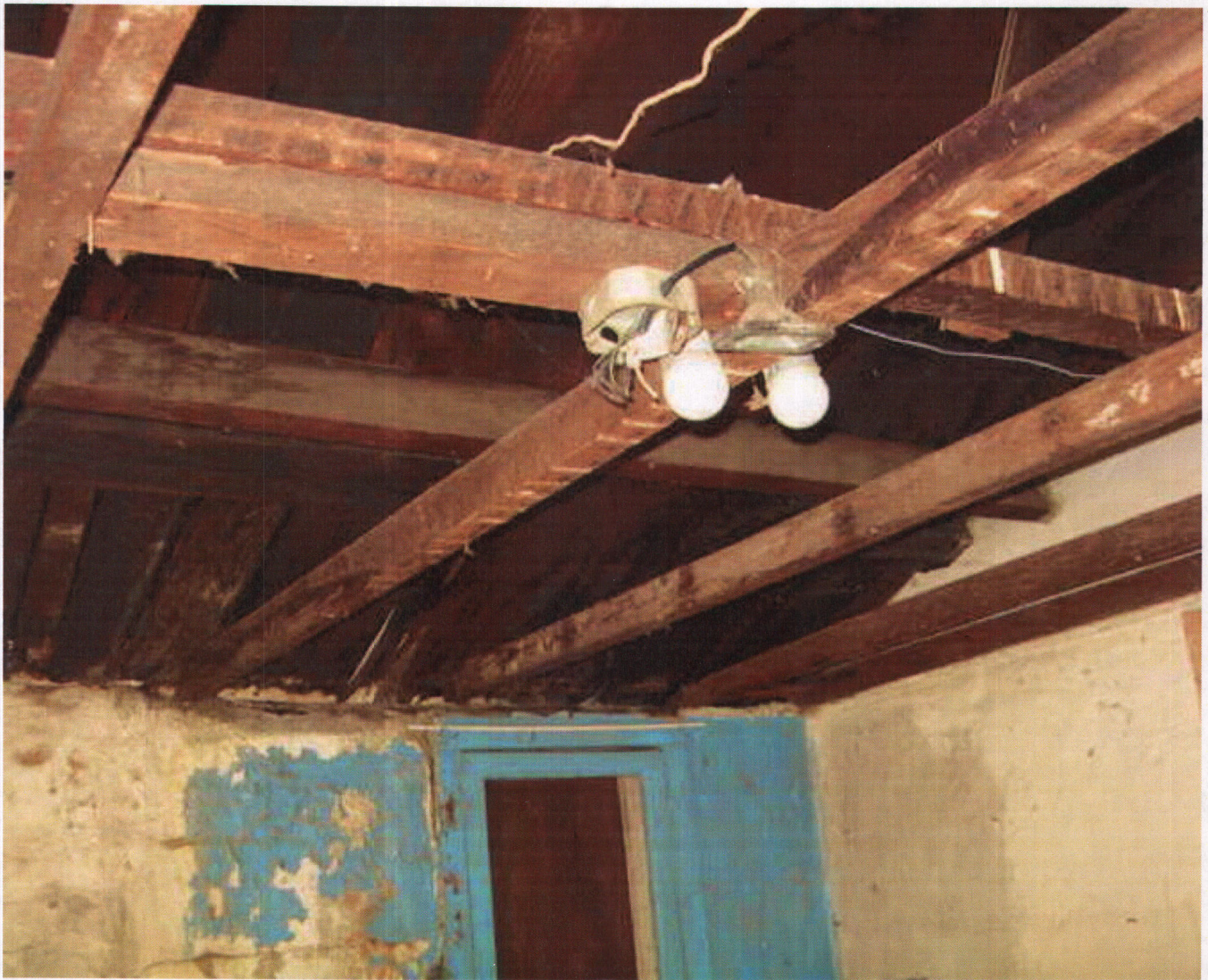
NO LIGHTING & EXPOSED WIRING. DEFECT #5 & 6 - 12/29/2009
