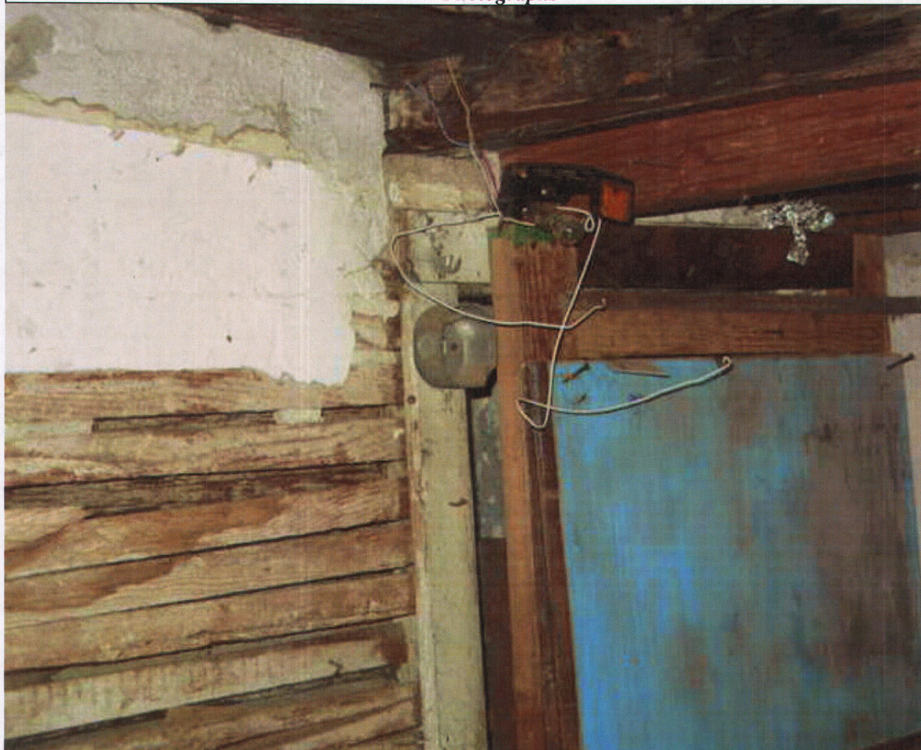
NO LIGHTING INSIDE HOUSE. DEFECT #6 - 12/29/2009
