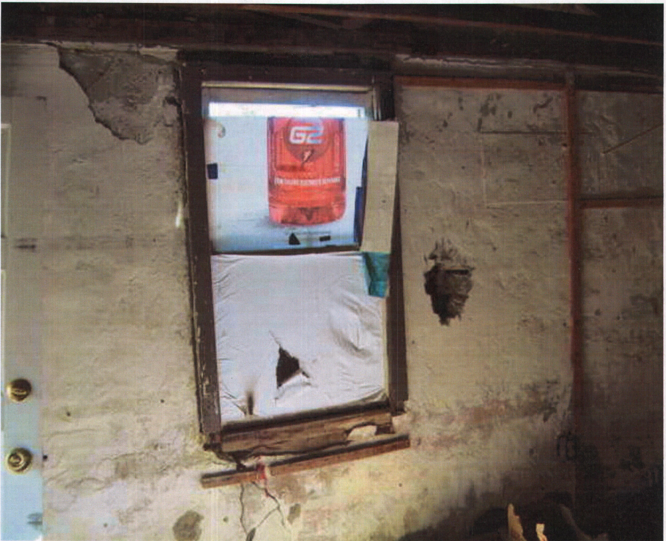
HOLE IN WALL. DEFECT #10 - 12/29/2009
