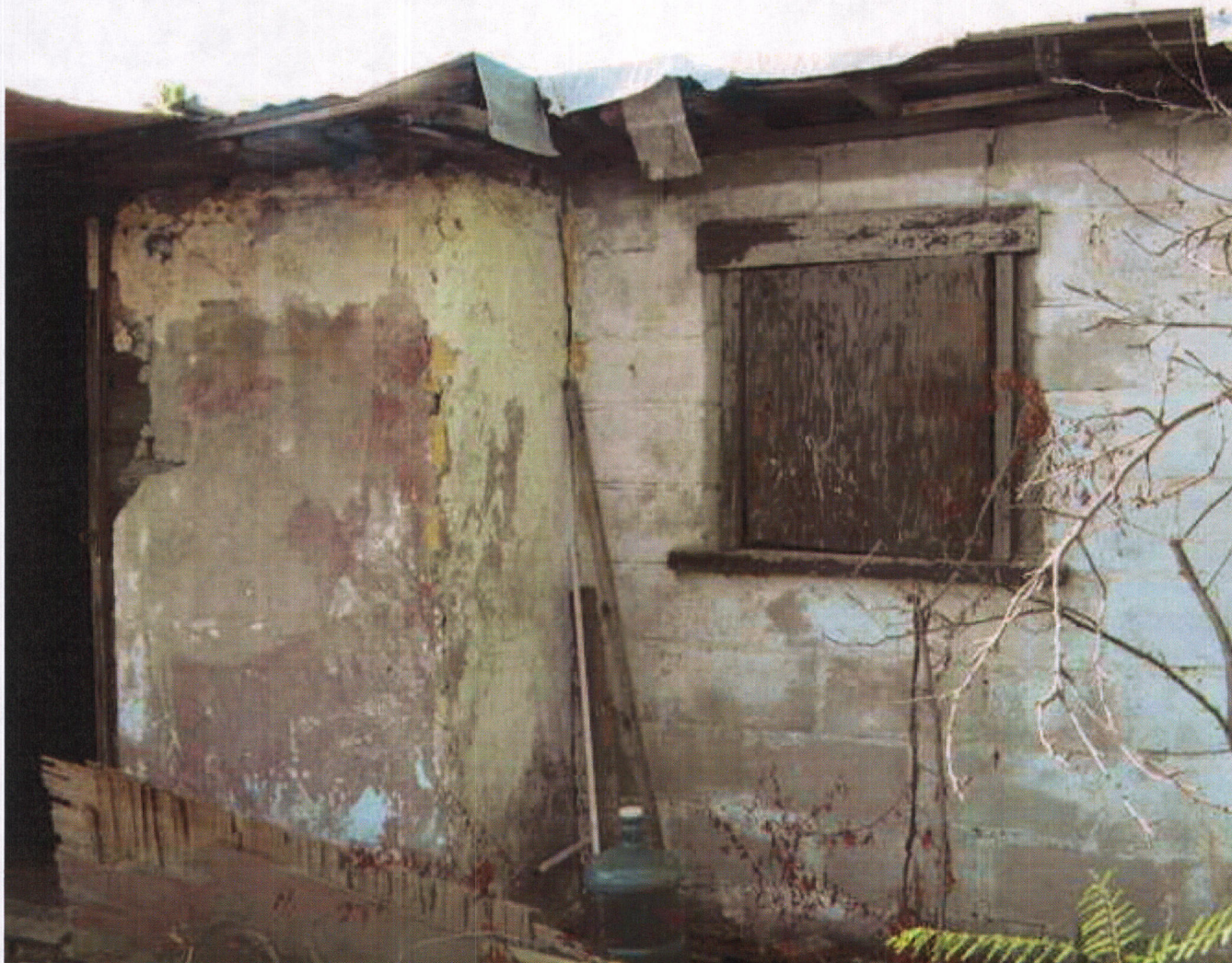
REAR OF HOUSE. DEFECT#14 - 12/29/2009
