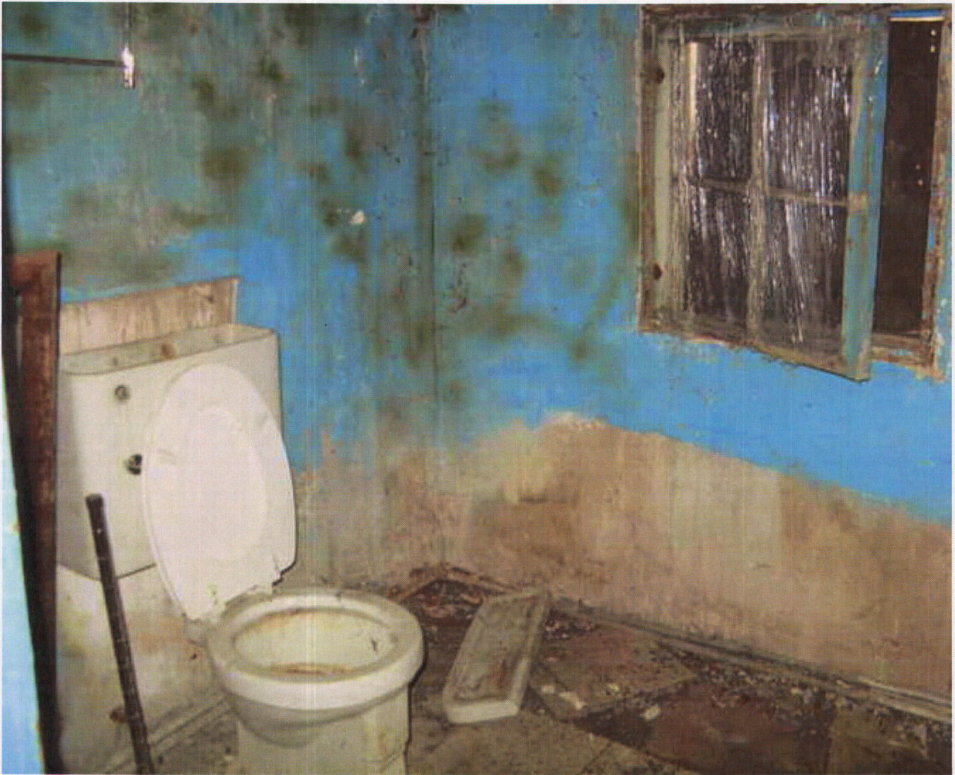
DAMAGED WALLS. DEFECT#14 - 12/29/2009
