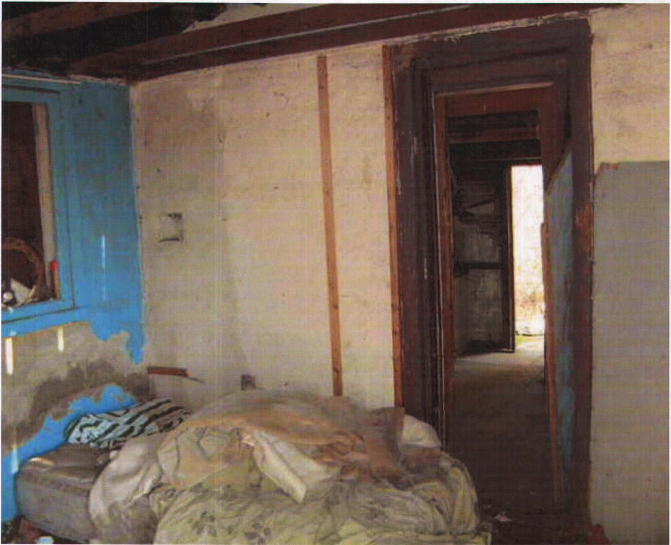
INSIDE OF HOUSE WITH MATTRESS ON GROUND. DEFECT #17 - 12/29/2009
