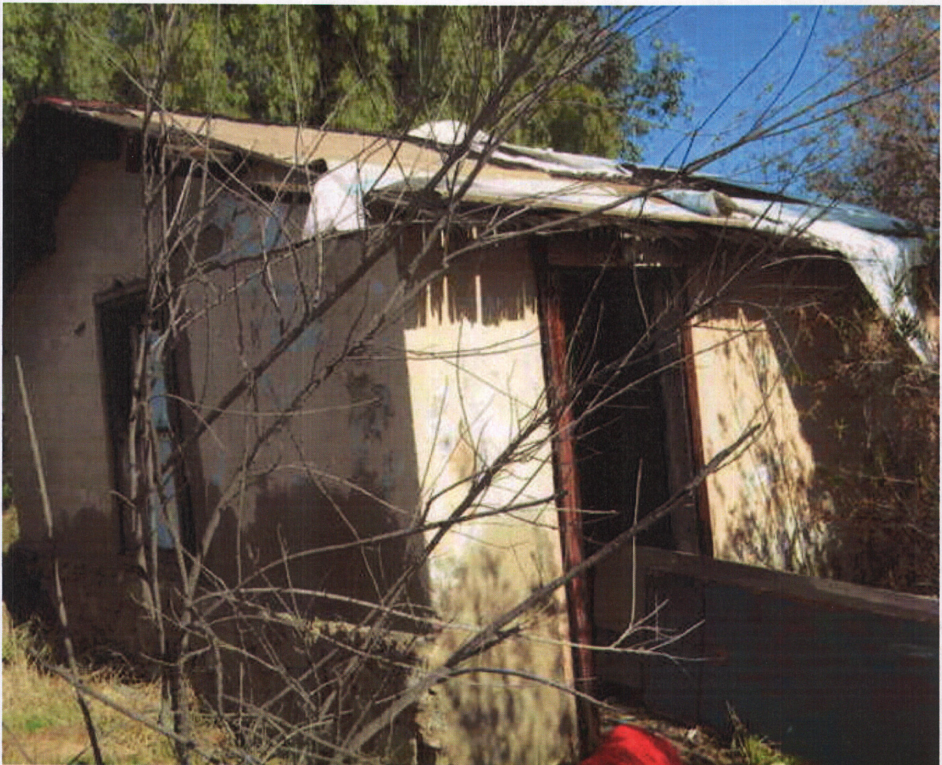
DETERIORATED ROOF. DEFECT #11 - 12/29/2009
