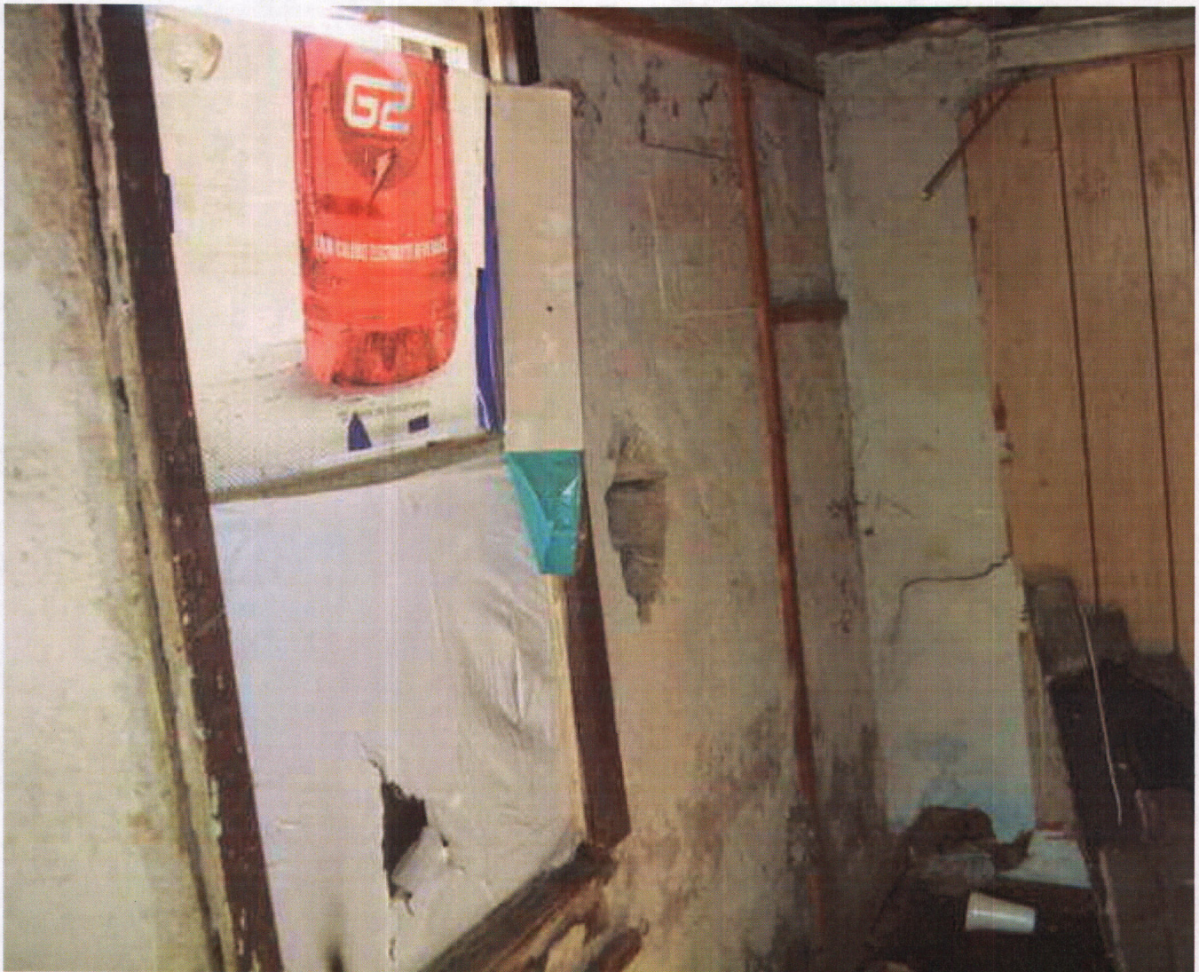
NO HEAT INSIDE HOUSE. DEFECT #7 R ARRIOLA. - 12/29/2009
