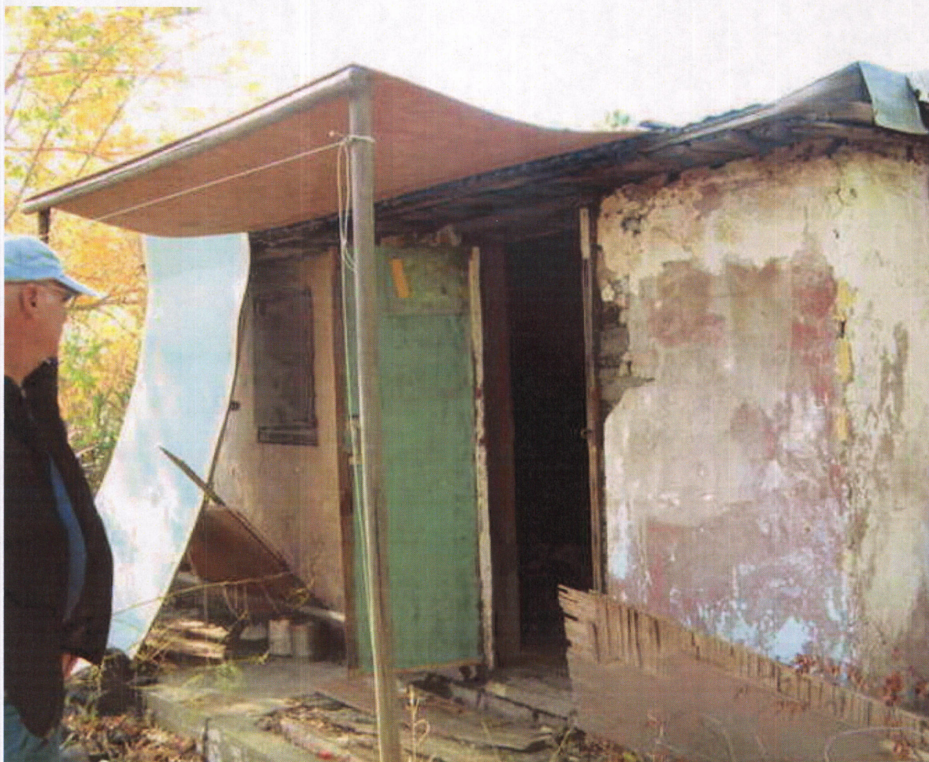
REAR DOOR NOT SECURED. DEFECT #13 & 14 - 12/29/2009
