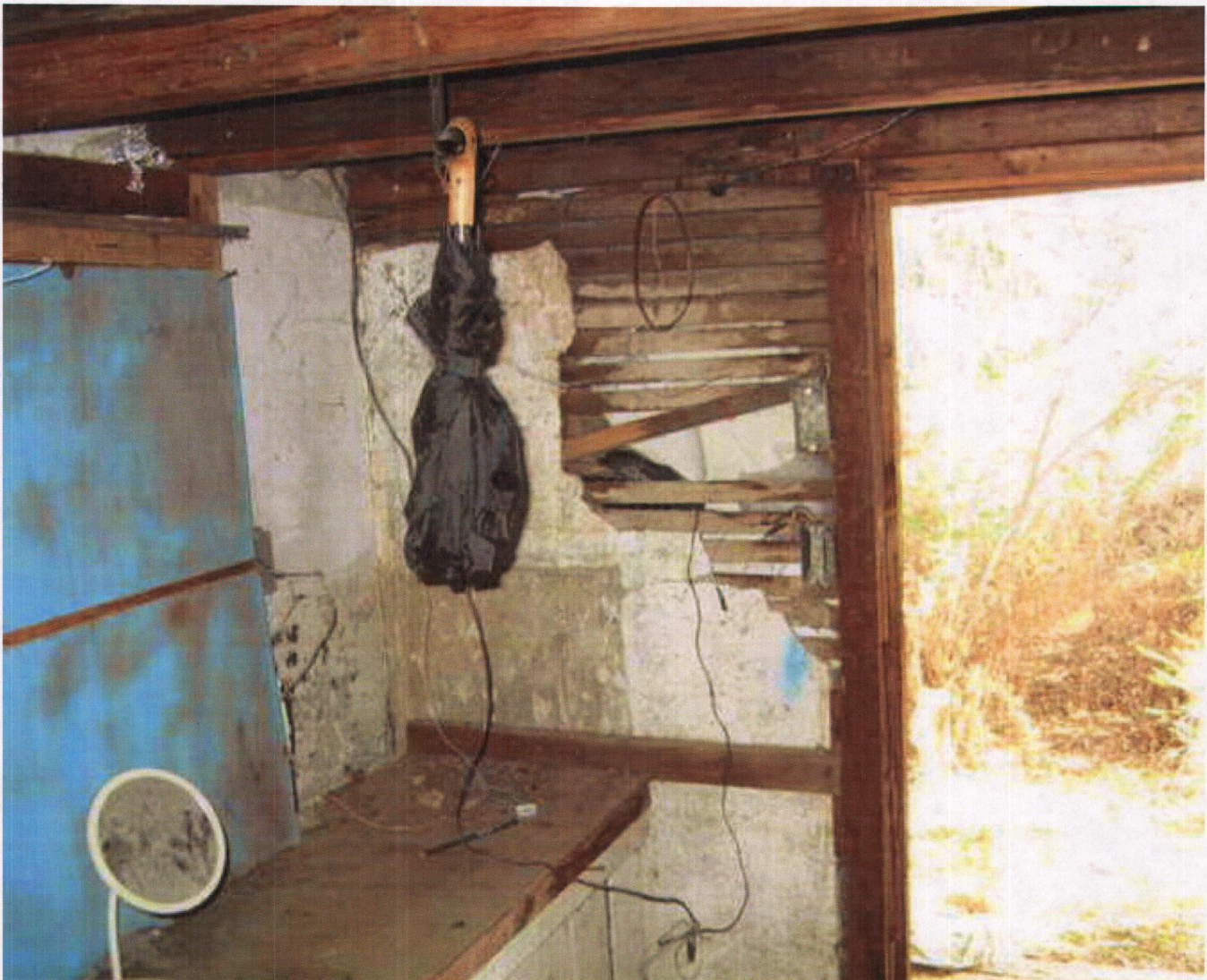
HOUSE OPEN TO THE ELEMENTS AND DETERIORATED WALL. DEFECT #10 & 13 - 12/29/
