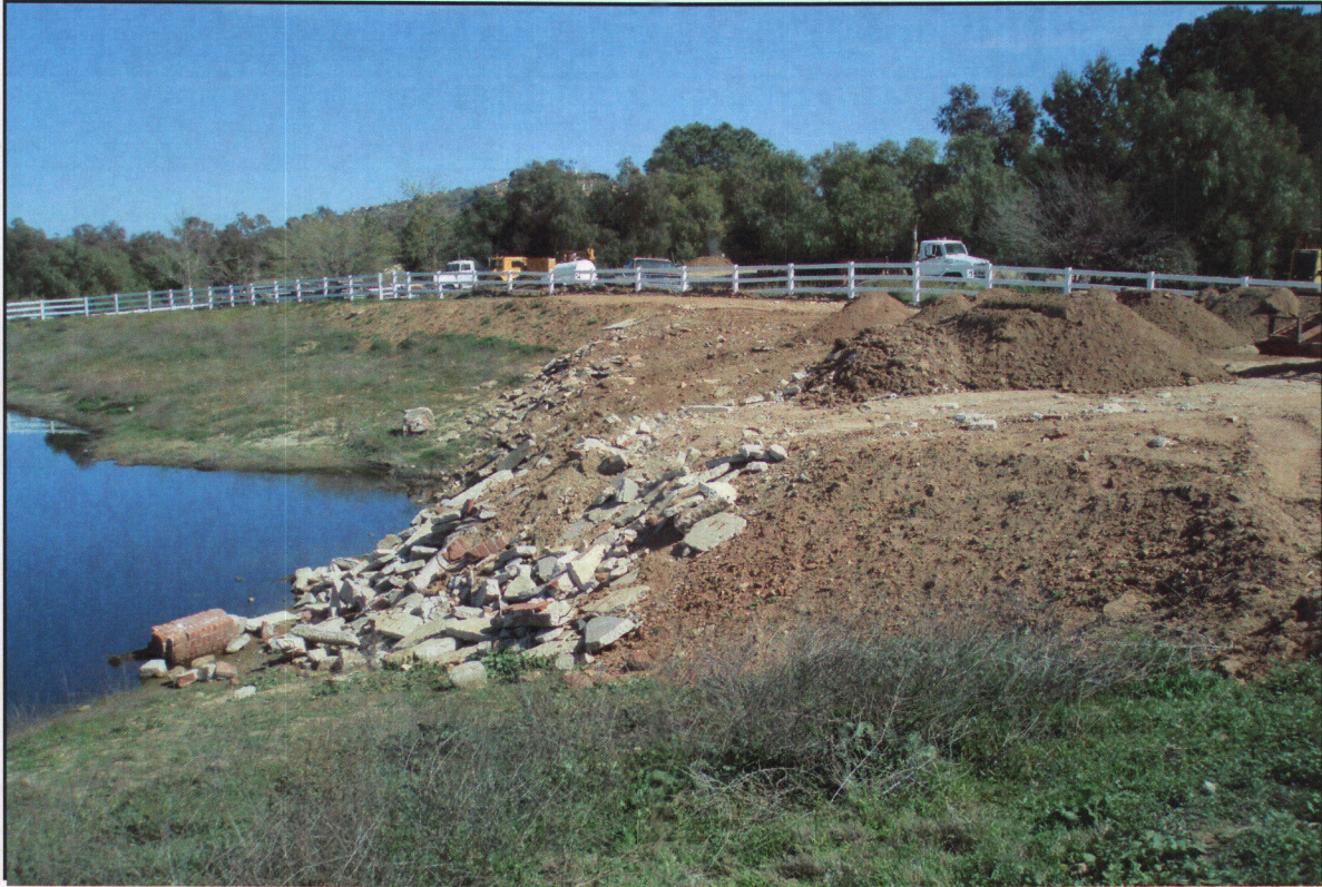
PHOTO # 3 DATE: 03/18/09 TIME: 1100 AM TAKEN BY: BF #21
