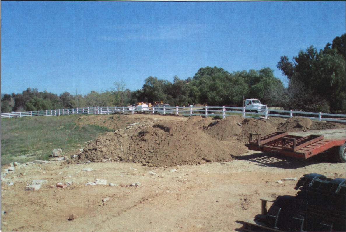
PHOTO # 1 DATE: 3/18/09 TIME: 1100 AM TAKEN BY: BF #21
