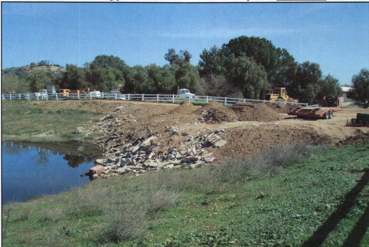
PHOTO # 4 DATE: 03/18/09 TIME: 1100 AM TAKEN BY: BF #21
