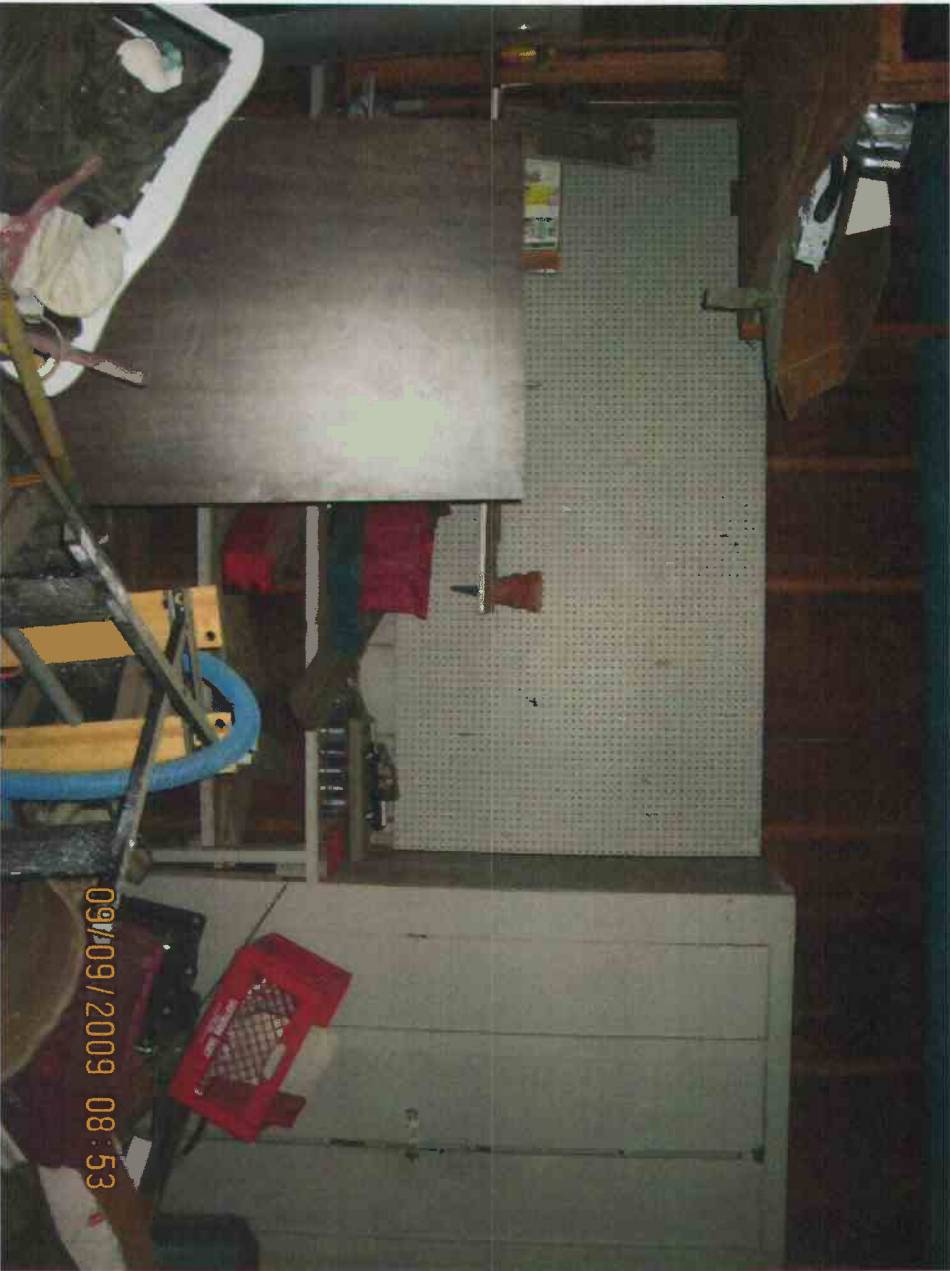
14. General dilapidation or improper maintenance: interior filled with rubbish
