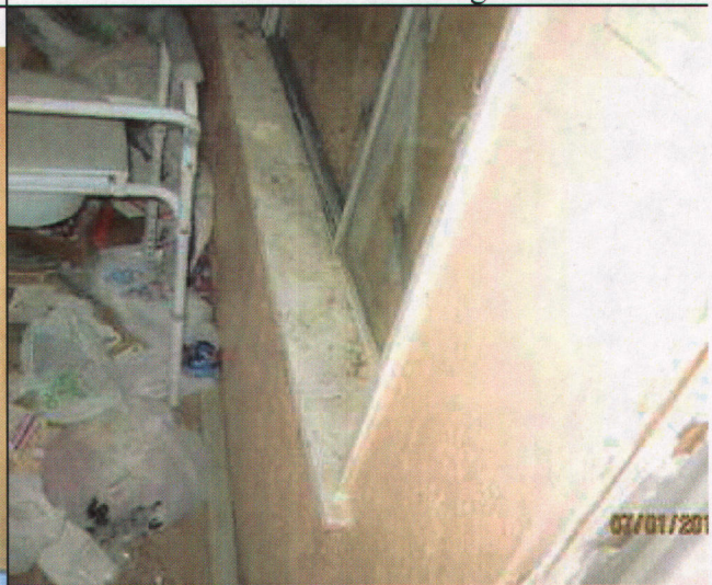
M Sanders 070110 - broken windows and water damage
