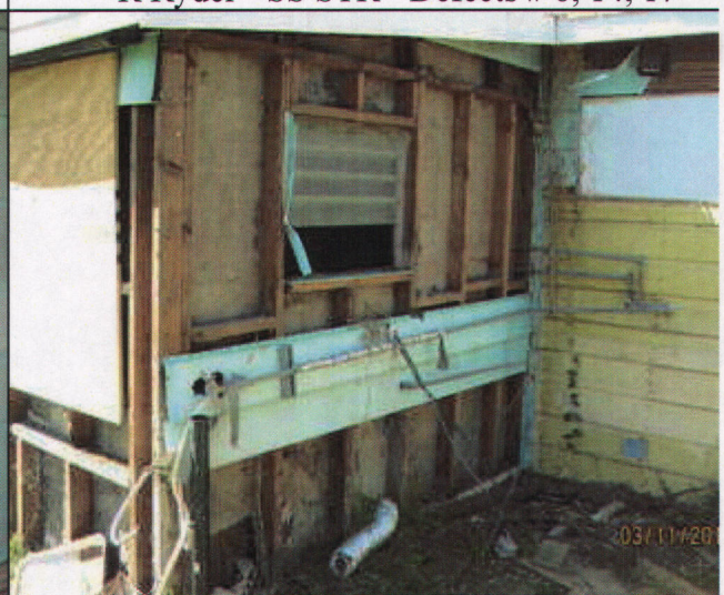
R Ryder - SS STR - Defects # 10, 13, 14, 17
