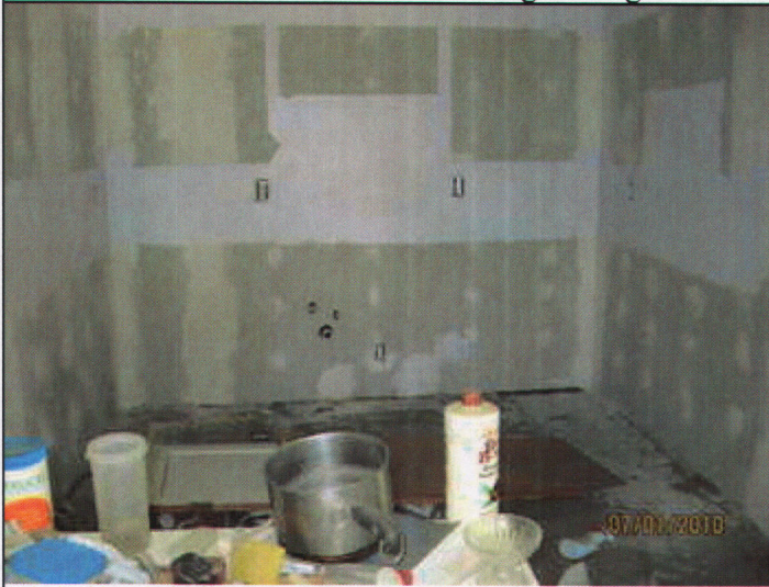
M Sanders 070110 - missing kitchen sink and lighting fixture
