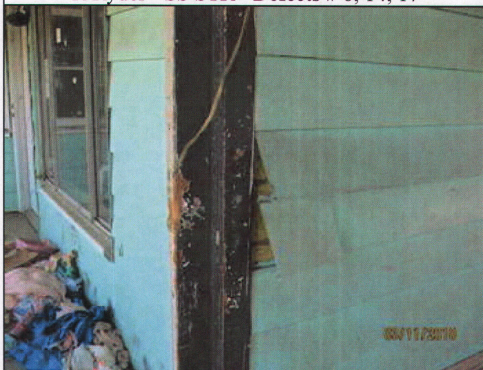
R Ryder - SS STR - Defects # 10, 14, 17
