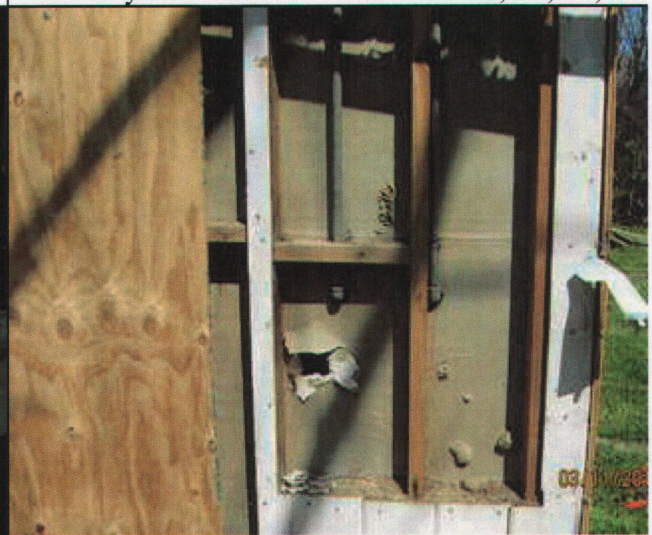
R Ryder - SS STR - Defects # 10, 12, 13, 14, 17
