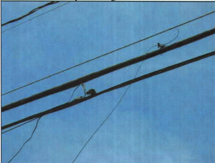
Powerline dropping. KR
