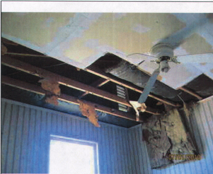
M Sanders 070110 - missing ceiling
