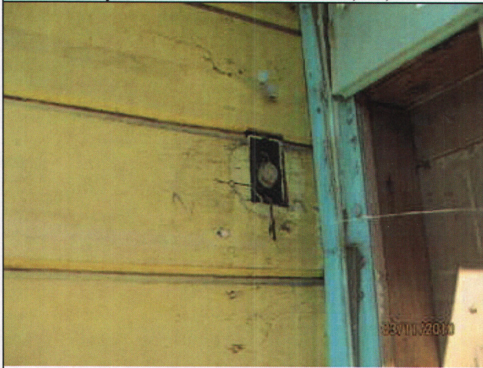
R Ryder - SS STR - Defects # 6, 14, 17
