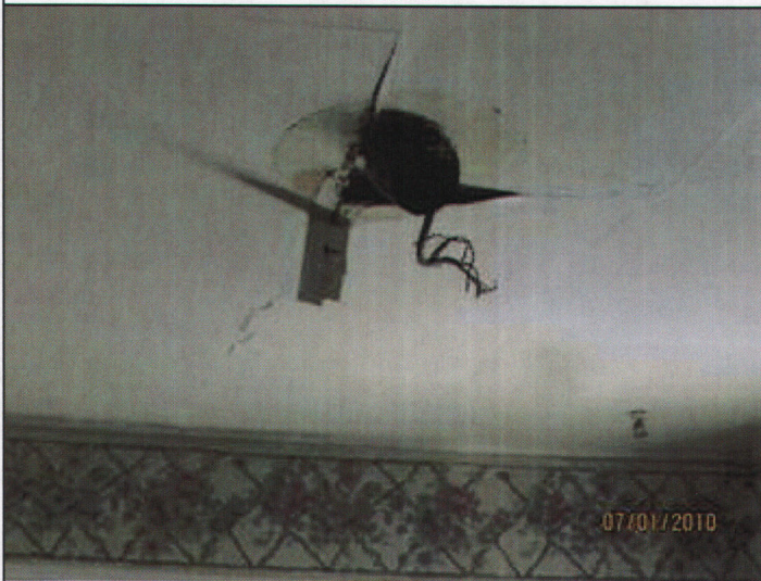
M Sanders 070110 - missing lighting fixture and exposed electrical wiring
