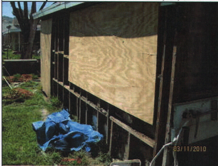
R Ryder - SS STR - Defects # 10, 13, 14, 17
