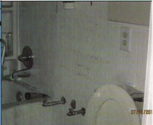
M Sanders 070110 - missing bathroom sink
