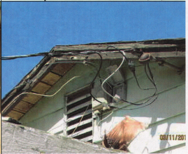
R Ryder - SS STR - Defects # 6, 14, 17
