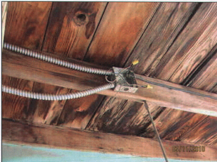
R Ryder - SS STR - Defects # 6, 14, 17
