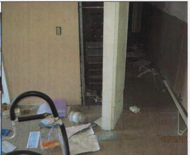
M Sanders 070110 - heater, thermostat missing fi wall
