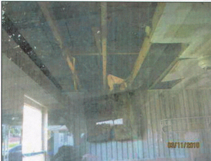
R Ryder - SS STR - Defects # 11, 12, 14, 17
