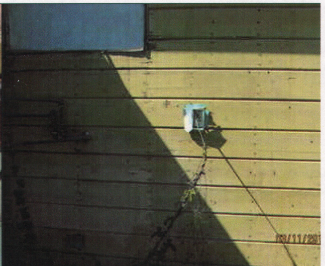
R Ryder - SS STR - Defects # 6, 14, 17
