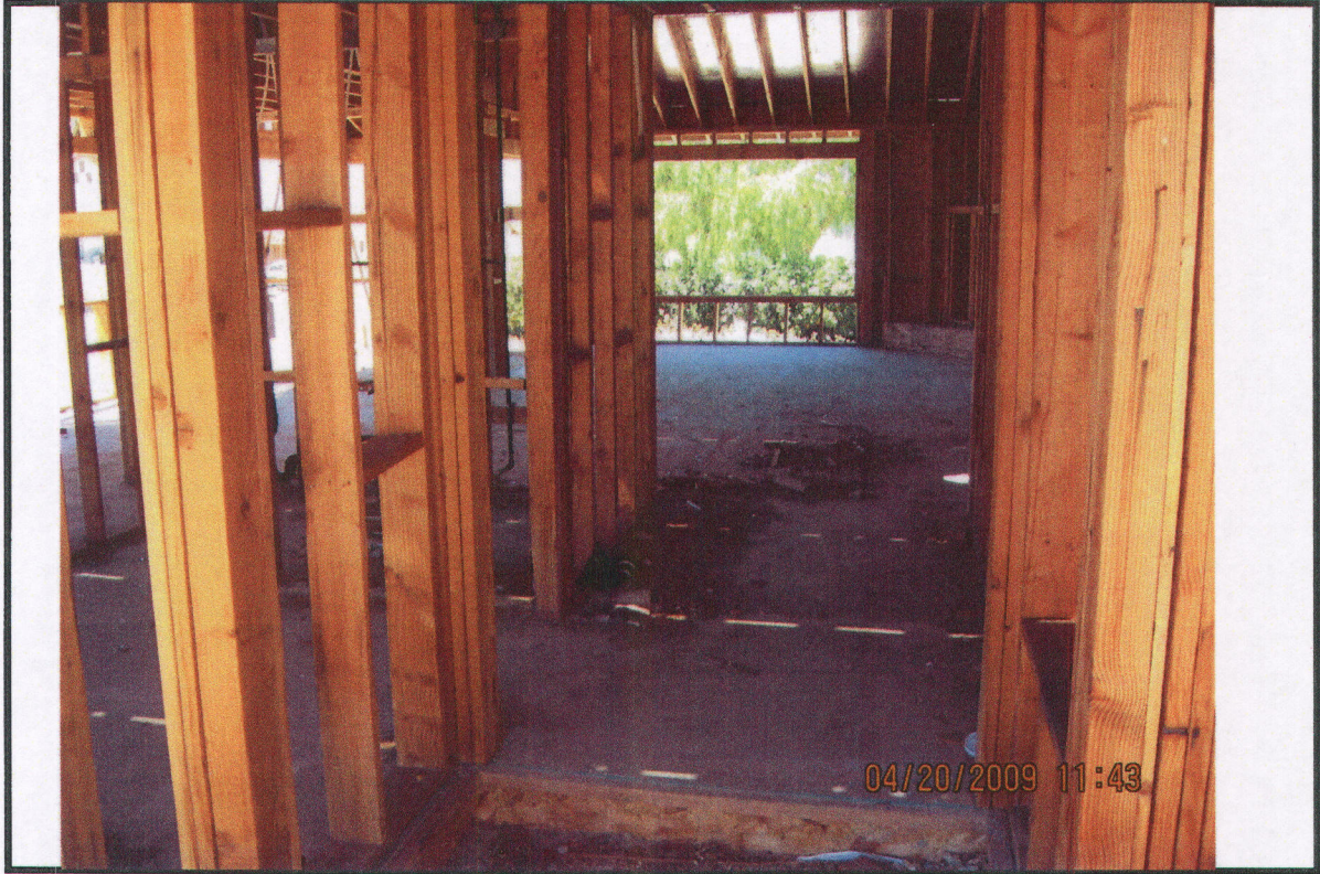
PHOTO # 3 DATE: 04/20/09 TAKEN BY: J. Pike #59 NOTES: Debris collecting inside Notice of Defect # 12, 13, 17, 19
