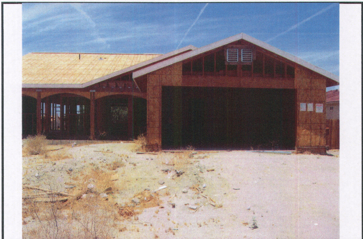
PHOTO # 2 DATE: 06/11/09 TAKEN BY: J. Pike #59 NOTES: Notice of Defect # 12, 13, 17, 19
