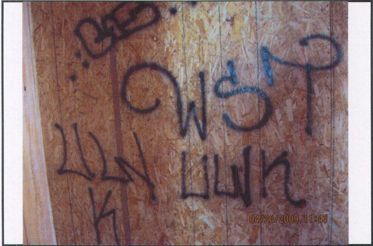
PHOTO # 5 DATE: 04/20/09 TAKEN BY: J. Pike #59 NOTES: Graffiti Notice of Defect # 17
