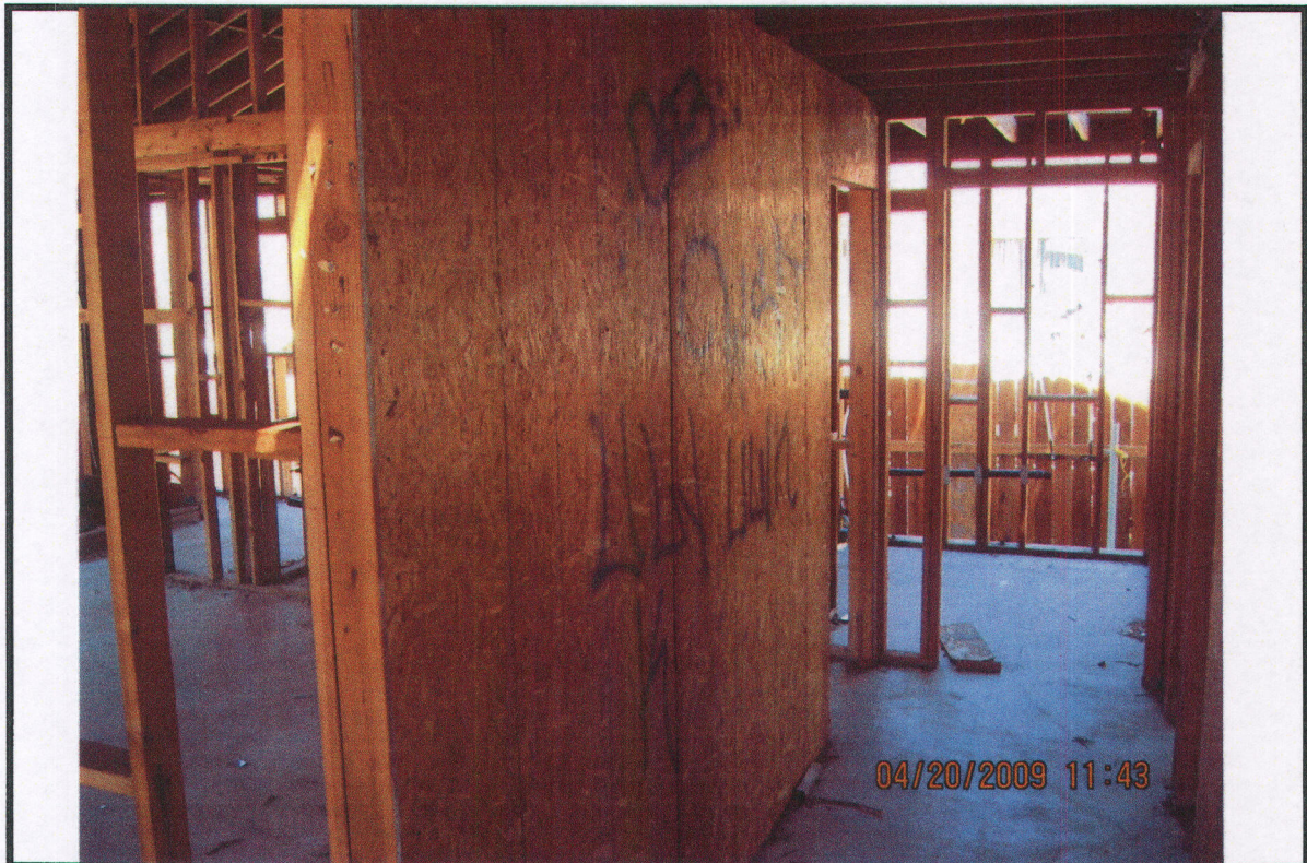
PHOTO # 4 DATE: 04/20/09 TAKEN BY: J. Pike #59 NOTES: Graffiti Notice of Defect # 12, 13, 17, 19
