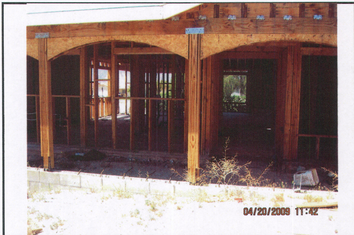
PHOTO # 2 DATE: 04/20/09 TAKEN BY: J. Pike #59 NOTES: No walls Notice of Defect # 12, 13, 17, 19
