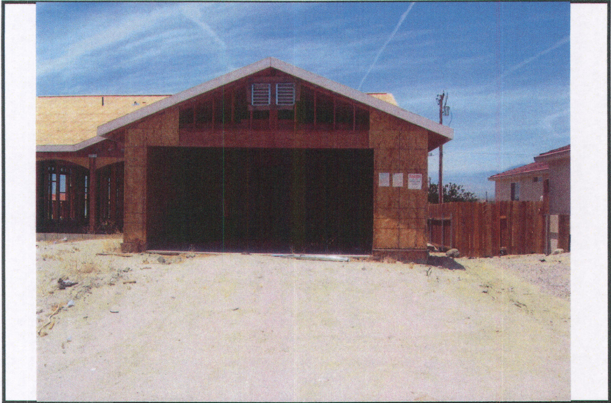
PHOTO # 1 DATE: 06/11/09 TAKEN BY: J. Pike #59 NOTES: Property remains in Violation Notice of Defect # 12, 13, 17, 19
