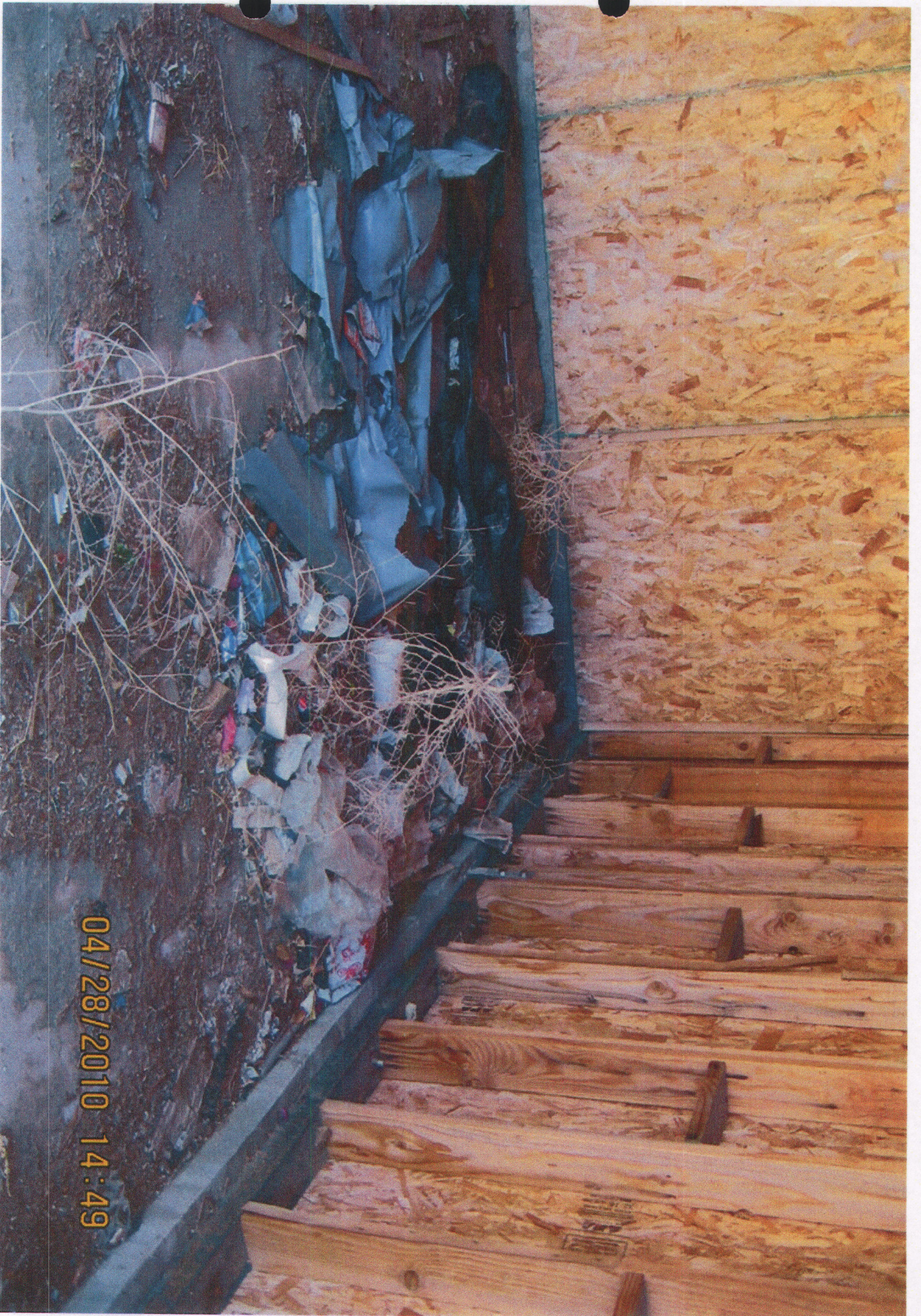
CV0807411, Herrera, Rubbish inside the structure
