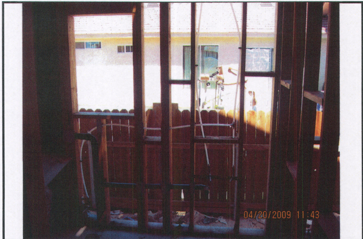
PHOTO # 6 DATE: 04/20/09 TAKEN BY: J. Pike #59 NOTES: Exposed plumbing Notice of Defect # 12, 13, 17, 19
