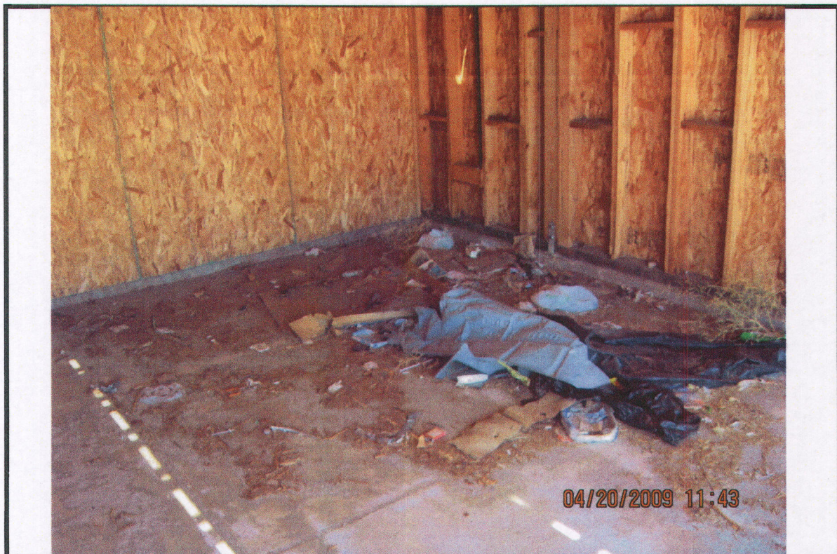
PHOTO # 8 DATE: 04/20/09 TAKEN BY: J. Pike #59 NOTES: Trash Notice of Defect # 17
