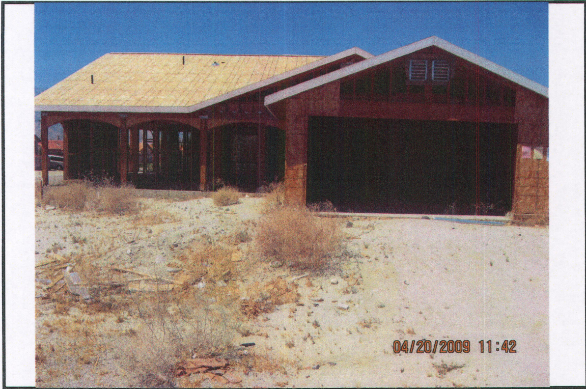
PHOTO # 1 DATE: 04/20/09 TAKEN BY: J. Pike #59 NOTES: Residence Unfinished Notice of Defect # 12, 13, 17, 19
