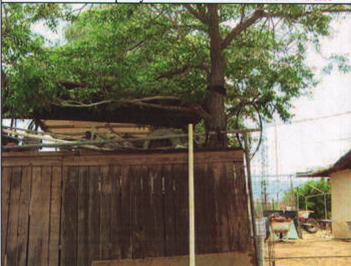
05/13/10 - Property Remains in Violation – Pike
