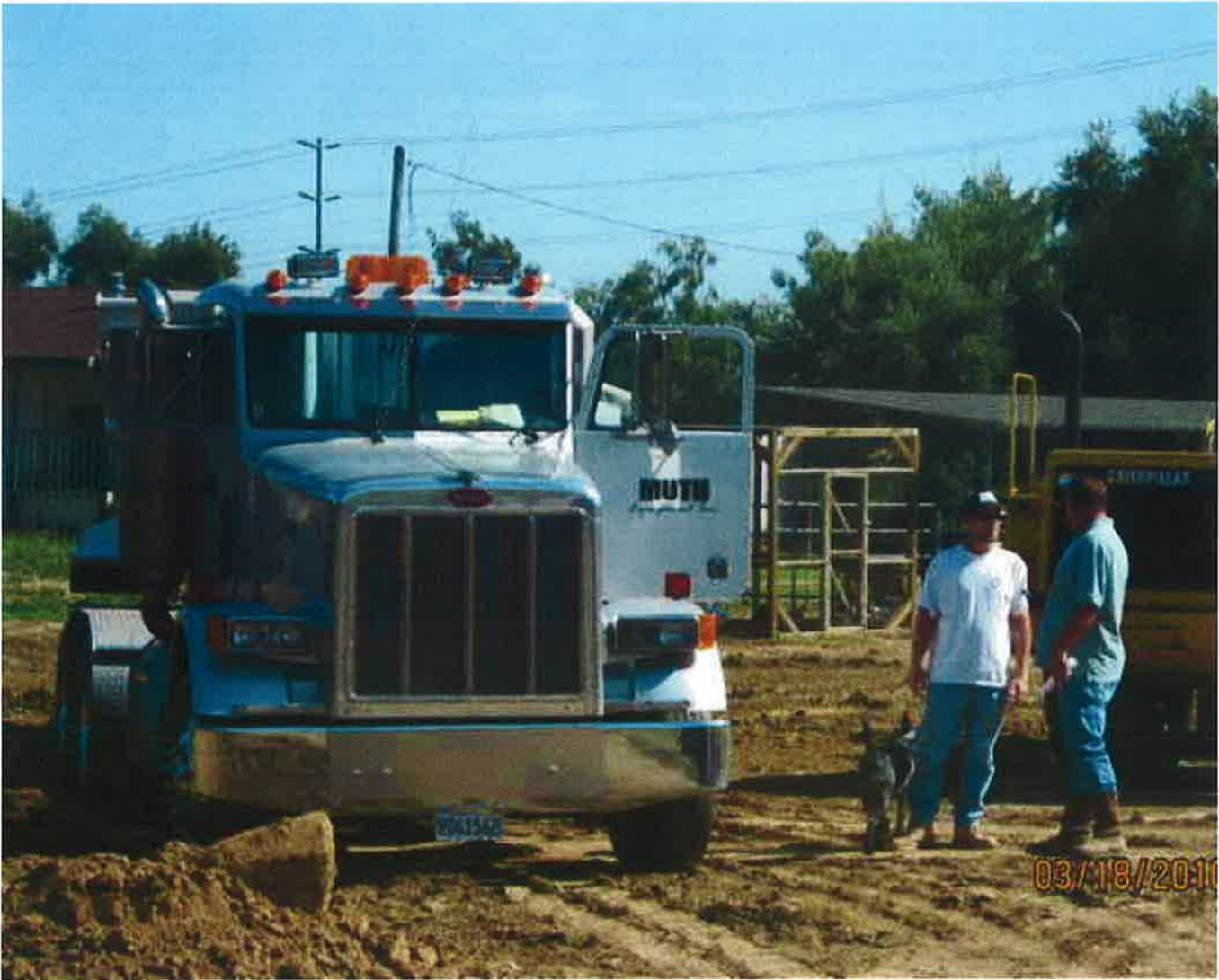
Another load of dirt to be dumped. PO informing driver to remove. J Chamberlain - 03/18/2010
