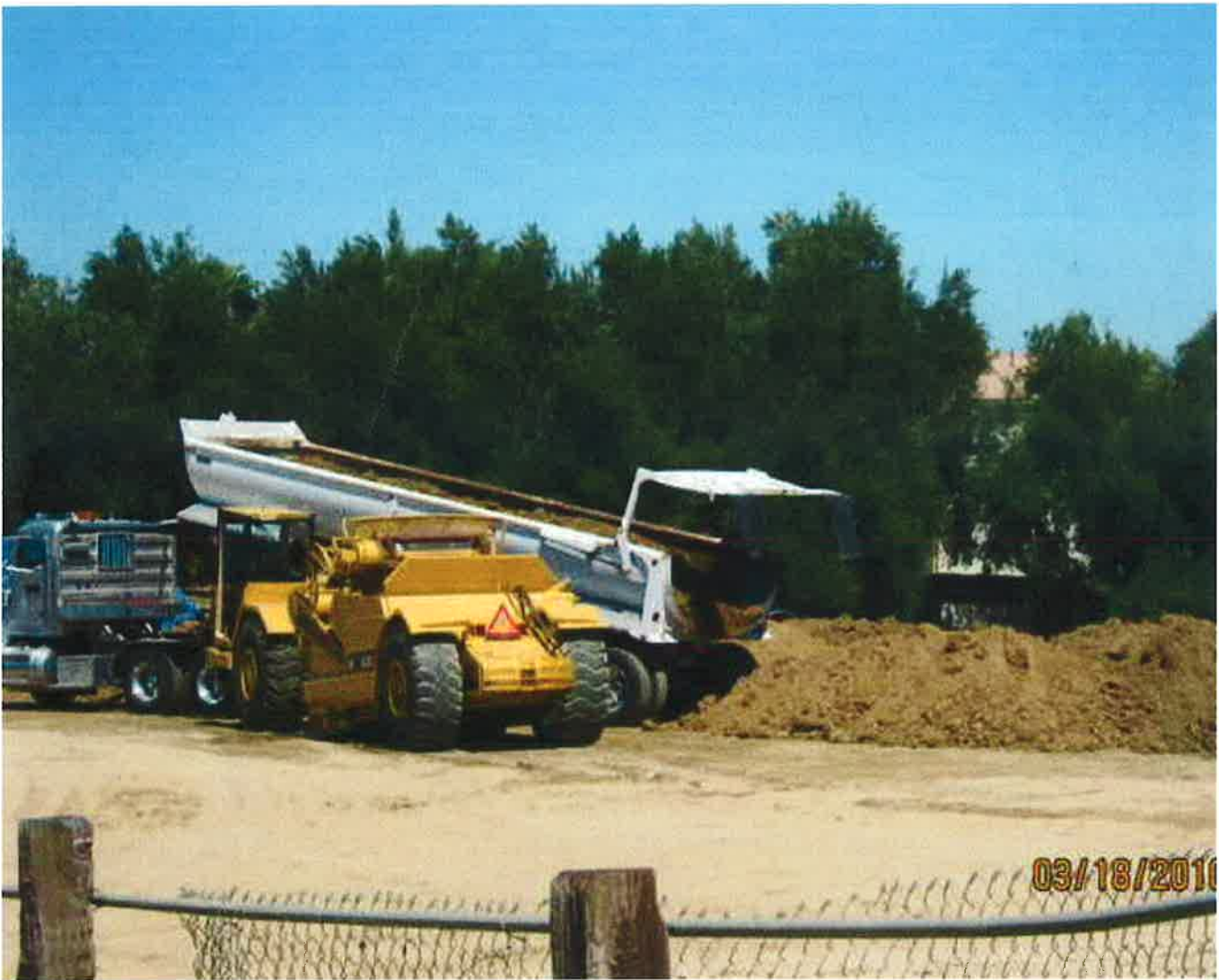
Dirt being dumped on property. J Chamberlain - 03/18/2010
