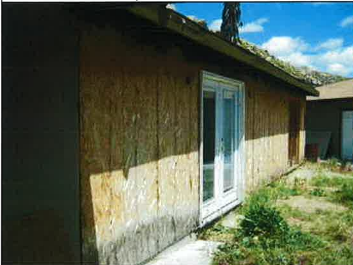
Condition 14; General dilapidation. KR
