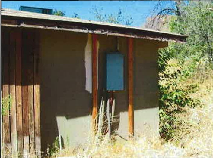
M Sanders 091610 - lack of paint & unprotected wiring
