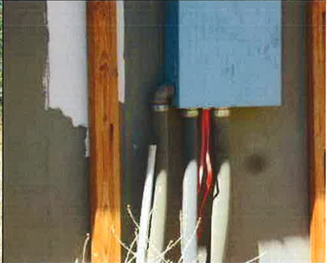
M Sanders 091610 - close up of the unprotecte wiring
