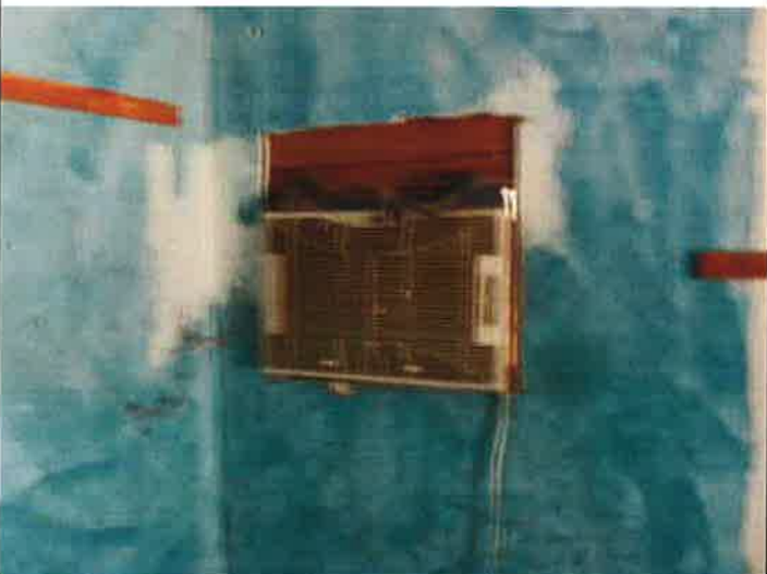
M Sanders 091610 - improper wall mounted swamp
