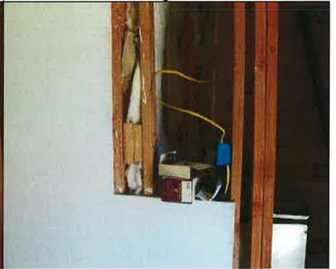
M Sanders 091610 -interior walls not finished unprotected wiring, no permits for renovation
