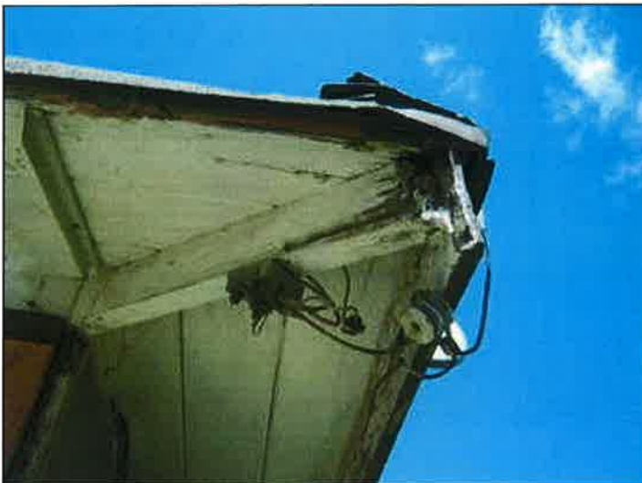
Condition 11; Deterioration of roof. KR
