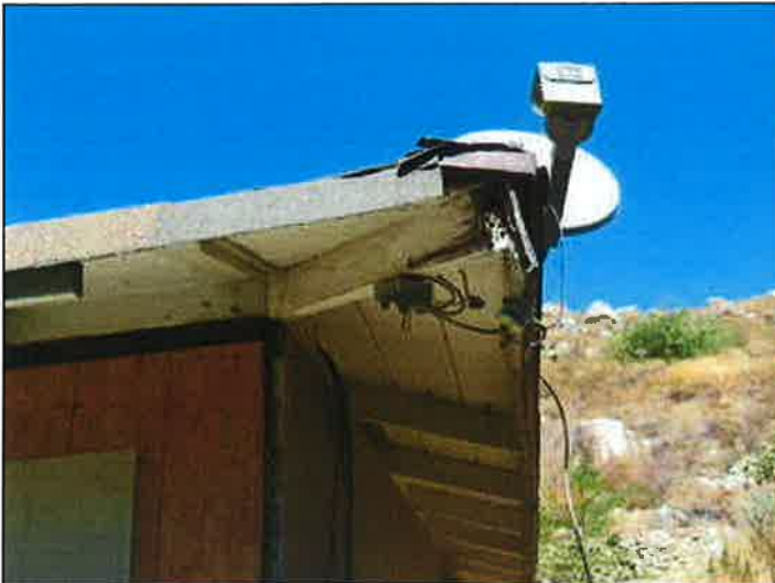
M Sanders 091610 - rotted eave, improper maintenance
