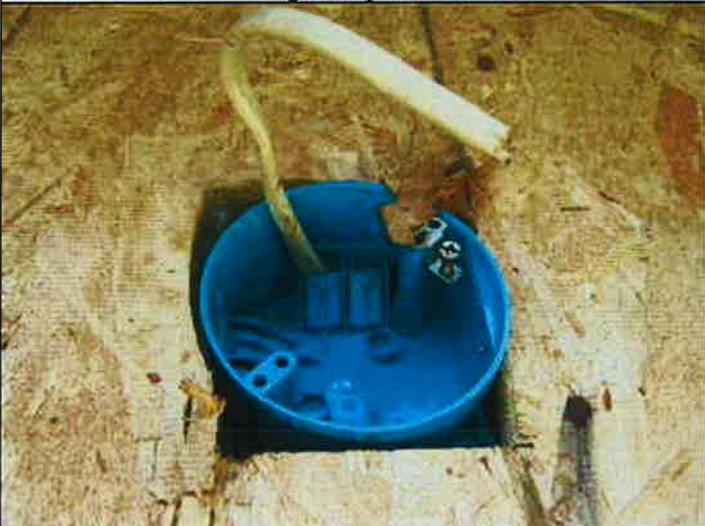
Condition 5; Lack of required electrical lighting. KR
