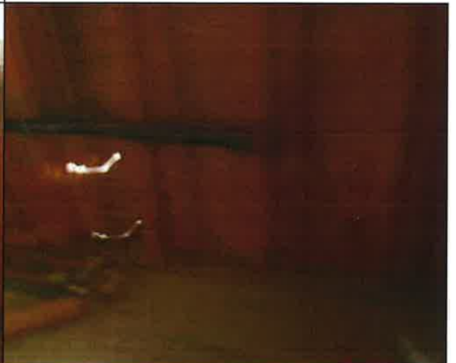
M Sanders 091610 -incompletd work, unknown drain and supply line
