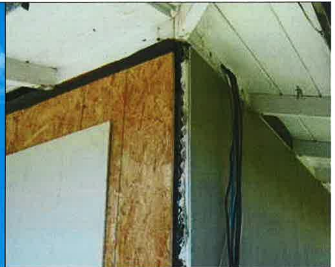
Condition 13; Faulty weather protection. KR
