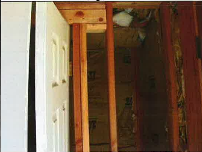
M Sanders 091610 - interior walls not finished, no permits for renovation
