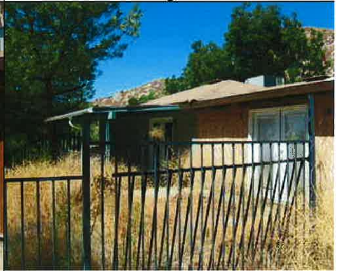
M Sanders 091610 -unfinished exterior wall, exposed wiring, west side
