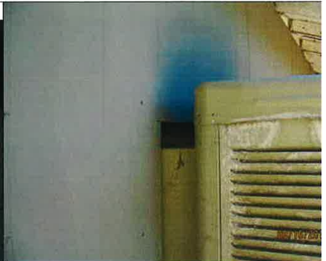
M Sanders 091610 - gap in wall between swann cooler, faulty weather protection
