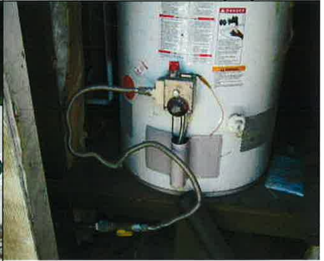
Condition 4; Hazardous plumbing. KR
