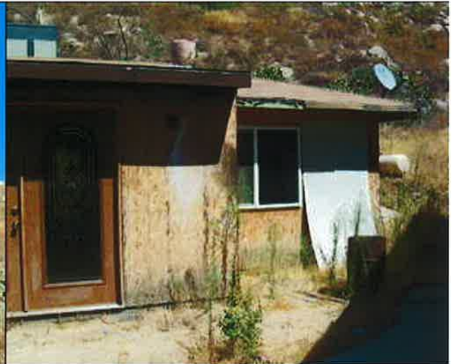
M Sanders 091610 - unfinished exterior wall, exposed wiring, east side
