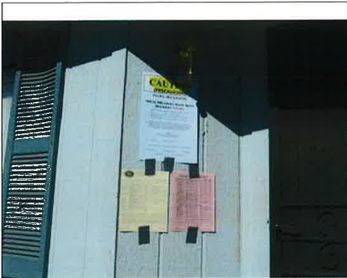
NOV, NOD & CAUTION sign posted on 04/28/2010.
