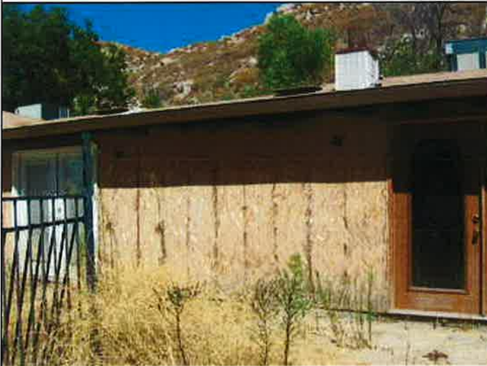
M Sanders 091610 -unfinished exterior wall, exposed wiring, center
