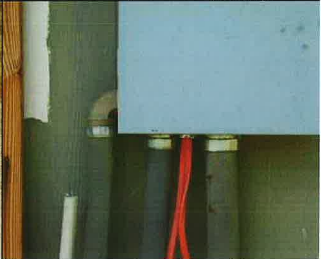
Condition 6; Hazardous wiring. KR
