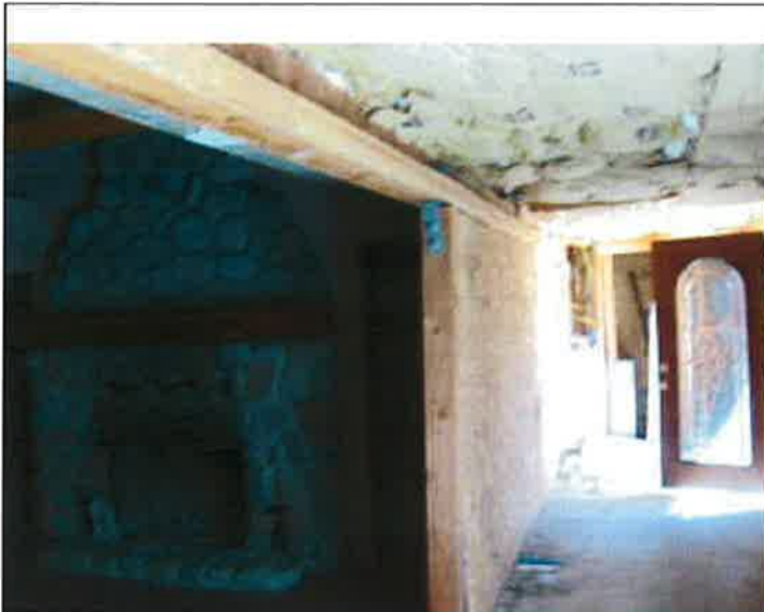
M Sanders 091610 -interior walls / ceiling not finished & no permits for renovation
