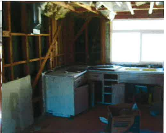
M Sanders 091610 -interior walls / ceiling not finished, lack of plumbing & no permits for renovation
