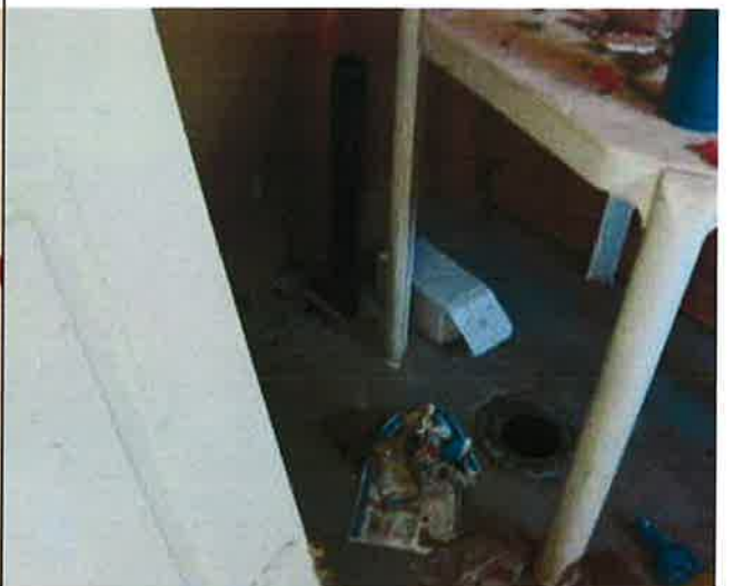
M Sanders 091610 - missing toilet and vent pip
