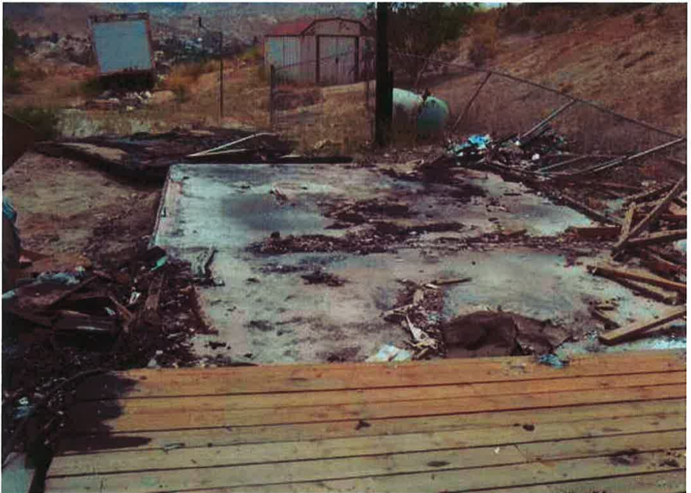
LLyon Remaining wood deck, foundation and burnt debris. - 06/11/2010
