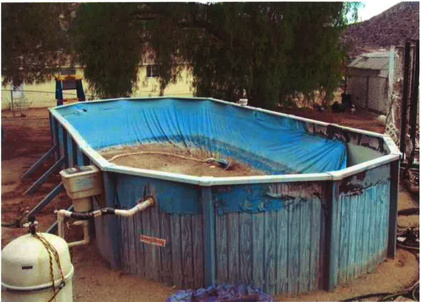
Taken by CEO Lyon - An above ground pool with damage from the fire. - 11/13/2009
