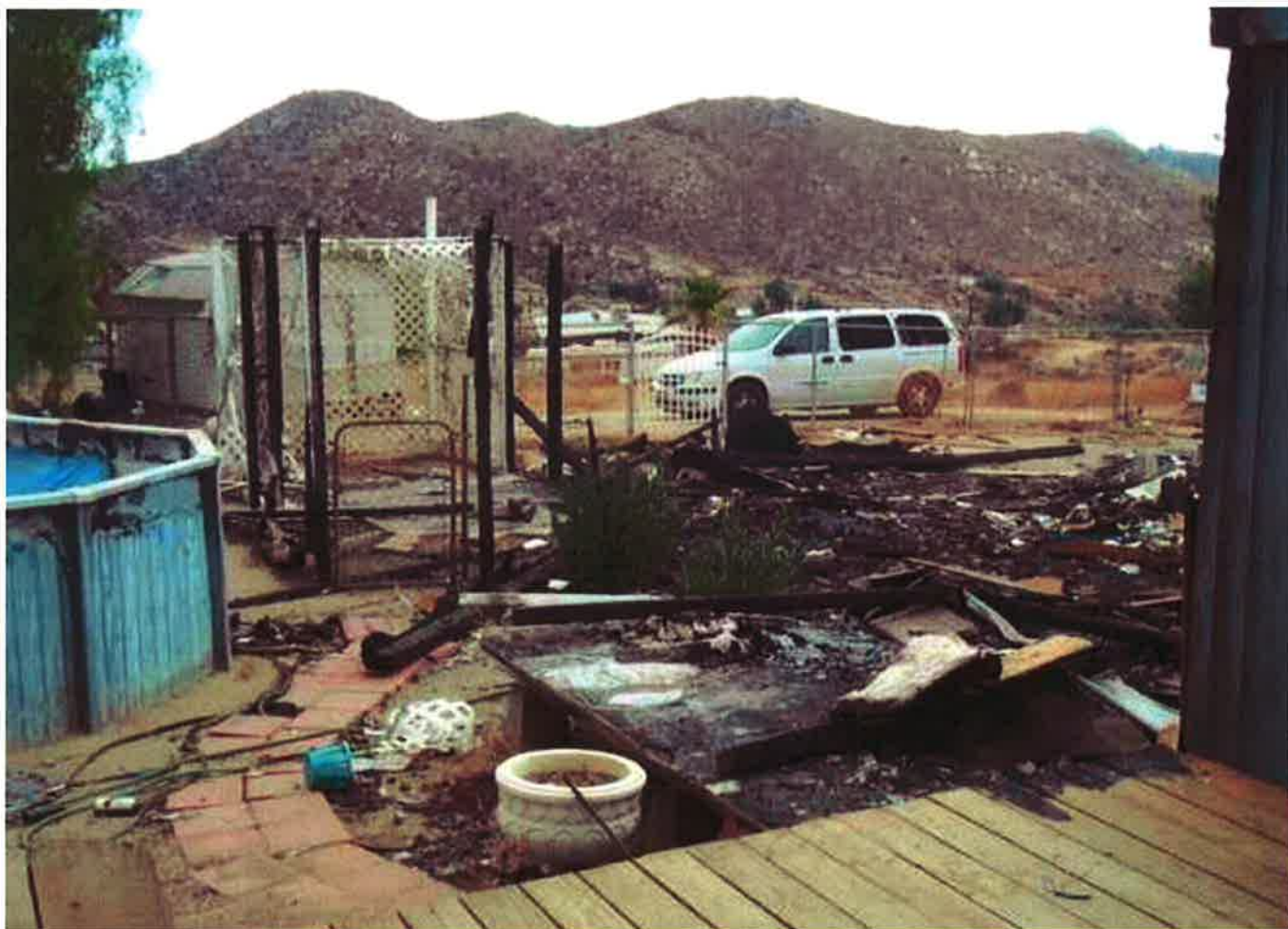
Taken by CEO Lyon - Take from deck on north side of the mobile facing the S/E across the front ya 11/13/2009
