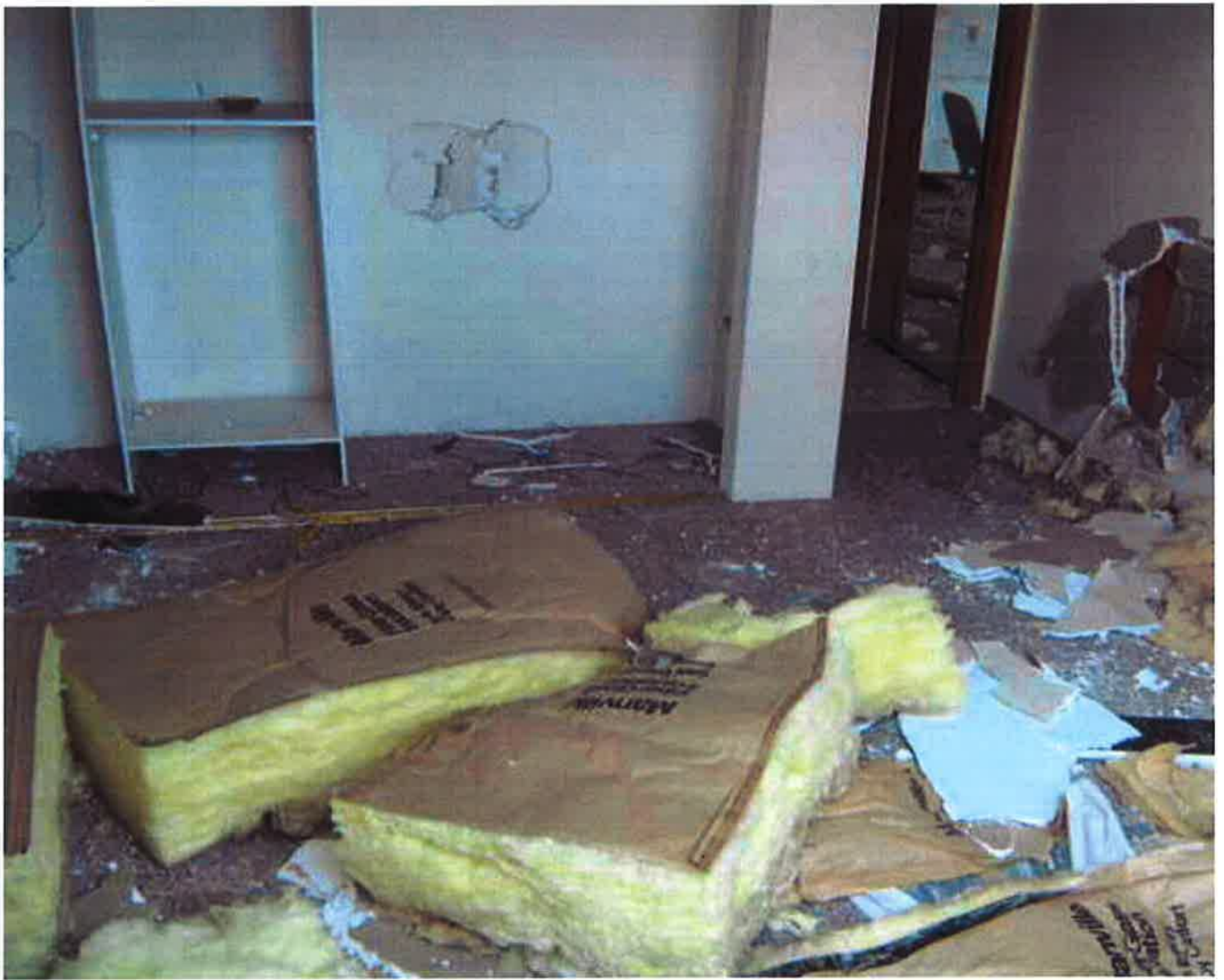
02/05/10 - Substandard Structure NOD# 12 - 02/05/2010
