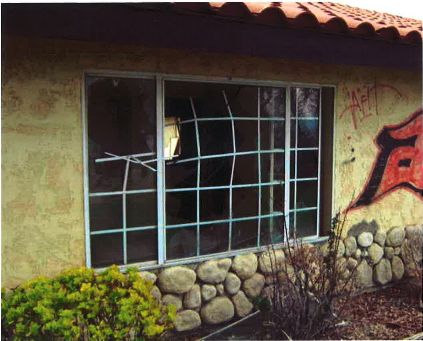
02/05/10 - Substandard Structure NOD# 17 - 02/05/2010
