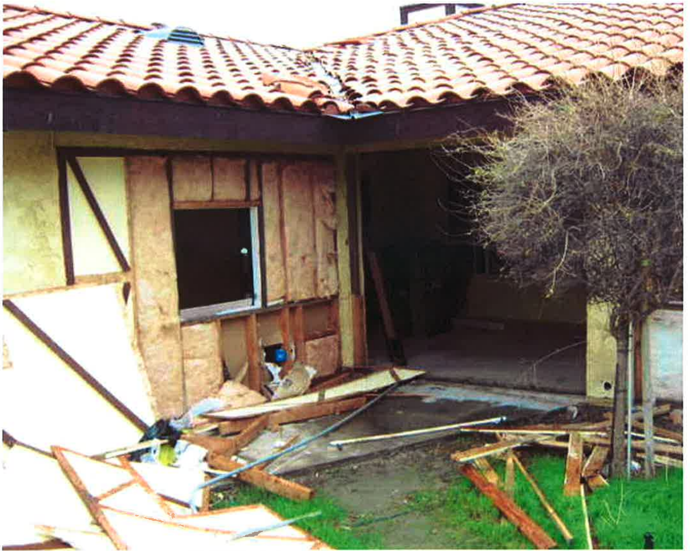
02/05/10 - Substandard Structure NOD# 1 - 02/05/2010
