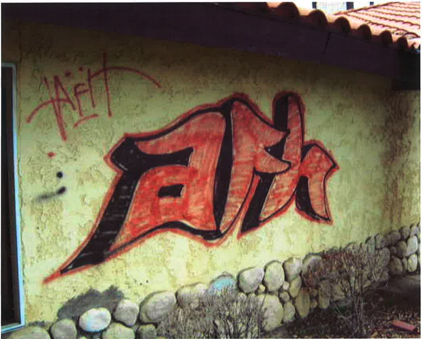
02/05/10 - Substandard Structure NOD# 17 - 02/05/2010
