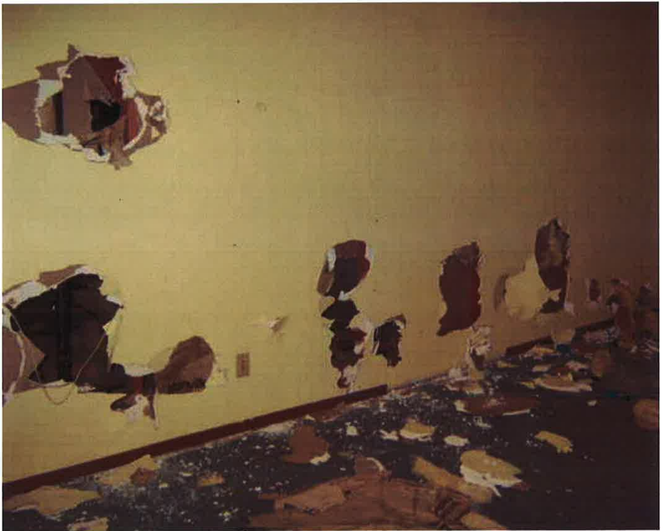
02/05/10 - Substandard Structure NOD# 10 - 02/05/2010
