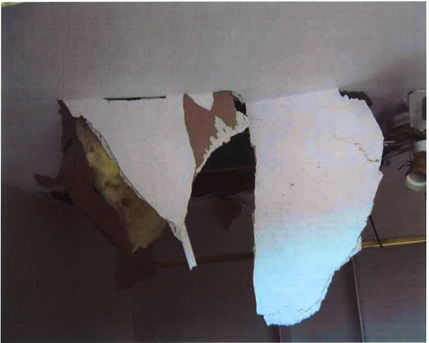
02/05/10 - Substandard Structure NOD# 11 - 02/05/2010
