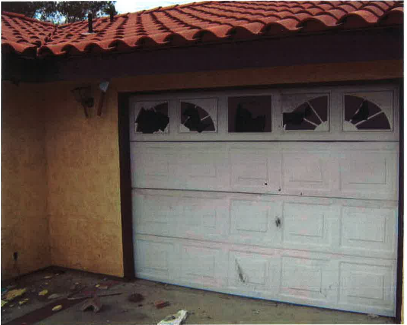
02/05/10 - Substandard Structure NOD# 14 - 02/05/2010
