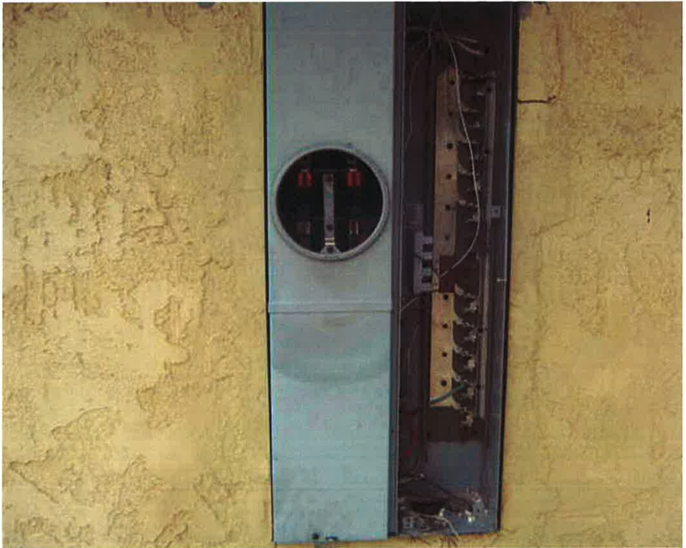
02/05/10 - Substandard Structure NOD# 5 - 02/05/2010
