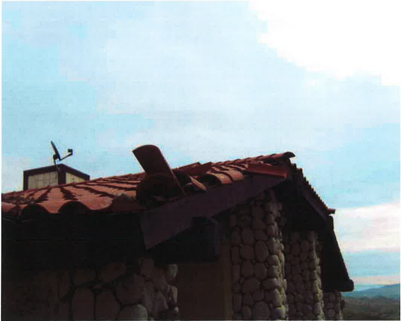
02/05/10 - Substandard Structure NOD# 11 - 02/05/2010
