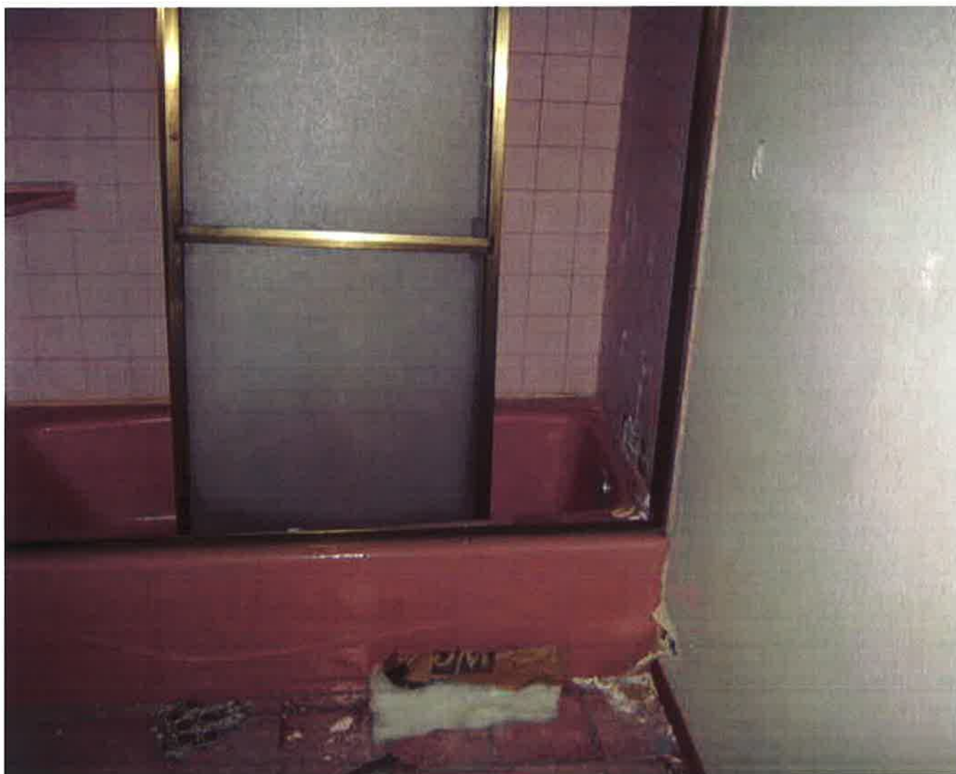
02/05/10 - Substandard Structure NOD# 1 - 02/05/2010
