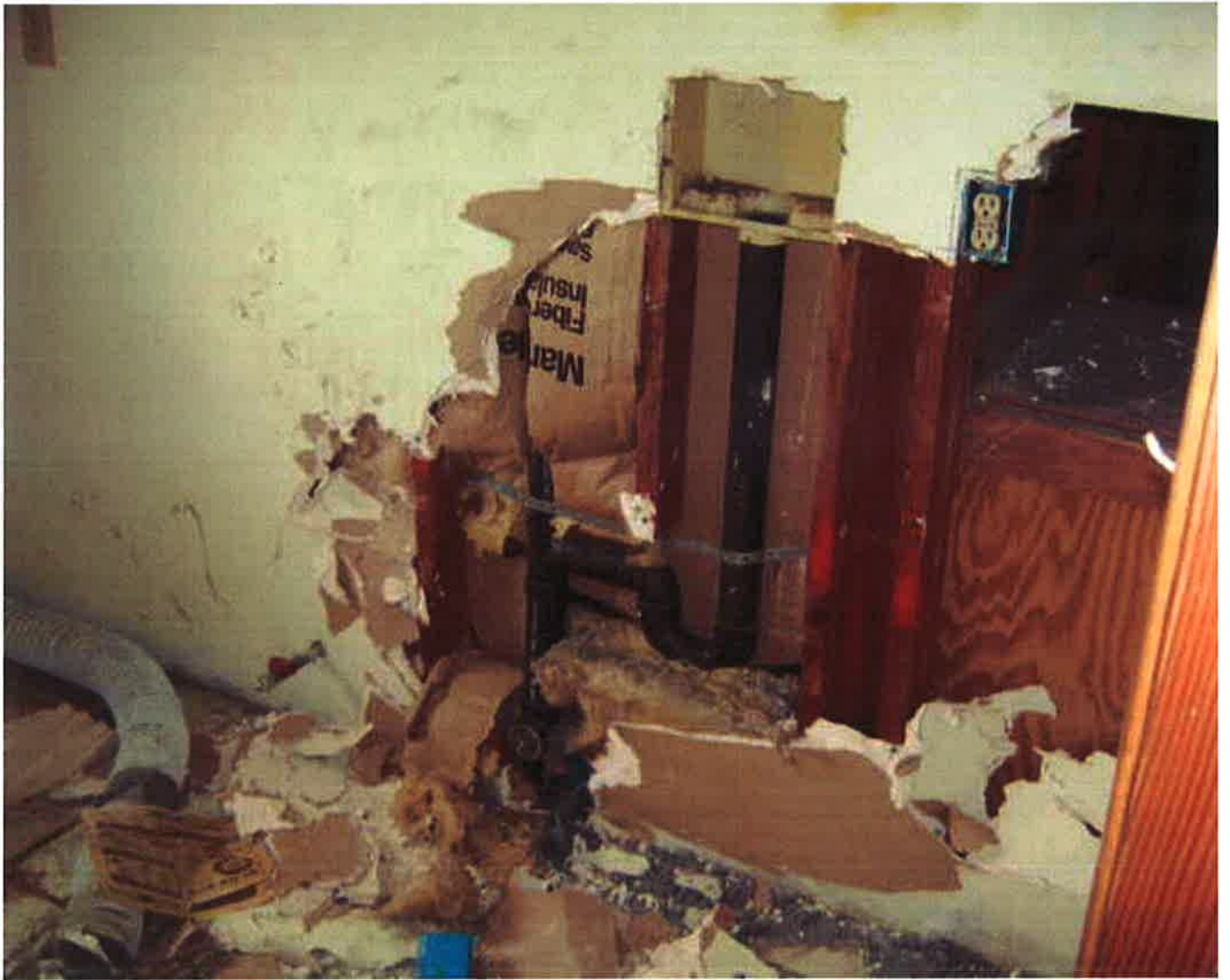
02/05/10 - Substandard Structure NOD# 2 - 02/05/2010
