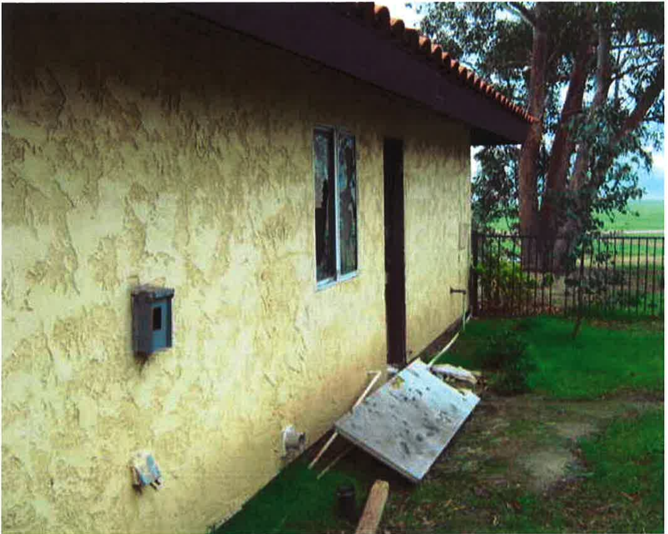
02/05/10 - Substandard Structure NOD# 7 - 02/05/2010
