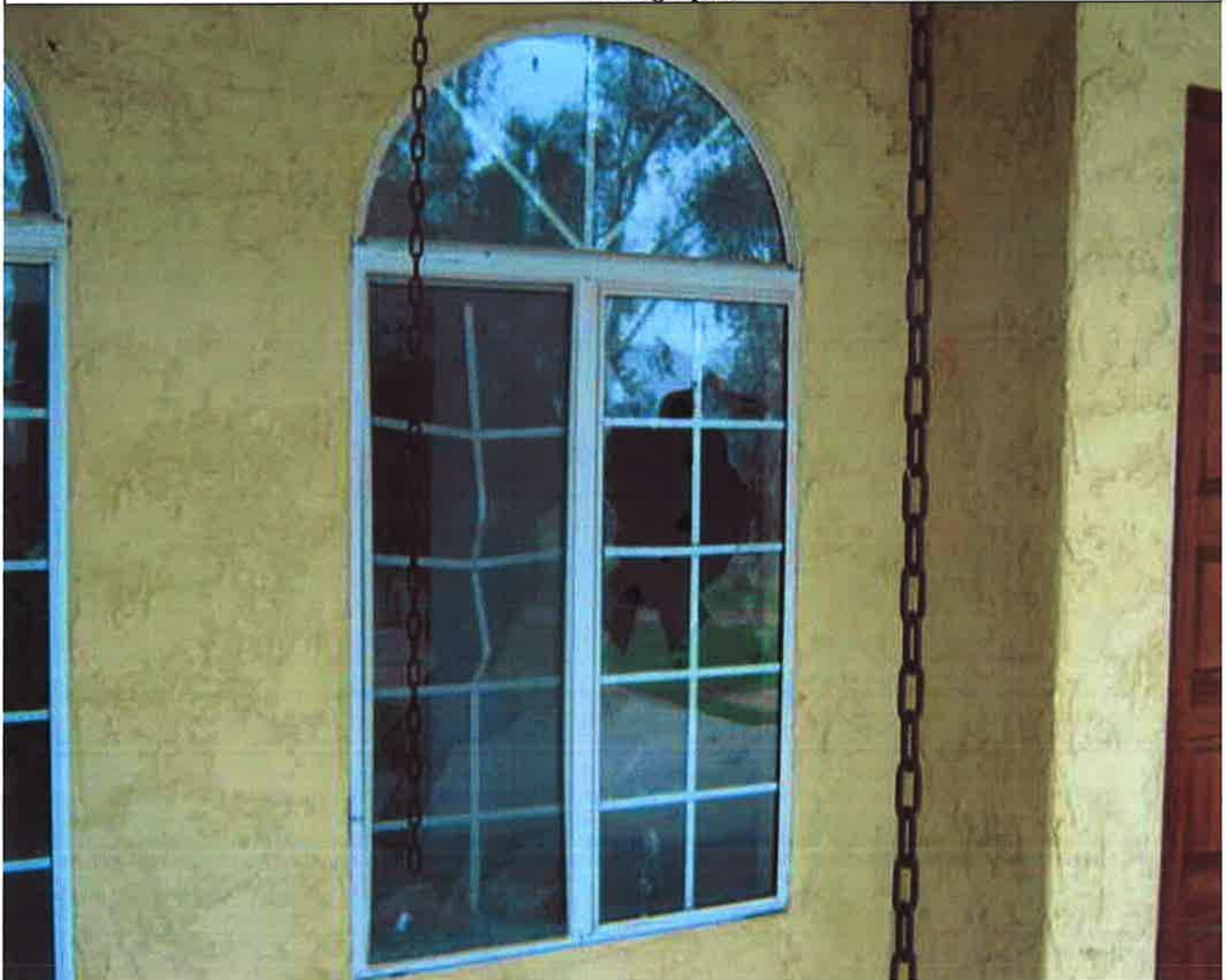
02/05/10 - Substandard Structure NOD# 13 - 02/05/2010
