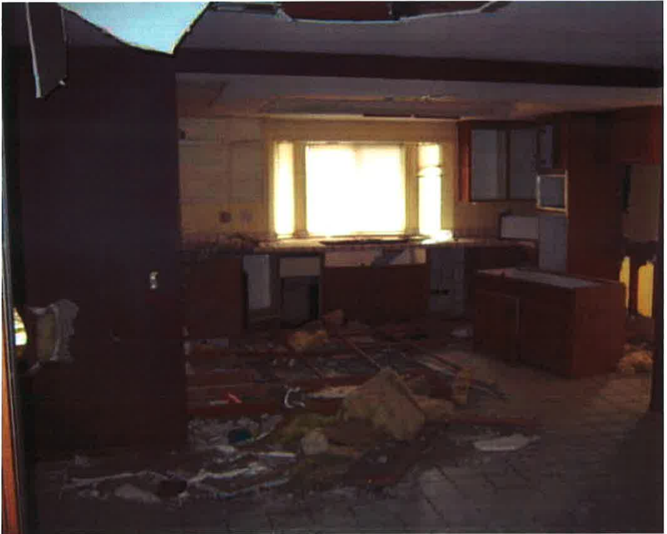
02/05/10 - Substandard Structure NOD# 1 - 02/05/2010
