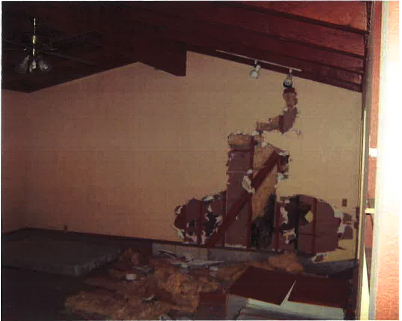
02/05/10 - Substandard Structure NOD# 2 - 02/05/2010
