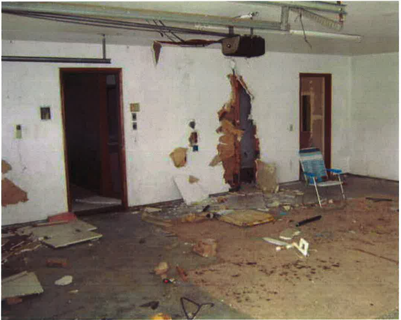
02/05/10 - Substandard Structure NOD# 10 - 02/05/2010
