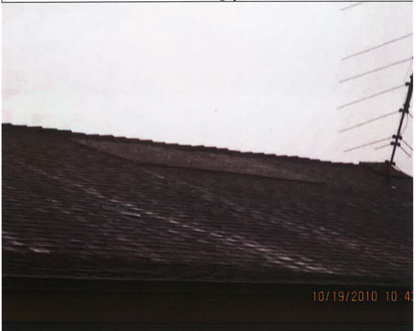
Roof has a hole in it from fire damaged. J. Kirchoff.10.19.10 006.jpg - 10/19/2010
