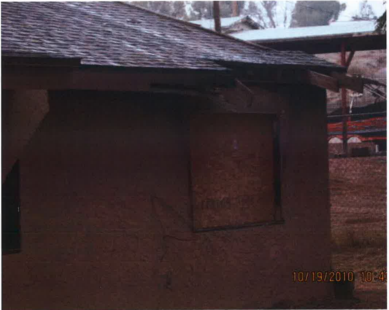
Window is broken out and roof is sagging from fire damage. J. Kirchoff.10.19.10 005.jpg - 10/19/20
