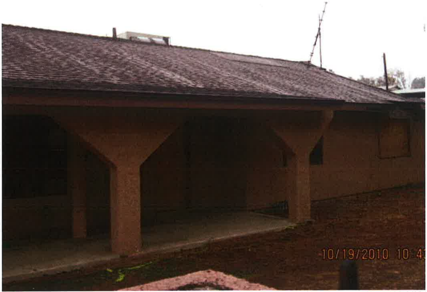
Windows are boarded but broken out along with the door. J. Kirchoff.10.19.10 004.jpg - 10/19/2010
