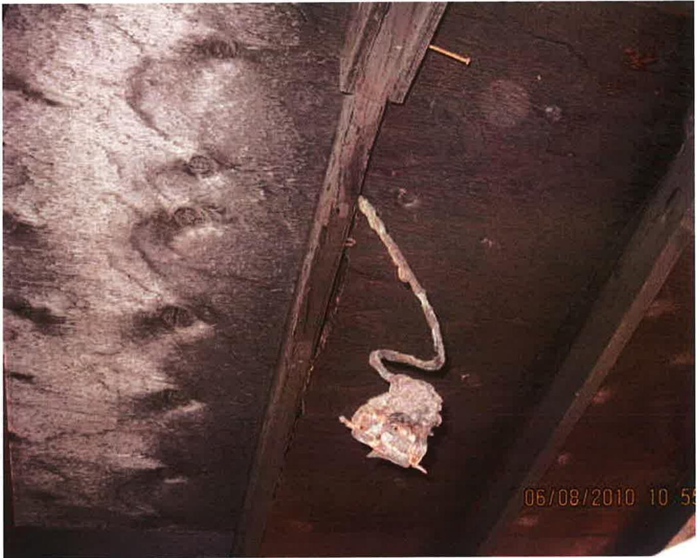
J.Wagner #80 Exposed wiring and fire damage. - 06/08/2010
