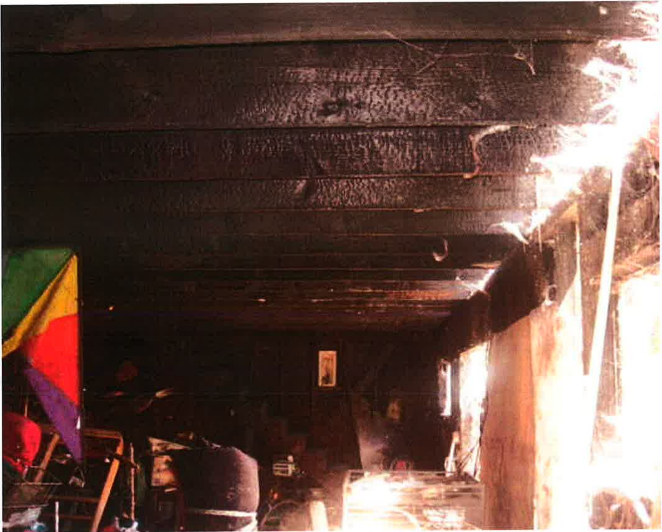
J.Wagner #80 Defect #16 extensive fire damage. - 06/08/2010
