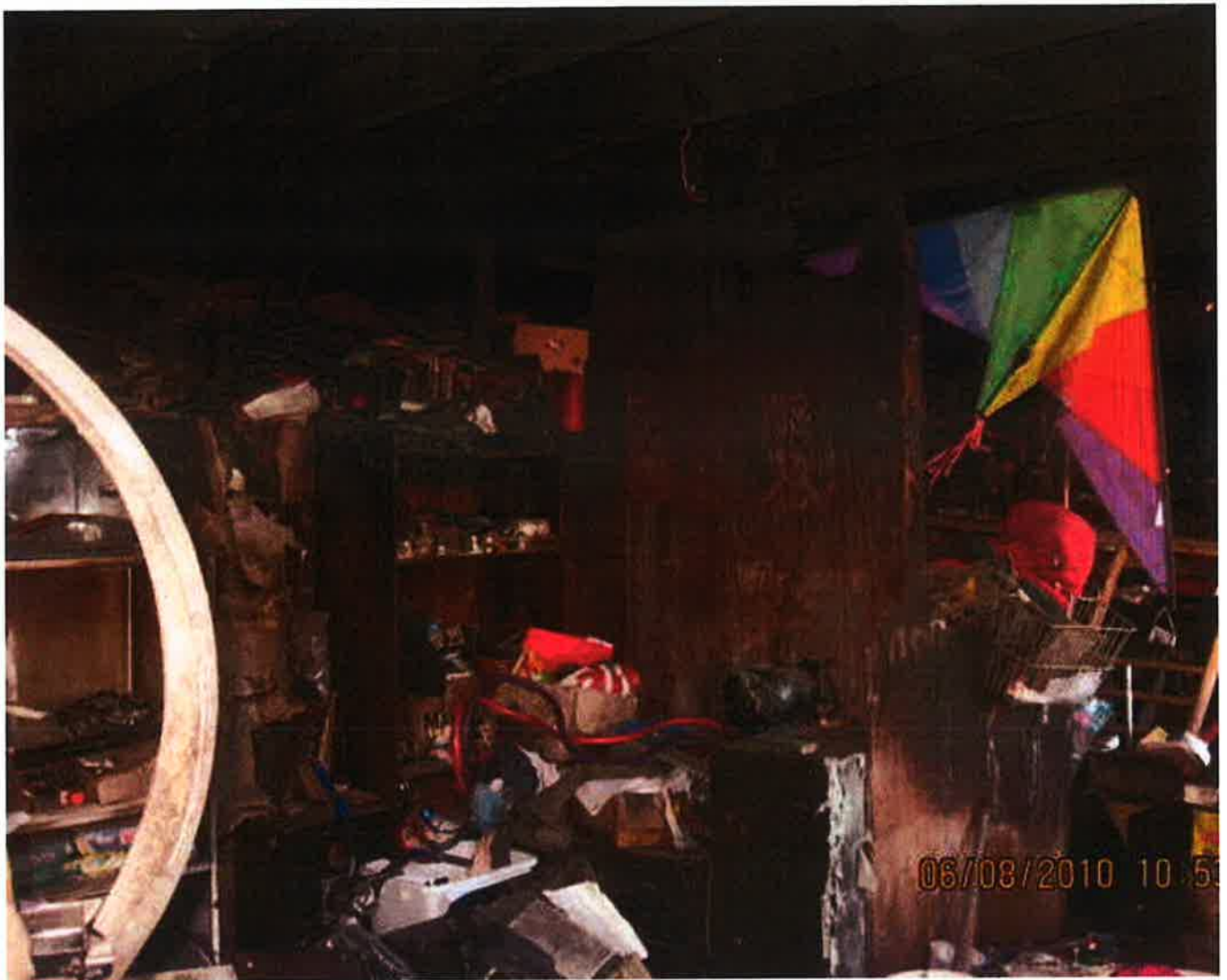
J.Wagner #80 Burned ceiling and fire damage. Defects #16 and 10 - 06/08/2010
