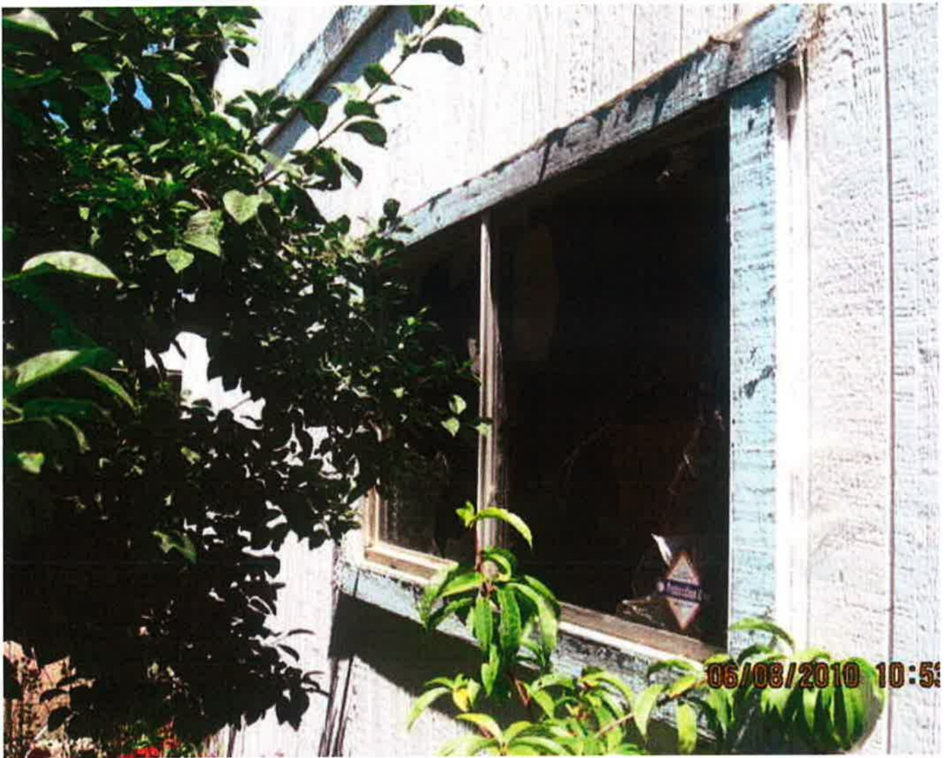
J.Wagner #80 Missing / broken window Defect #13 - 06/08/2010
