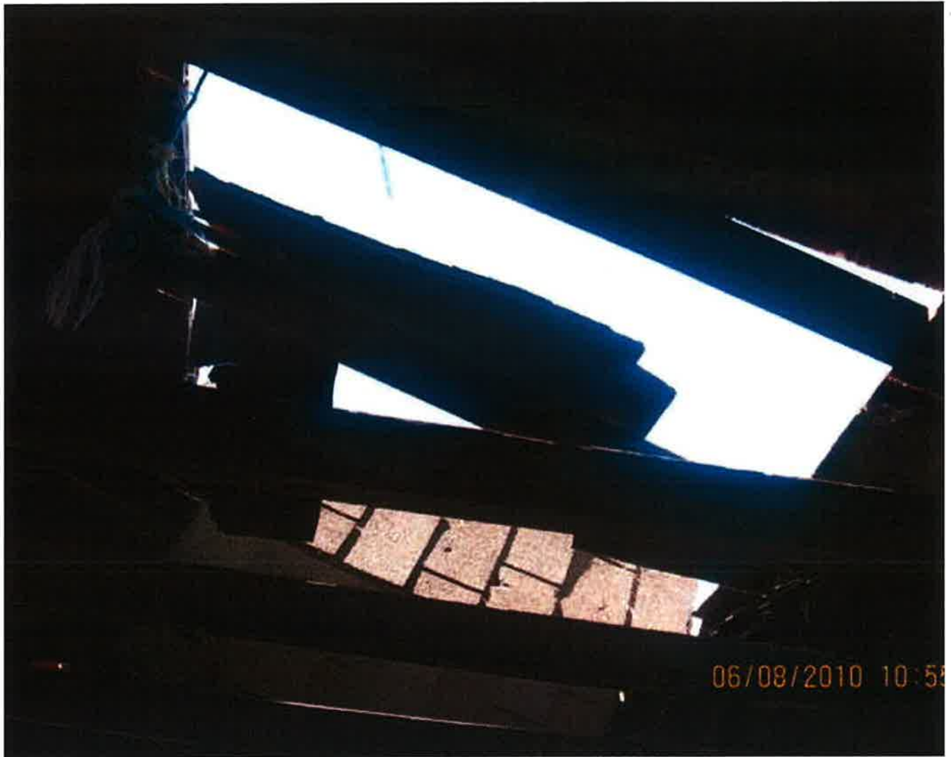
J.Wagner #80 Large hole in the roof. Defect #12 and 13 - 06/08/2010
