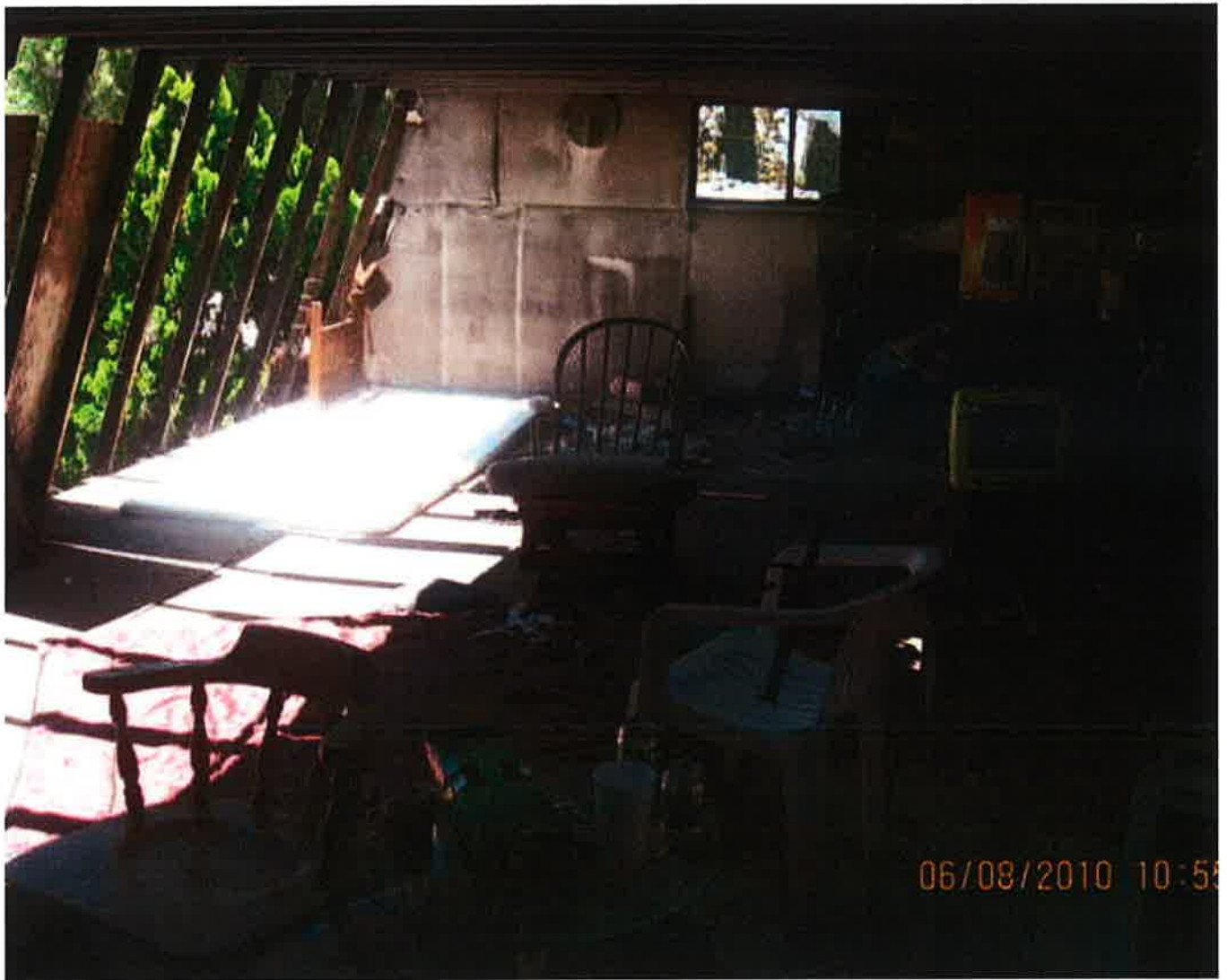
J.Wagner #80 2nd story room. Defect #12. Wall missing. Evidence of people still occupying structure 06/08/2010
