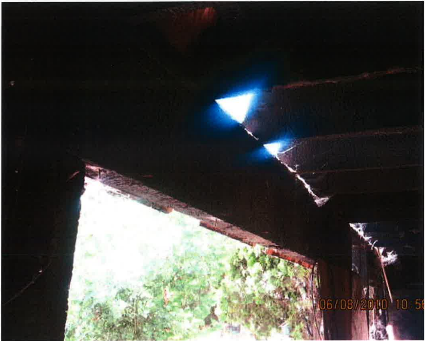
J.Wagner #80 Fire damage to load bearing beam in the structure. - 06/08/2010
