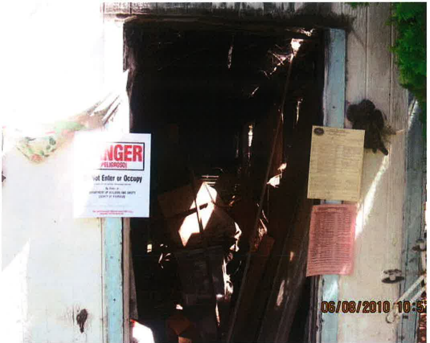
J.Wagner #80 NOD, NOV, and Danger sign posted to structure. - 06/08/2010
