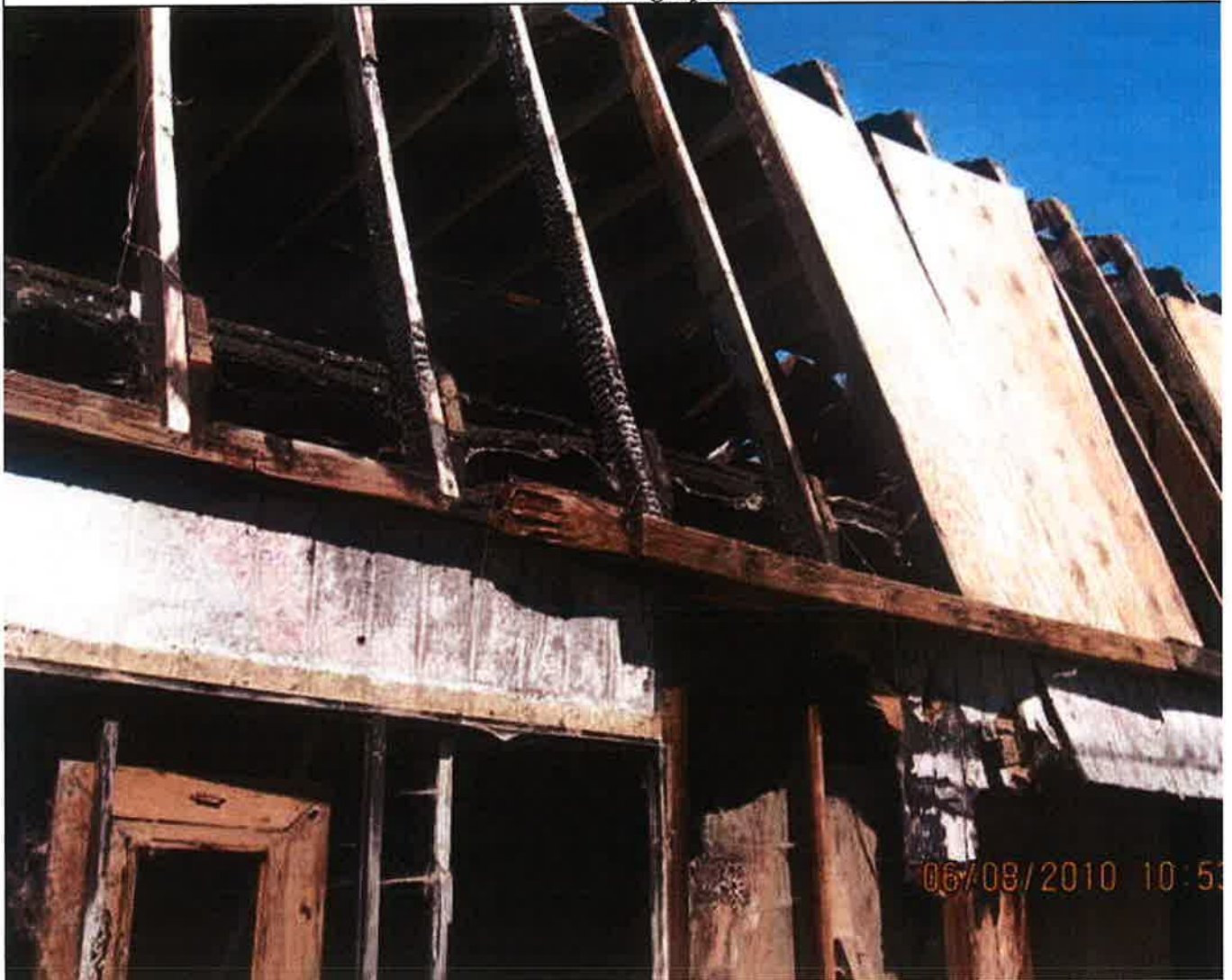
J.Wagner #80 Defect #11 and 13. Faulty weather protection. Members of ceiling and walls that sag, spl buckle - 06/08/2010
