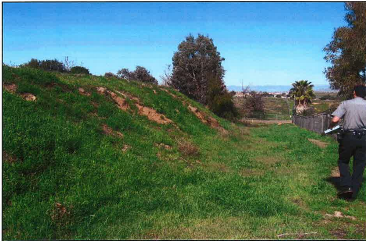
R Welch PHOTO # NOTES: Inspecting erosion on the 1/1 slope
