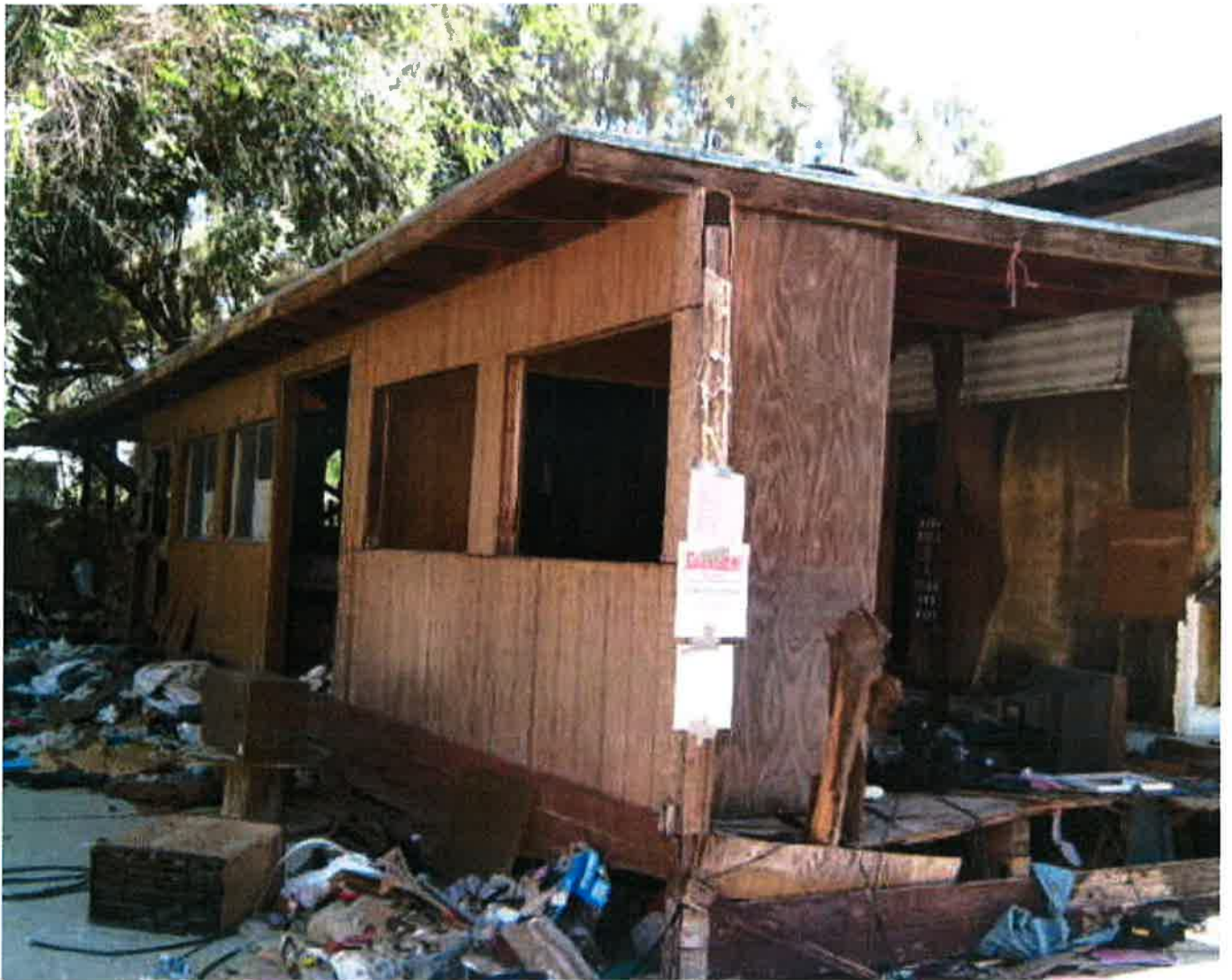
Substandard Structure - NOD# 9,11,13,14,17 - 07/17/2010
