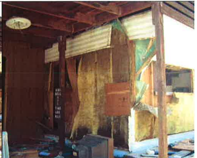
Substandard Structure - NOD # 9,11,13,14,17
