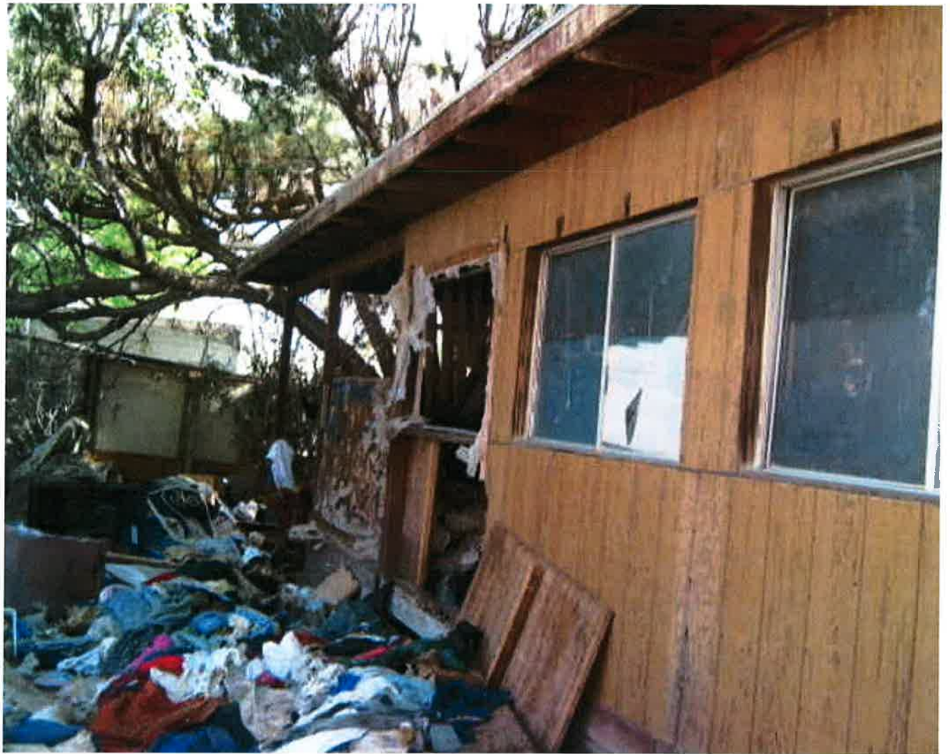
Substandard Structure - NOD# 10,13,14,17 - 07/17/2010
