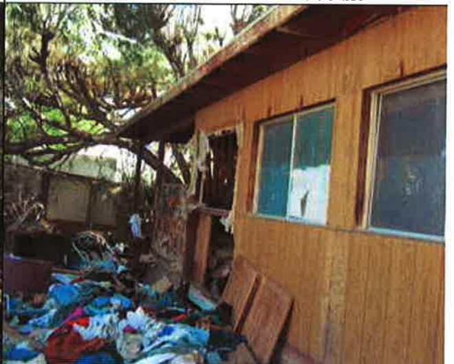
Substandard Structure - NOD# 10,13,14,17
