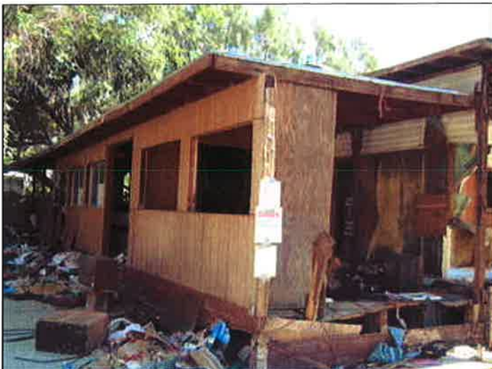
Substandard Structure - NOD# 9,11,13,14,17
