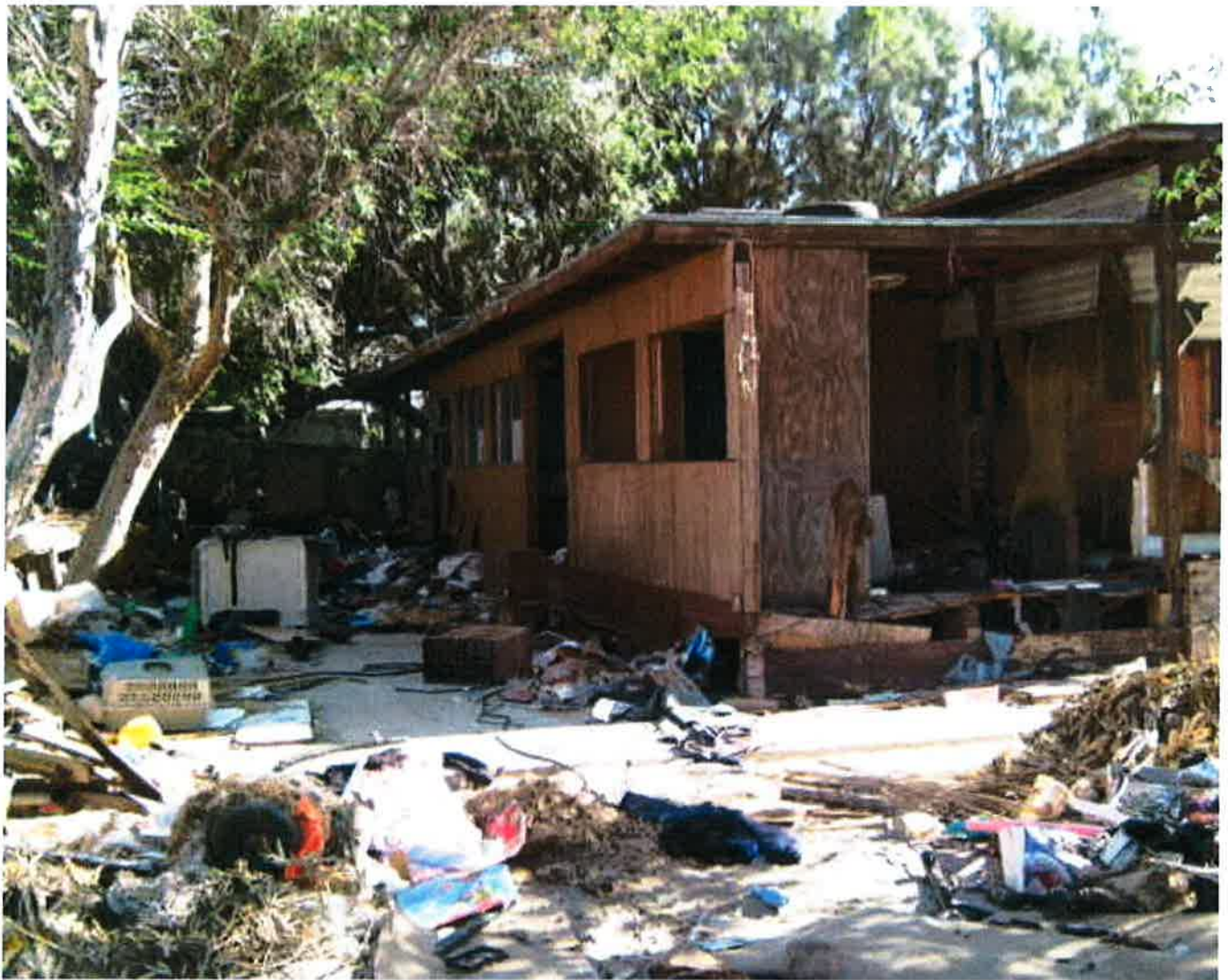
Accumulation of Rubbish - 07/17/2010
