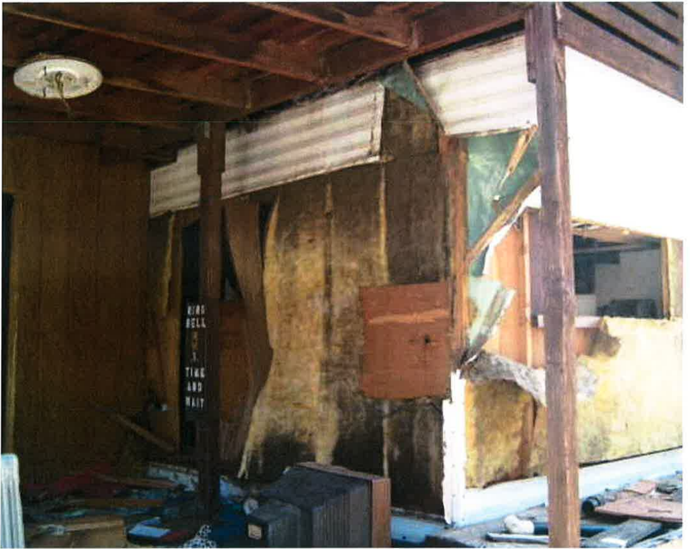
Substandard Structure - NOD # 9,11,13,14,17 - 07/17/2010
