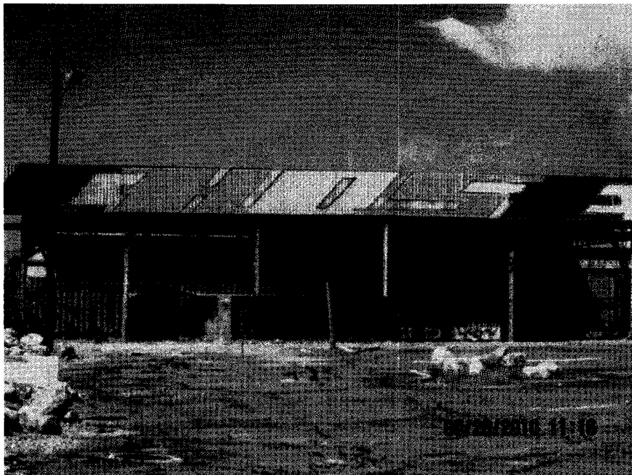
082610, CV1003317 - Substandard Structure - T Cervantes - 08/26/2010
