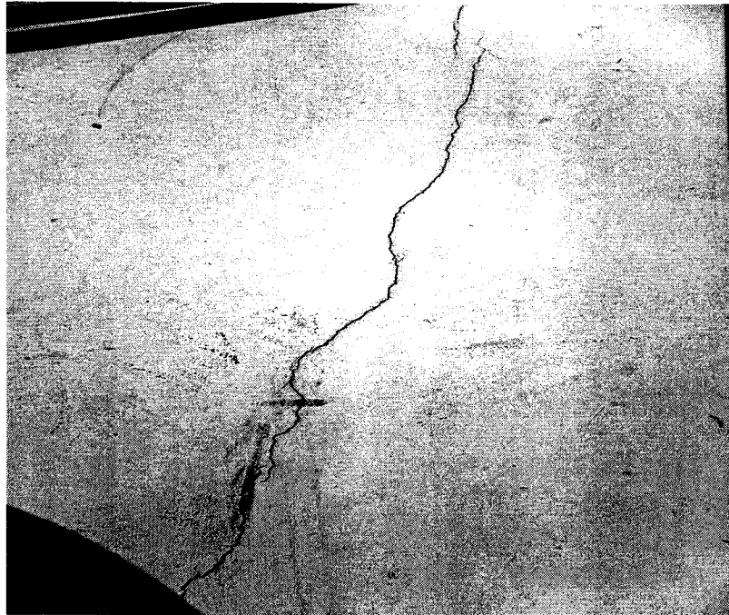
Picture 10 – Cracking on first floor perimeter wall
