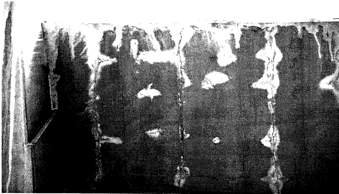
Picture 6- Cracking on perimeter cantilever slab
