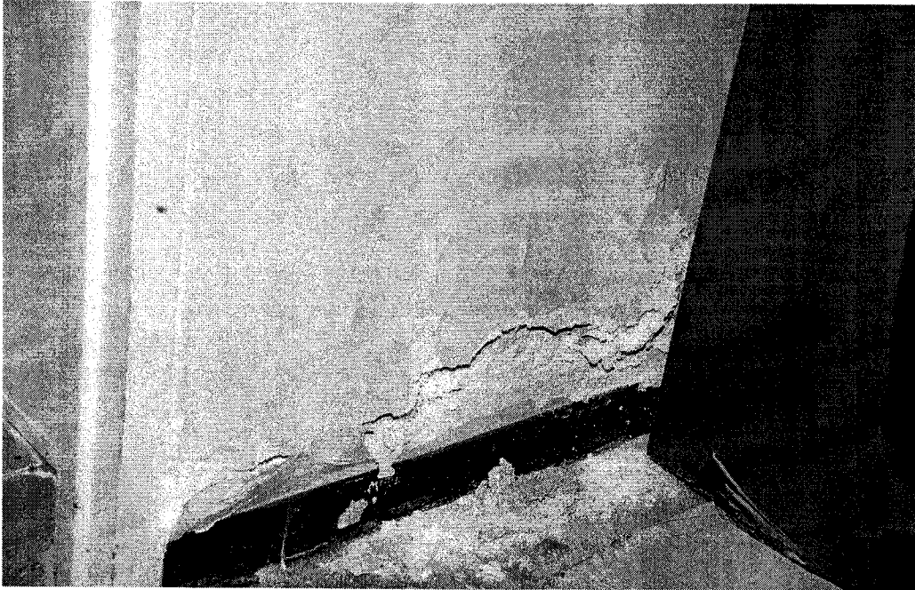
Picture 20 – Water-damaged interior partition
