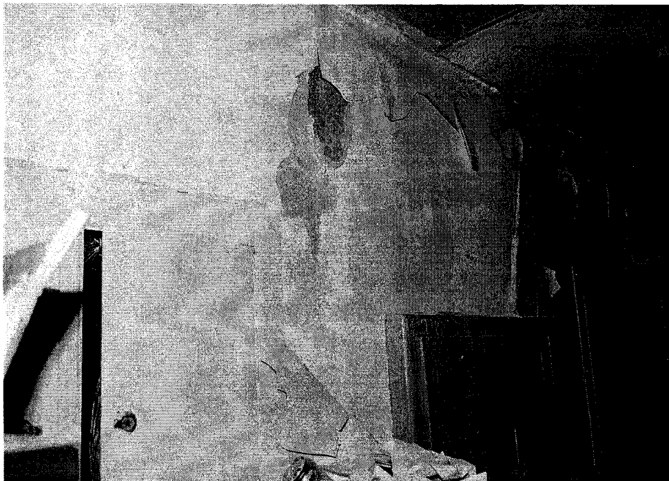
Picture 19 – Water-damaged interior partition
