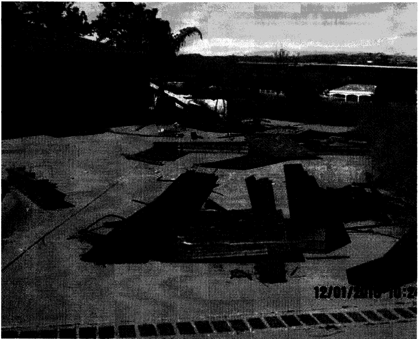
Photo #23 - accumulated rubbish - 12/01/2010
