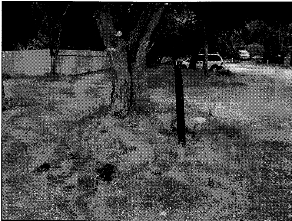
Photograph 14 – View looking south along the west side of the lodge structure. A 4-inch diameter PVC pipe possibly related to a septic tank system is in view in the foreground.
