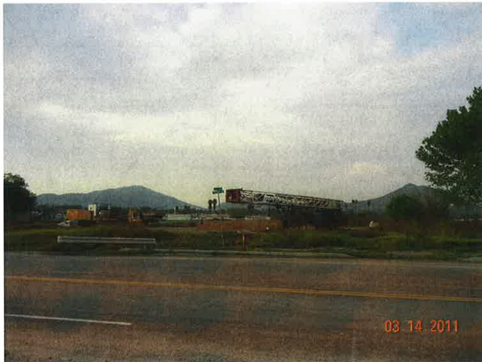
View looking north-northwest across 46th Street/Crestmore Road toward the Project site. Machinery and equipment for the construction of the well can be seen on-site.
