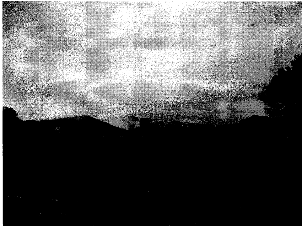
View looking north-northwest across 46th Street/Crestmore Road toward the Project site. Machinery and equipment for the construction of the well can be seen on-site.
