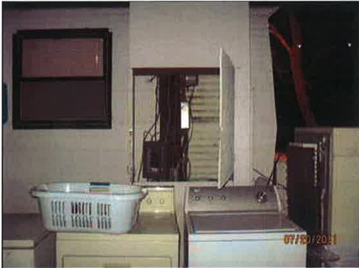
Appliances in front of meter access
