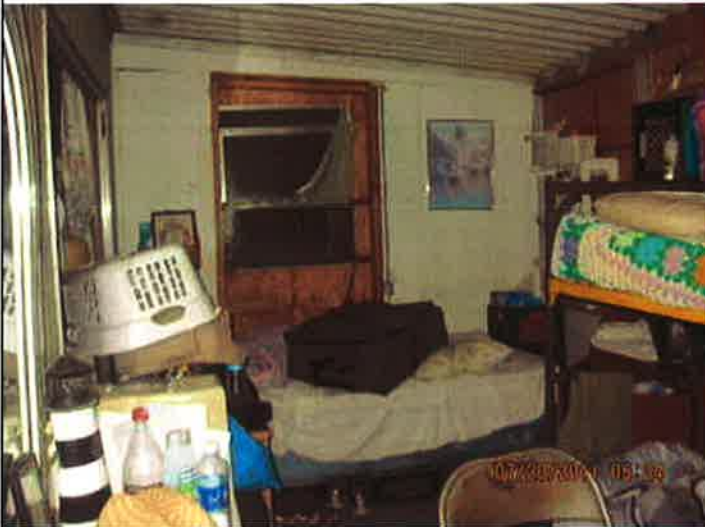
Johnston, Defect #15 - Window blocked by bunk beds and water cooler installed at window
