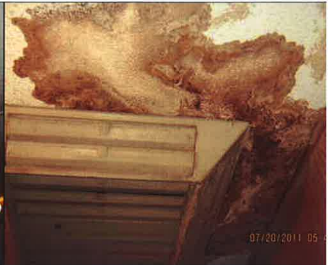
Johnston, Defect #11 & #12 - ceiling is bowing caused by water damage
