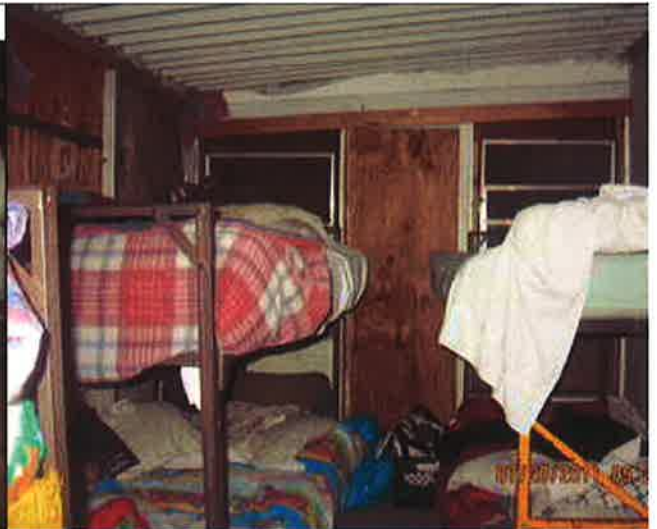
Johnston, Defect #15 & 18 - Window blocked by bunk beds
