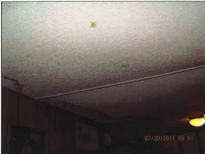
Johnston, Defect #11 - veiw of ceiling water damage inside mobile ceiling is bowing
