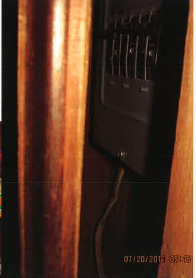
Johnston, Defect #15 - interior mobile elec. panel blocked by beds.
