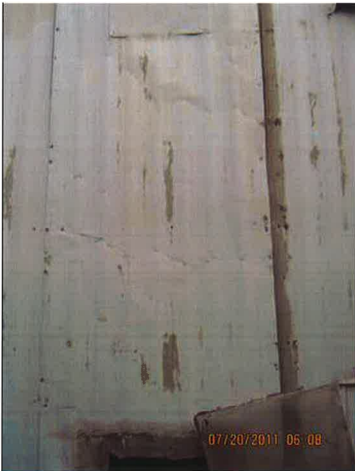
Johnston, Defect #7 - View of furnace unit compartment closed and sealed with mobile metal siding
