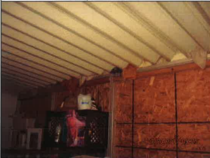
Johnston, Defect #13, corrugated alum ceiling no insulation and plywood only wall.
