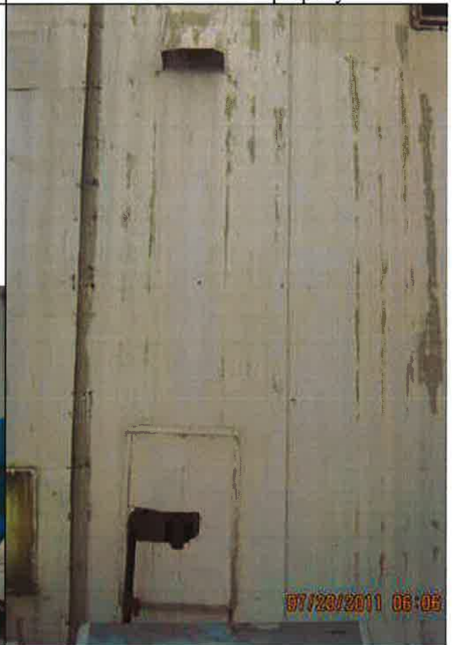
Johnston, Defect #4 - View of water heater area compartment closed and sealed with mobile home siding.
