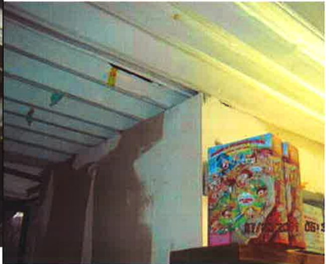
Exposed drywall in porch area.jpg
