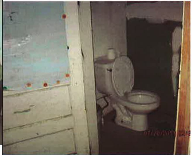
Exterior toilet room without sink or light.jpg
