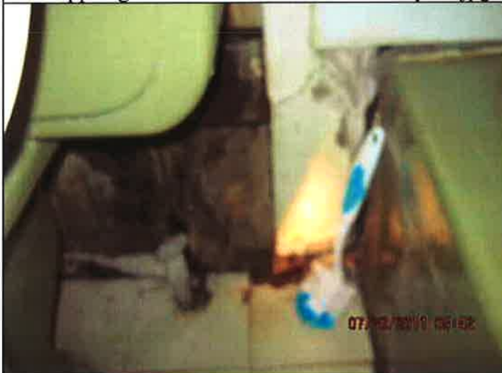
water damage in interior wall behind toilet.jpg
