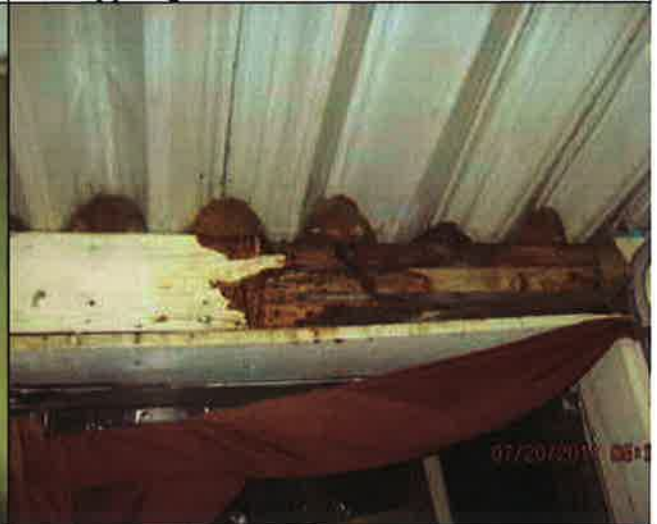
Water damage in porch-bunk room awning roof.
