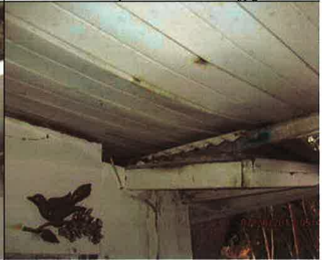
Damaged leaking awning.jpg
