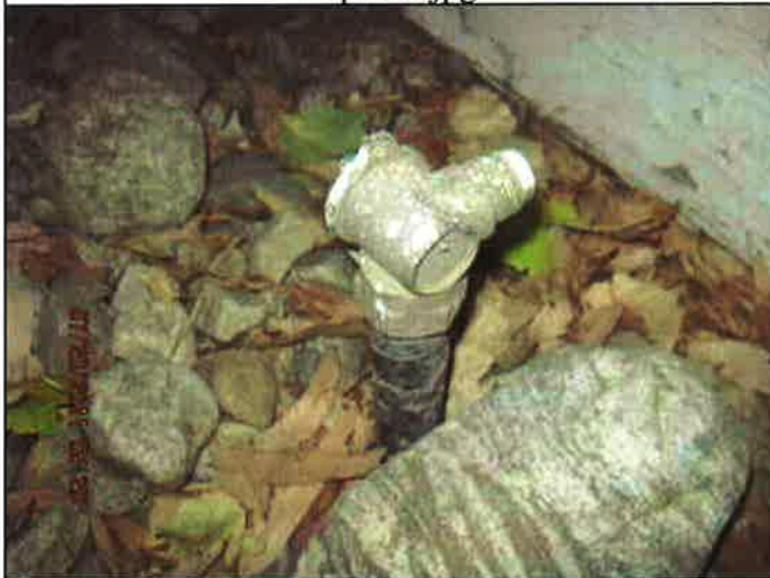
Uncapped gas line 3 behind mobile in rear yard.jpg
