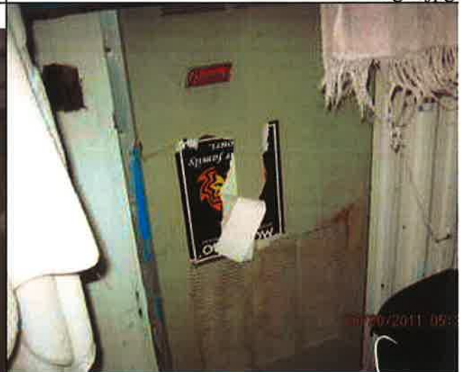
Furnace removed from interior of mobile and installed in exterior wall to heat enclosed porch.jpg
