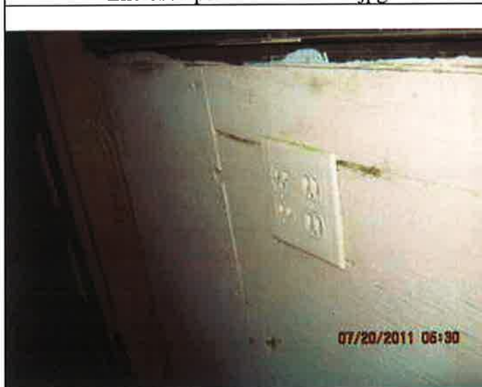
Exterior exposed non protected outlet.jpg
