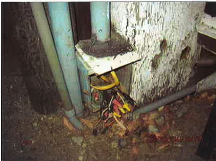
Exposed and live junction box below meter on pole.jpg
