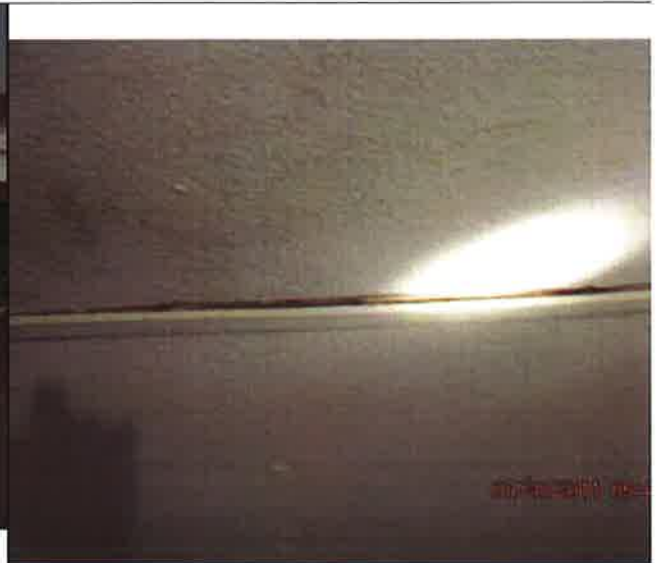
stain from leaking roof in mobile.jpg
