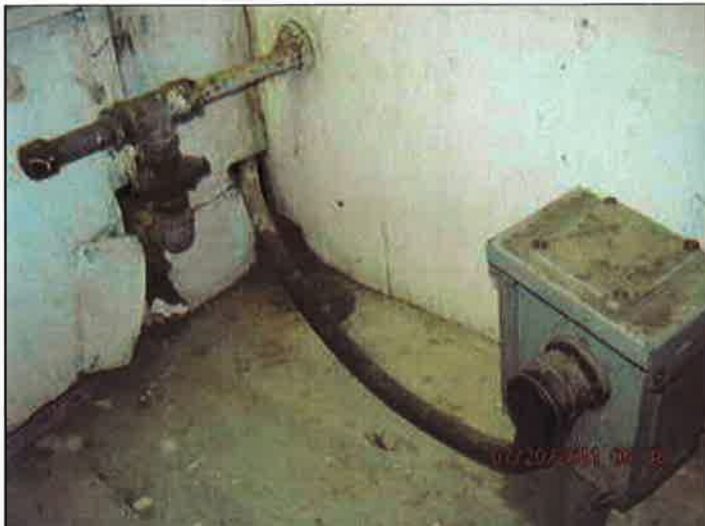
Power outlet from ground conduit to cord in porch area.jpg
