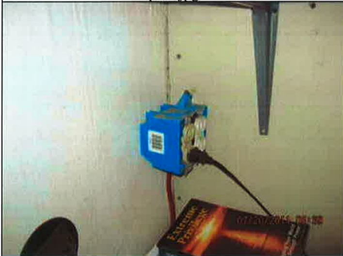
exposed duplex box with no plate powered by cord.jpg
