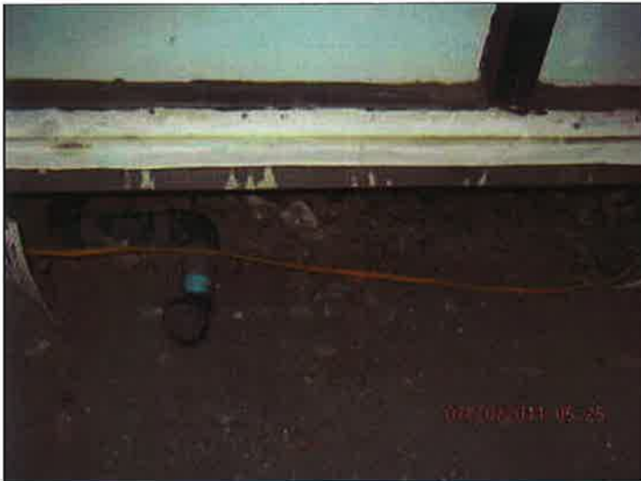
Romex wire laid on ground under porch and exposed.jpg
