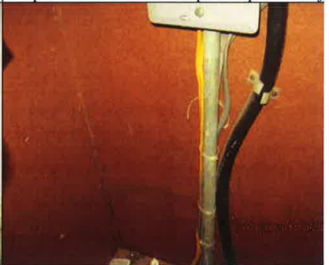
Exposed romex running from interior panel.jpg
