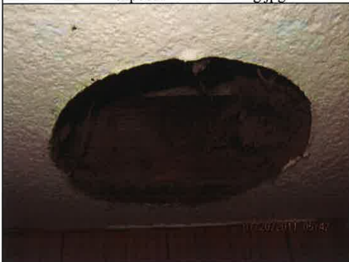
hole in bathroom ceiling.jpg
