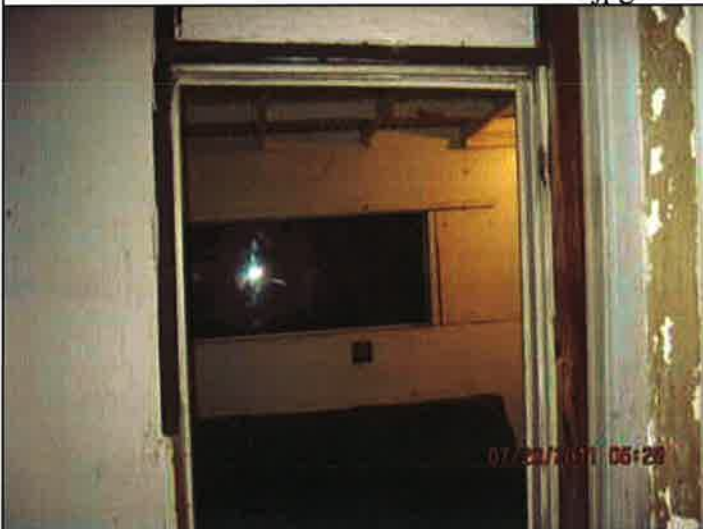
rear door way to yard from enclosed carport (exposed framing holding up carport).jpg
