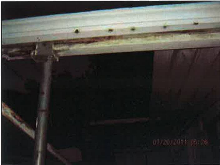
Awning missing pans and header.jpg
