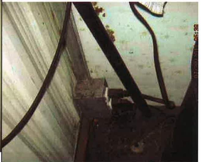
exposed outlet box without plate in porch area.jpg
