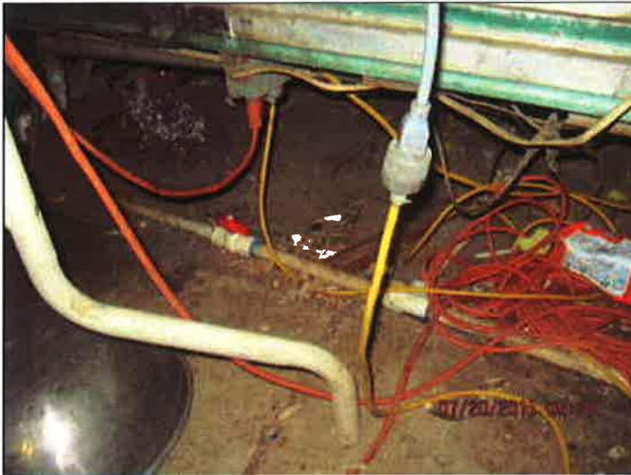
Plugs and wiring to exterior coffee bar in carport.jpg
