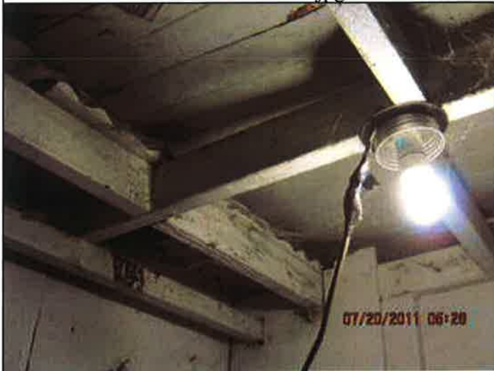
Carport light using damaged cord.jpg
