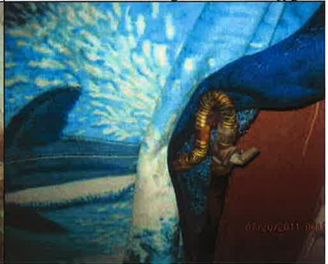
Uncapped gas line beside bed in demoed kitchen.
