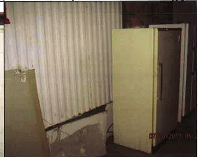
Energized and in use refrigerators (2) outside under carport awning.jpg
