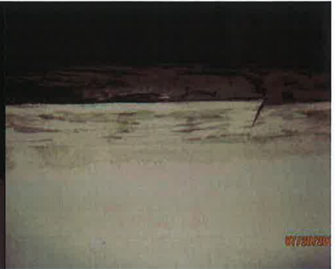
rotted eves on west side of mobile/D.Parra
