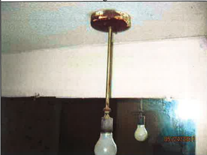
Repaired as requested. JHeagstedt
