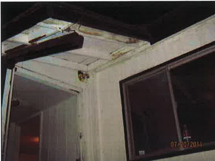
unpermitted delapidated addition to entrance of mobile/D.Parra
