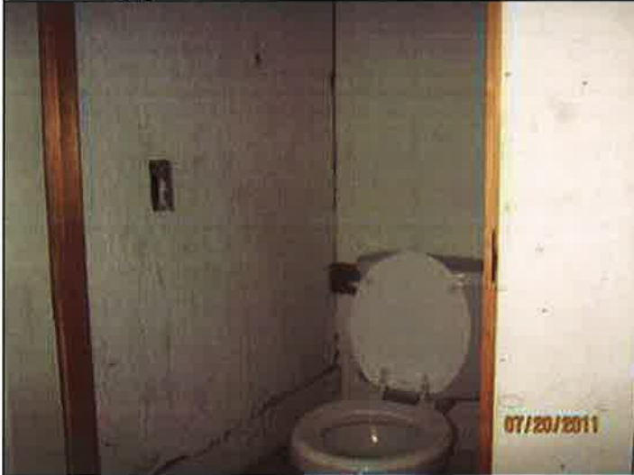
unpermitted bathroom addition accessible from exterior only/D.Parra
