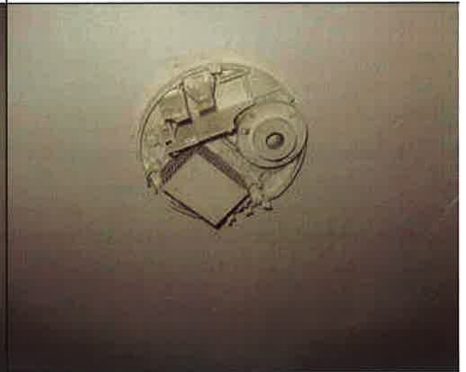
broken fire alarm/D.Parra
