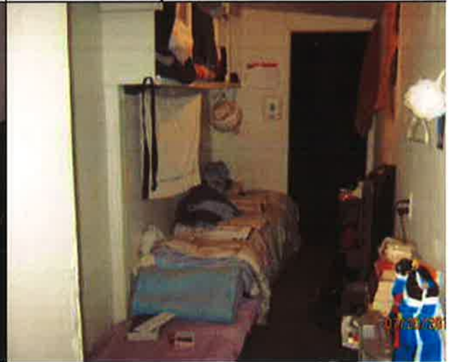
2 sleeping areas set up in unpermitted room addition/D.Parra
