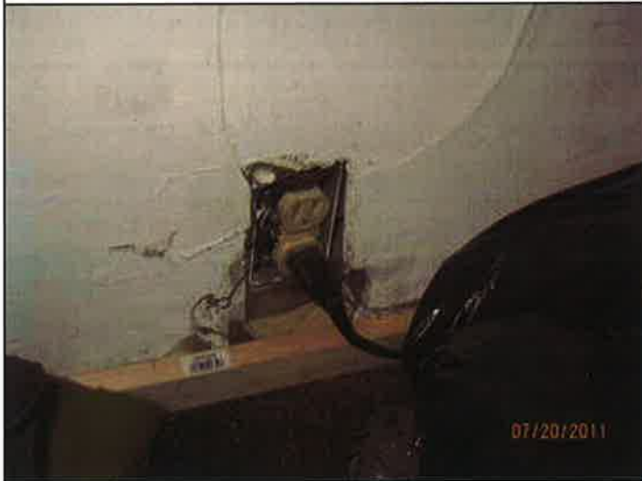
electrical outlet no face plate near bed in front room/D.Parra
