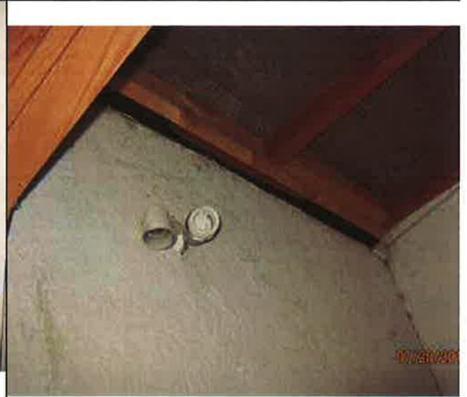
electrical to unpermitted bathroom addition/D.Parra
