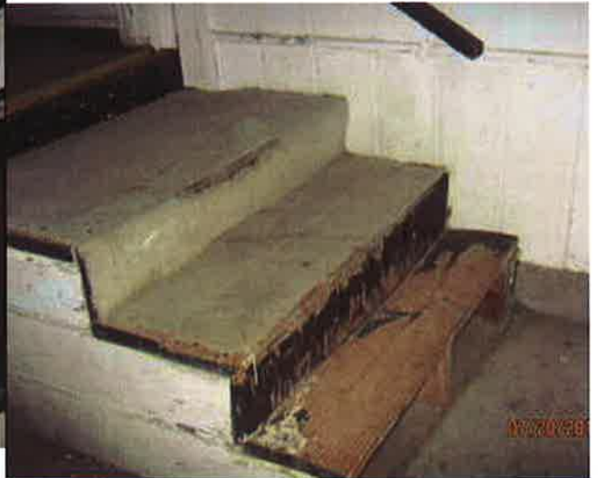
slightly rotted stairs to entrance of mobile/D.Parra
