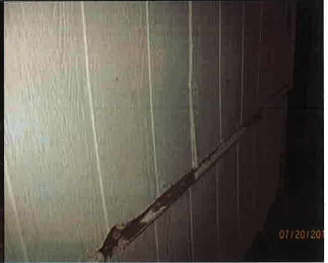
crack on exterior of west side of mobile/D.Parra
