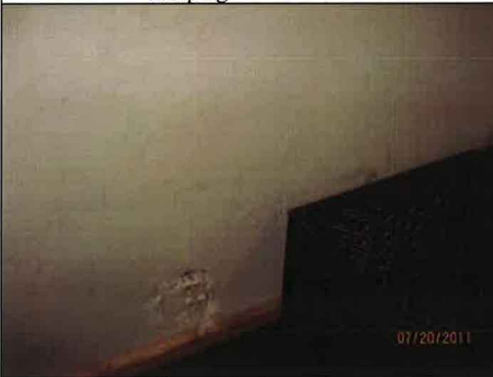
outlet with damaged wall around it/ D.Parra
