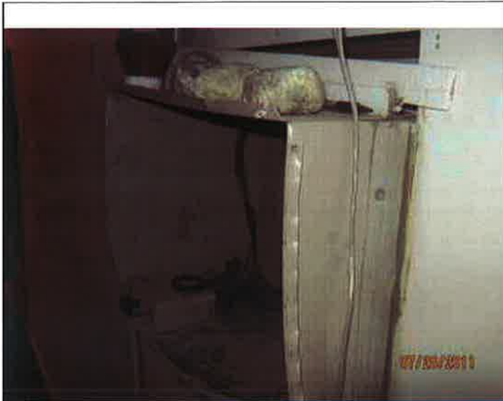
air conditioner with spliced electrical/D.Parra
