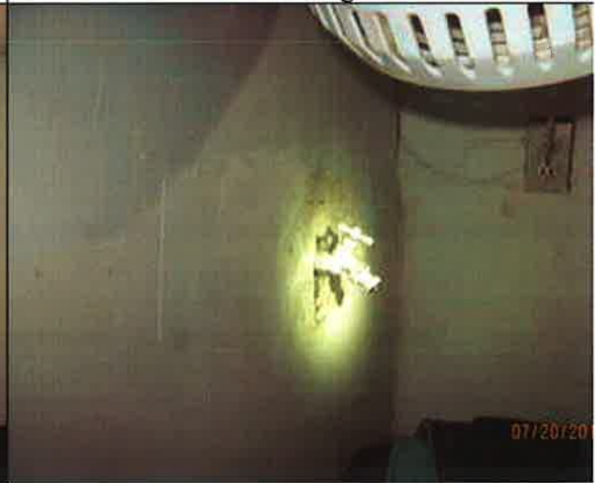
faucet protruding from wall in unpermitted room addition/D.Parra
