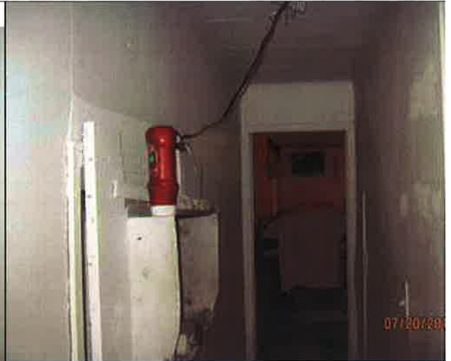
air conditioner plugged into ceiling lighting fixture/D.Parra
