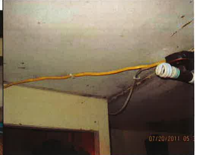
unprotected wiring at light fixture mobile. M. Villanueva
