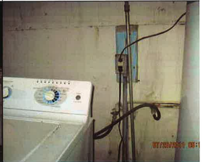
close up of washer and electrical. M. Villanueva
