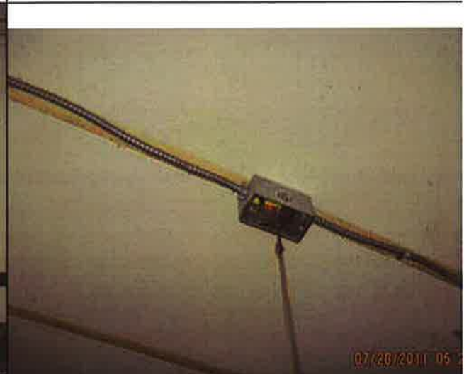
unprotected wiring at junction box. M. Villanueva
