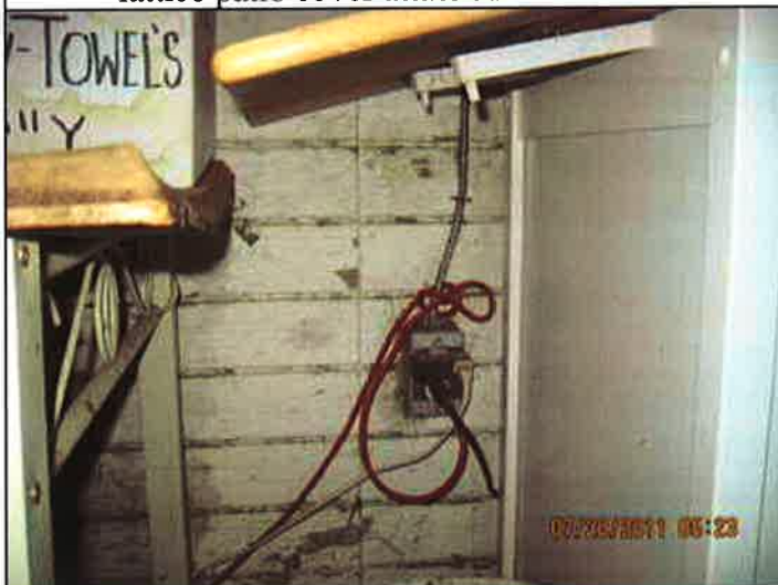
close up electrical outlet outside of structure. M. Villanueva
