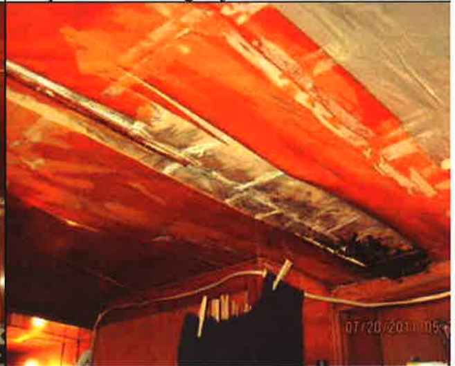
water damage and repair ceiling of mobile. M Villanueva
