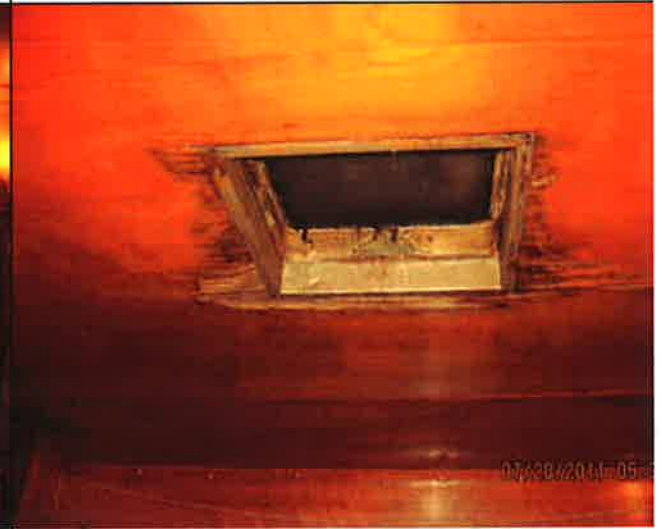
water damage around vent of mobile. M. Villanu
