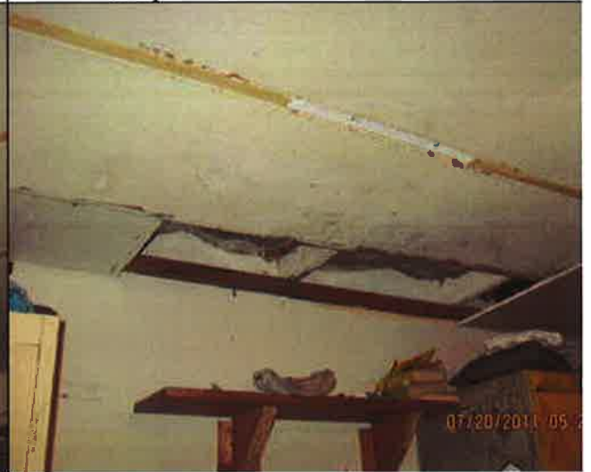
ceiling damage and exposed insulation sleep area M. Villanueva
