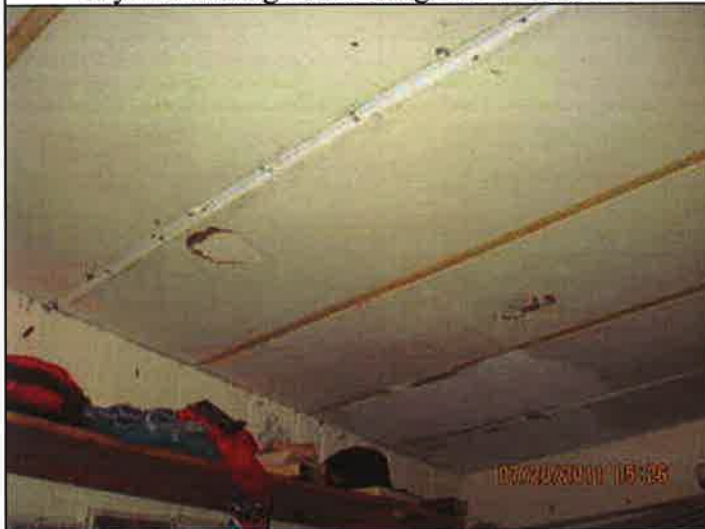
overall ceiling damage near front entrance. M. Villanueva
