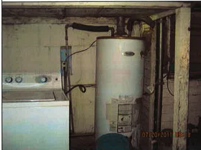
overall water heater no strapping. M. Villanueva
