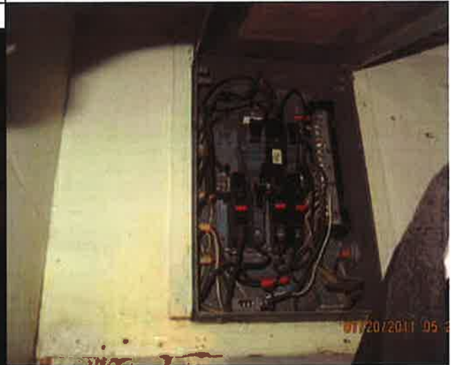
missing dead front on electrical panel near sleep area #2. M. Villanueva
