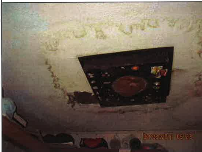
ceiling of structure drywall peeling and water damage. M. Villanueva
