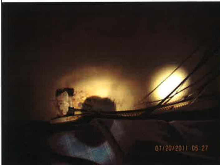
unprotected wiring sleep area #2. M. Villanueva
