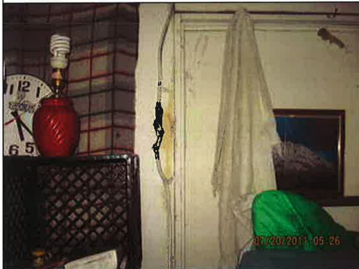
spliced wiring and egress door blocked by bunk. M. Villanueva
