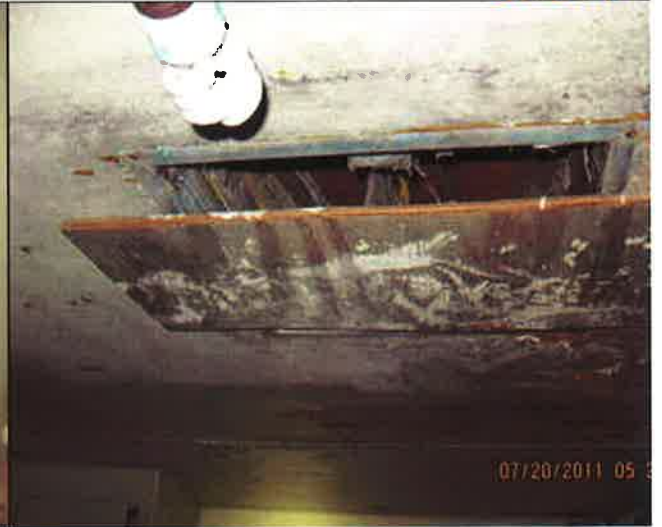
ceiling and water damage to moible. M. Villanue
