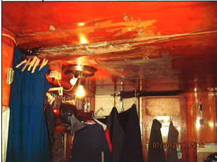
unprotected wiring at light fixture of mobile. M. Villanueva
