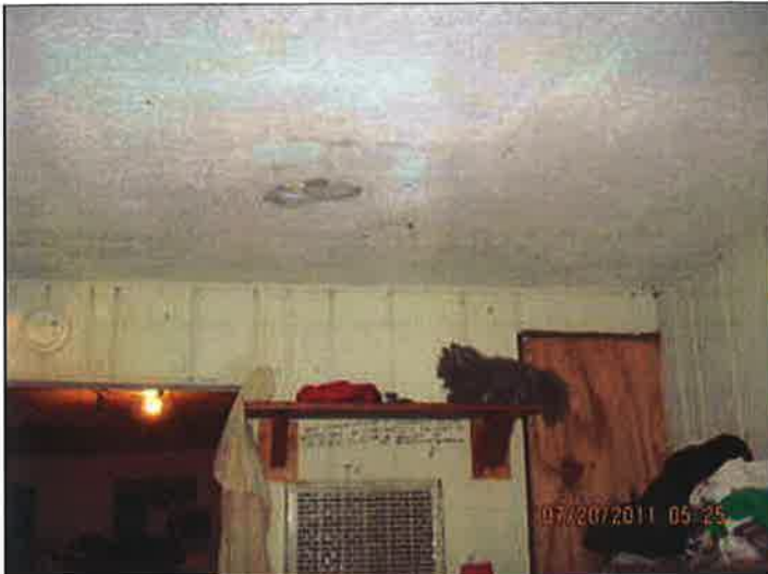
drywall damage on ceiling. M. Villanueva
