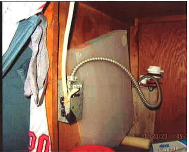
unprotected wiring at junction box. M. Villanue
