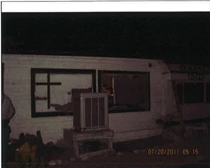
partially blocked window. M. Villanueva
