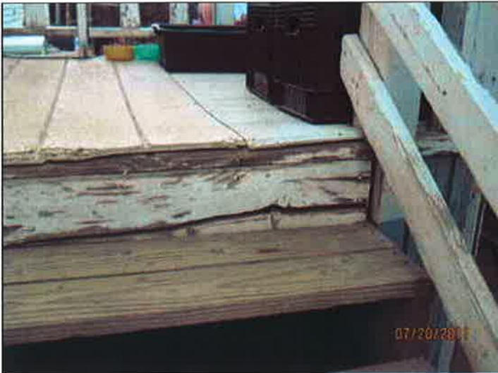
CForrey / 07/20/11 - Defect # 14 - dilapidated side deck
