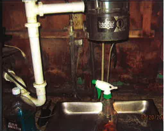
CForrey / 07/20/11 - Defect #10 wall missing in cabinet under sink
