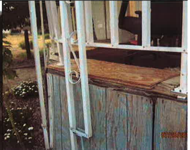
CForrey / 07/20/11 - Defect # 14, dilapidated fro deck
