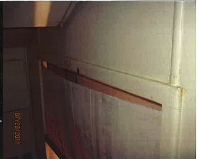
CForrey / 07/20/11 - open light fixture above cooking facilities
