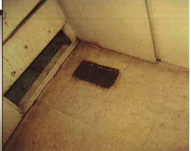
CForrey / 07/20/11 - Defect #14 - Lack of maintenance
