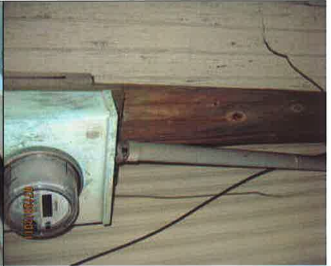
CForrey / 07/20/11 - Defect #6 - main power sup not secured to power pole
