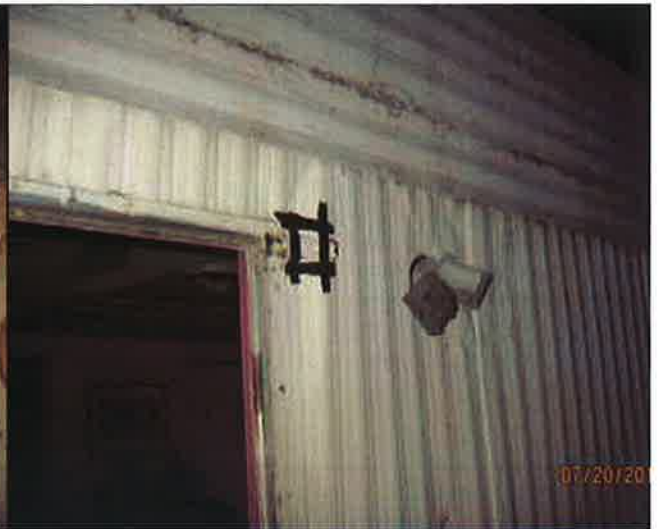
CForrey / 07/20/11 - Defect #5 - missing light at door
