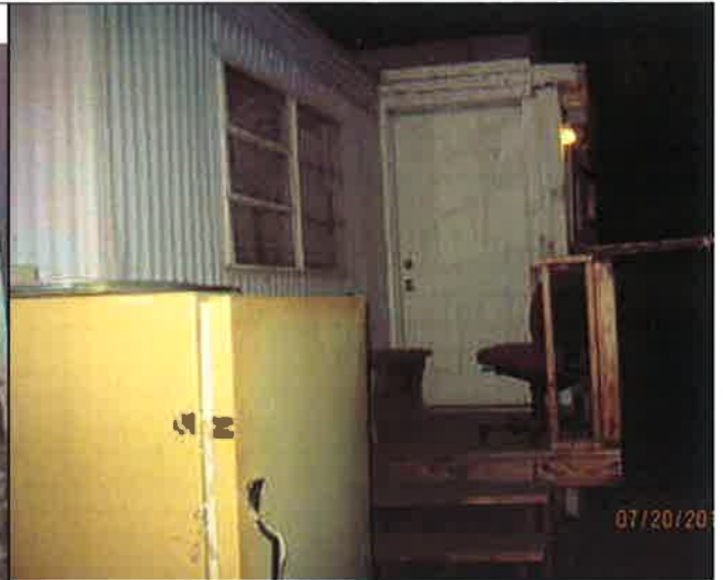
CForrey / 07/20/11 - Defect #19 exterior of overs bedroom, Defect # 5 missing exit door light
