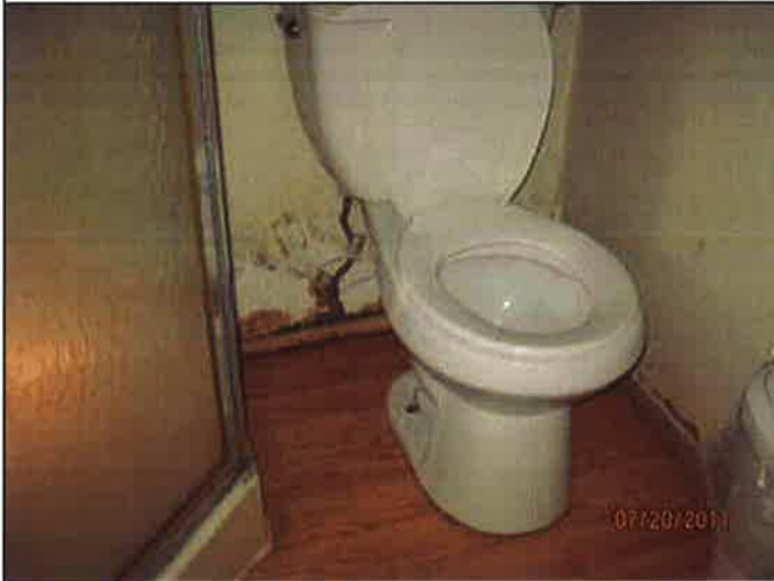
CForrey / 07/20/11 - Defect #12 - damp/dry rot in bathroom
