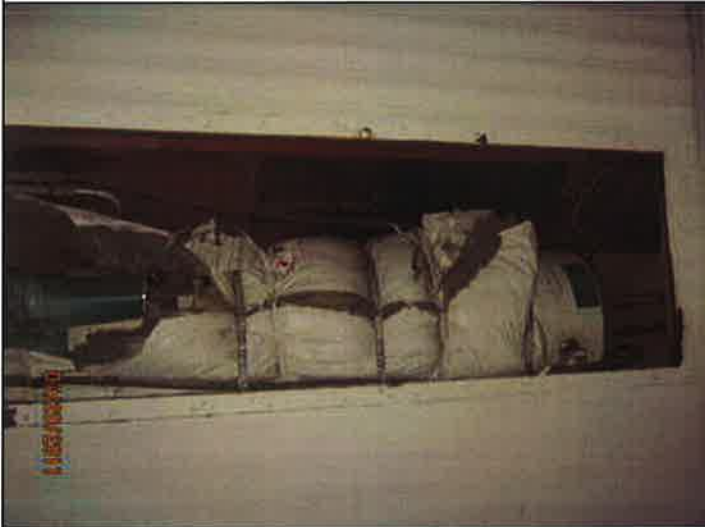
CForrey / 07/20/11 - Water heater strapped and vented
