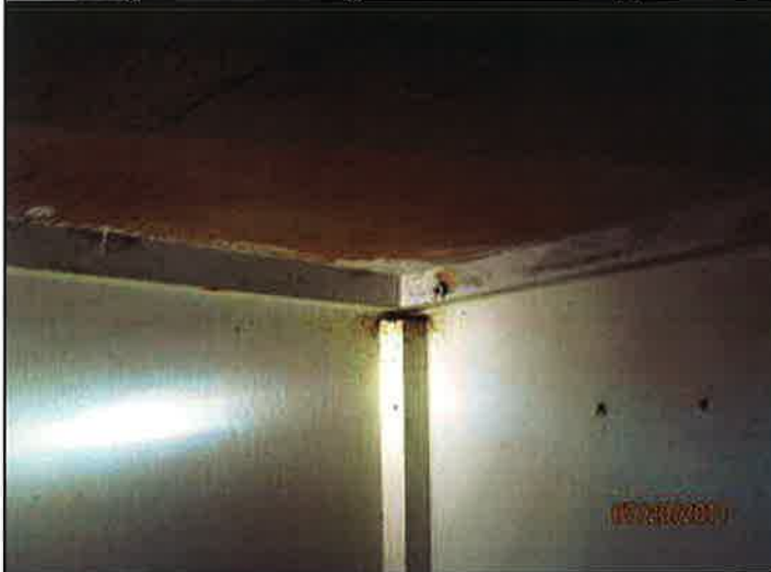
CForrey / 07/20/11 - Defect #14 - cockroach infestation above stove
