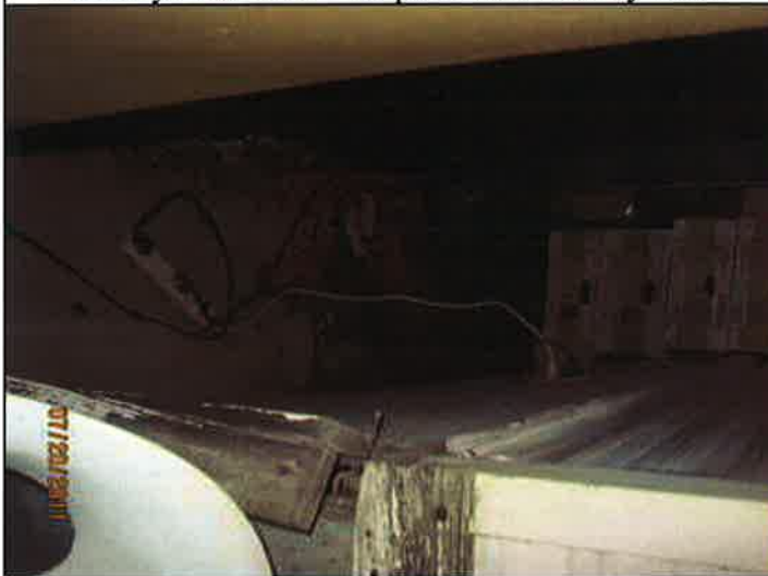
CForrey / 07/20/11 - Defect #6 - exterior reffridgerators using extension cords
