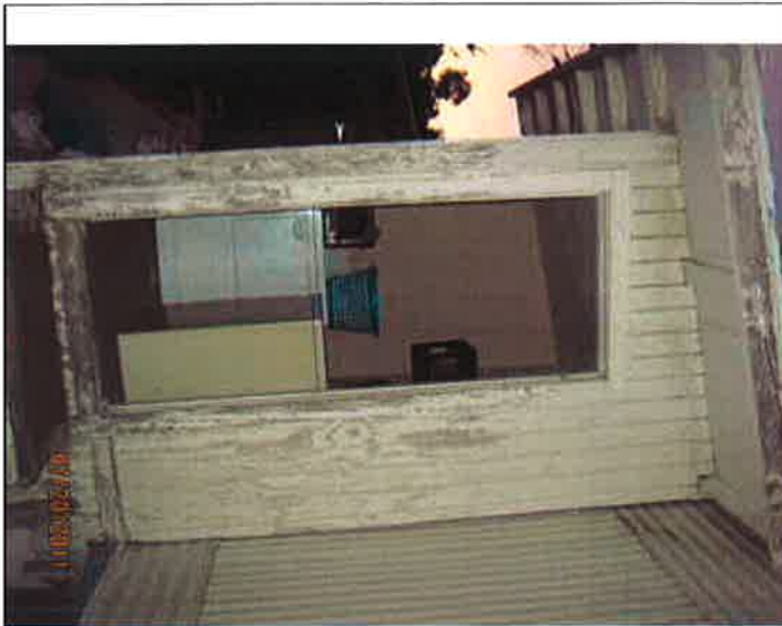
CForrey / 07/20/11 - Unpermitted laundry room
