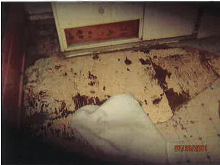
CForrey / 07/20/11 - Defect #9 - deteriorated bathroom floor
