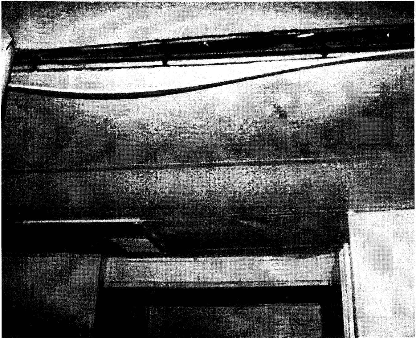
E. Torres; sagging ceiling in ssmh-defects 11, 14, 17 - 06/25/2010
