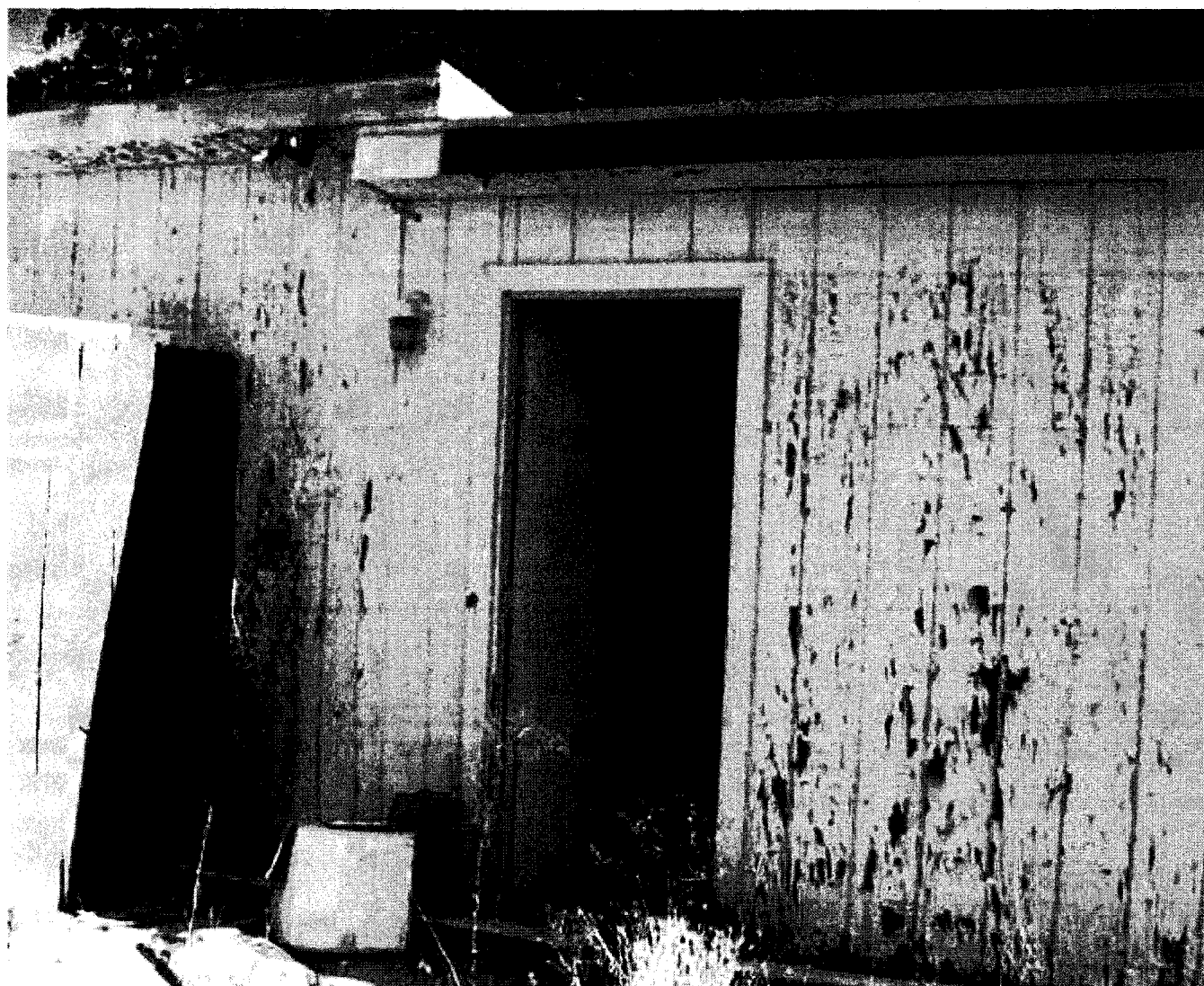
L Lyon - Rubbish at the garage door. - 10/26/2010
