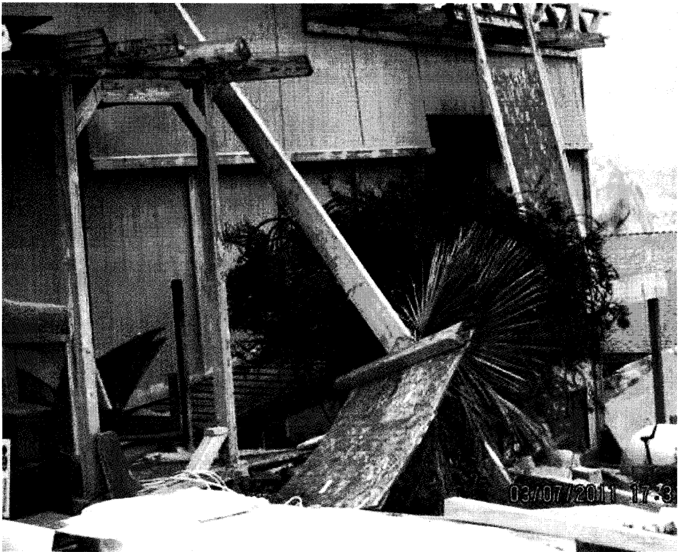
Photo #3 - Defects 12 and 13 - 03/07/2011
