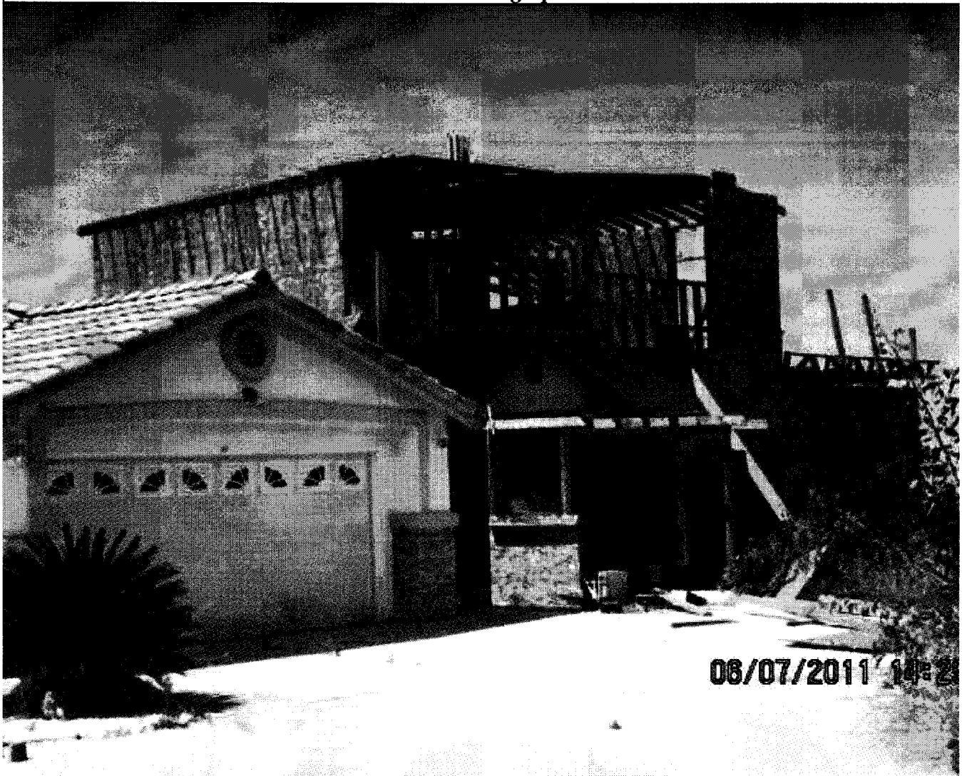
Photo #1 - Substandard structure from the roadway. RW - 06/07/2011
