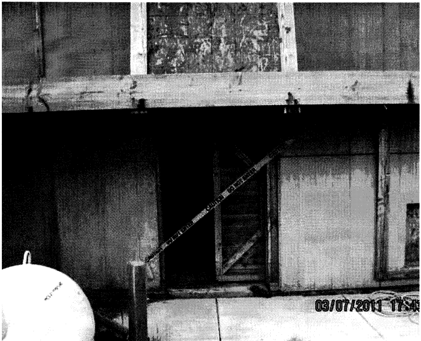
Photo #18 - Defect 17, open sliding door - public nuisance - 03/07/2011
