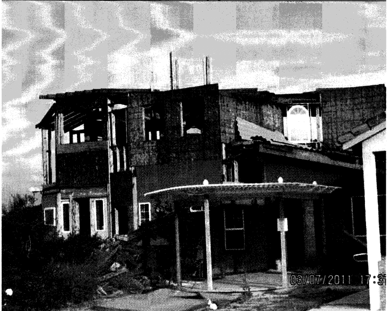
Photo #1 - rear of substandard structure/cwp defects 12,13,14,17 - 03/07/2011
