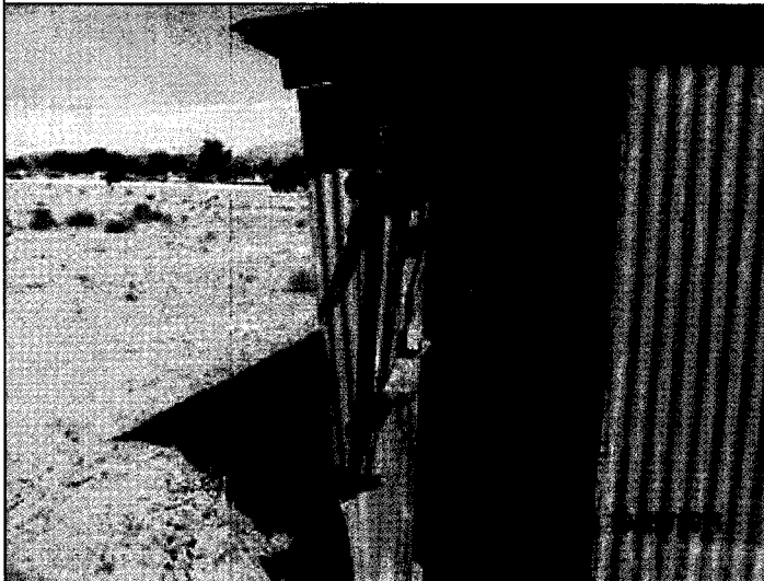
M Sanders 102811 - SSS # 1 broken verticle member
