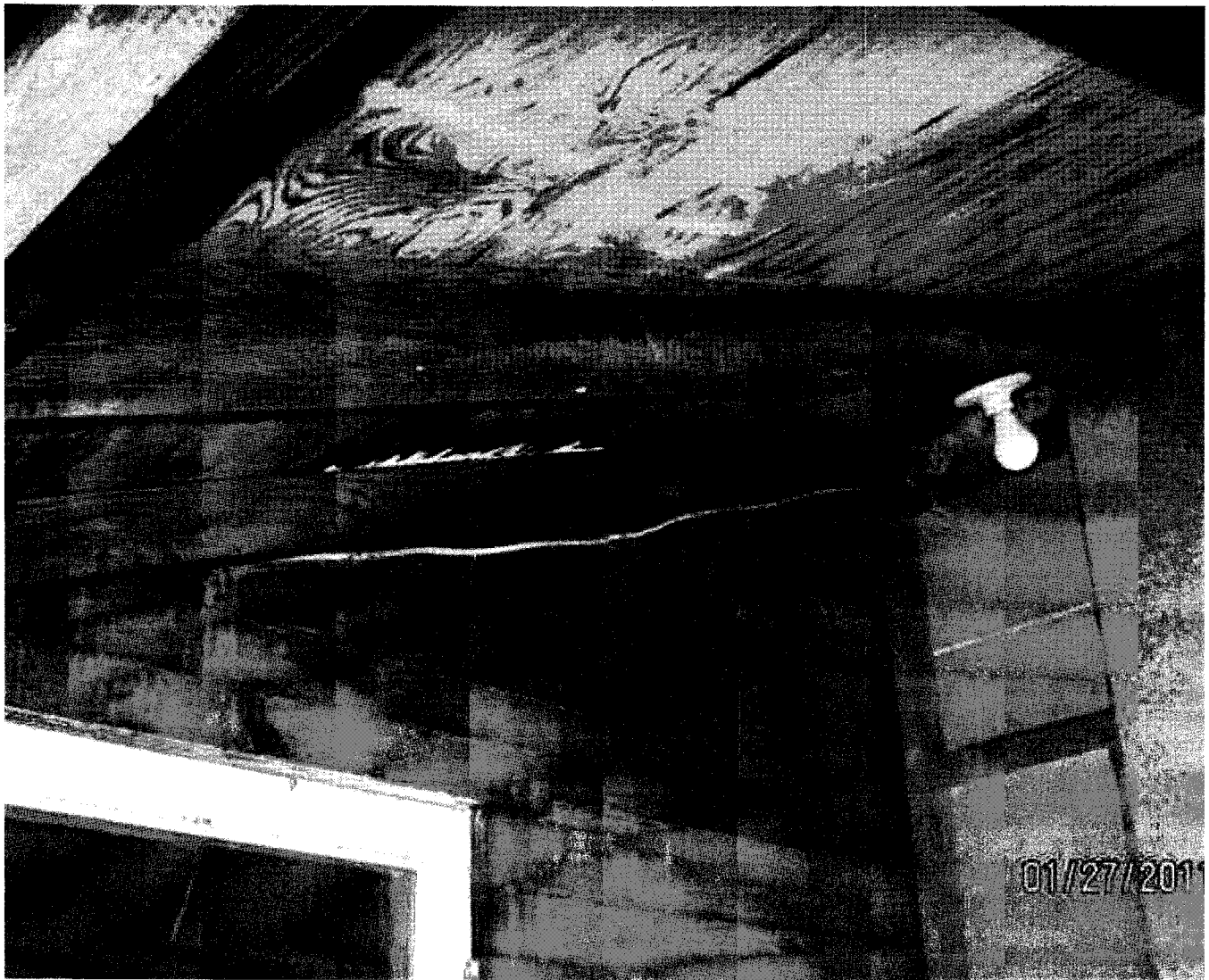
CForrey / SSS#2 - #12 Dampness causing mold and mildew - 01/27/2011
