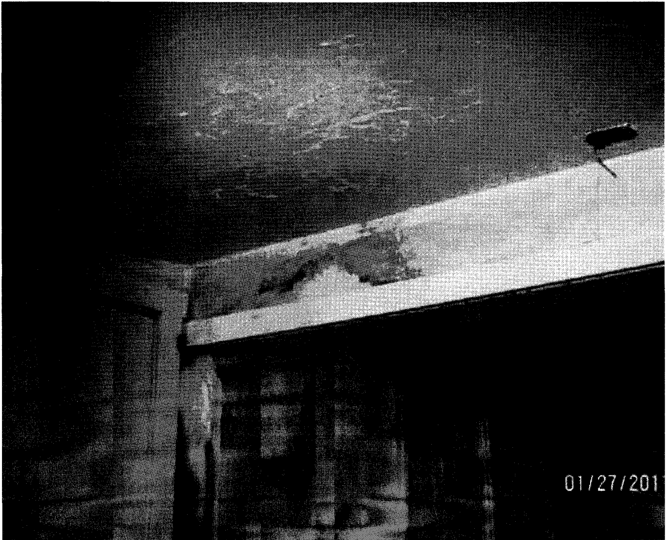
CForrey /SSS #1 Defect #12, 6 - Water damage, bare wires - 01/27/2011
