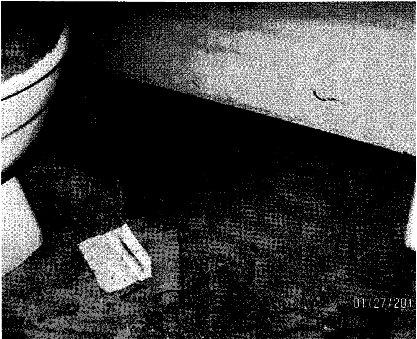
CForrey /SSS#2 Defect #8,9 - Bathroom floor sinking causing gap at base of bathtub - 01/27/2011
