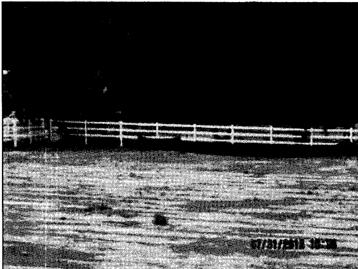
Wagner 80 - Section of silt fence along south property line.
