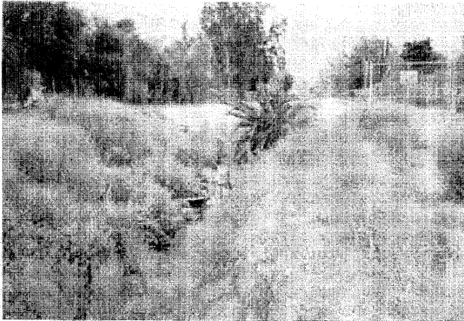
PHOTOGRAPH 3. This photograph depicts the North Norco Flood Control Channel on the east end of the channel as it transitions into the improved concrete channel. Photograph taken looking east on 9-11-2008.
