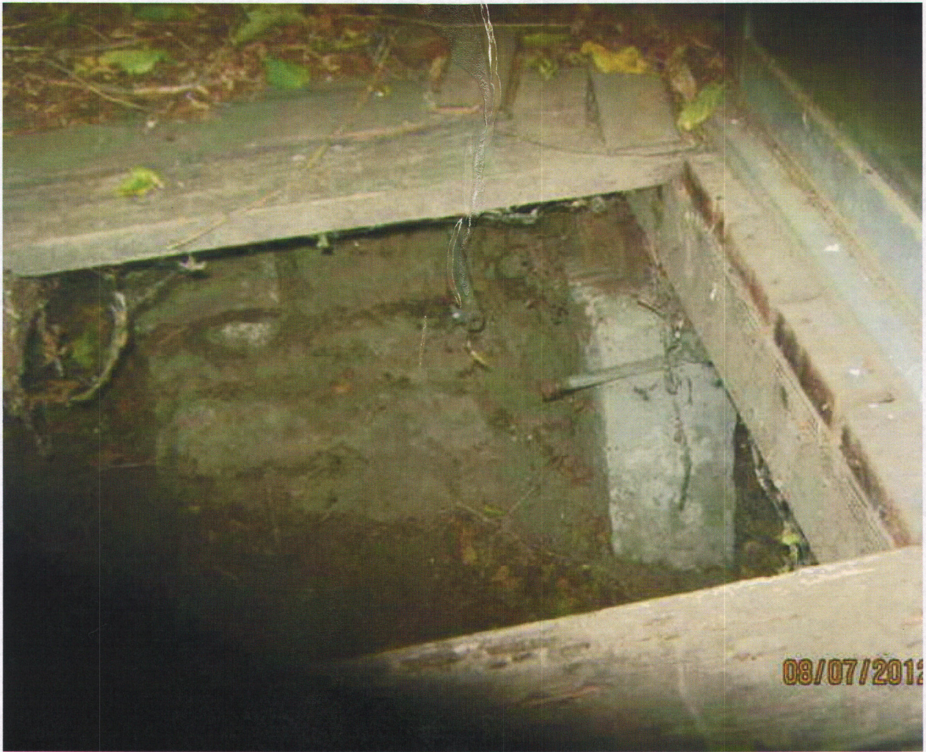
CForrey / Defect #8, 9 -Sink hole on s/w corner of house. - 08/07/2012
