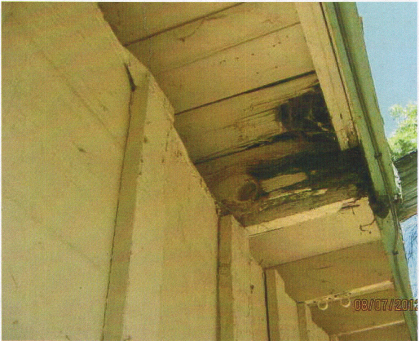
CForrey / Defect # 11, 14 - Rotted eaves, not maintained - 08/07/2012
