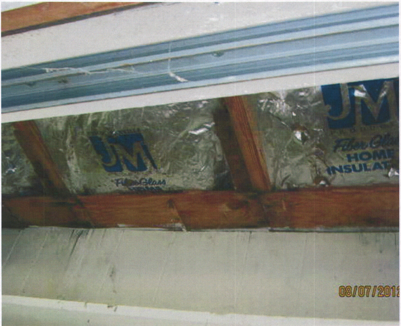
CForrey / Defect # 11 - missing ceiling drywall - 08/07/2012
