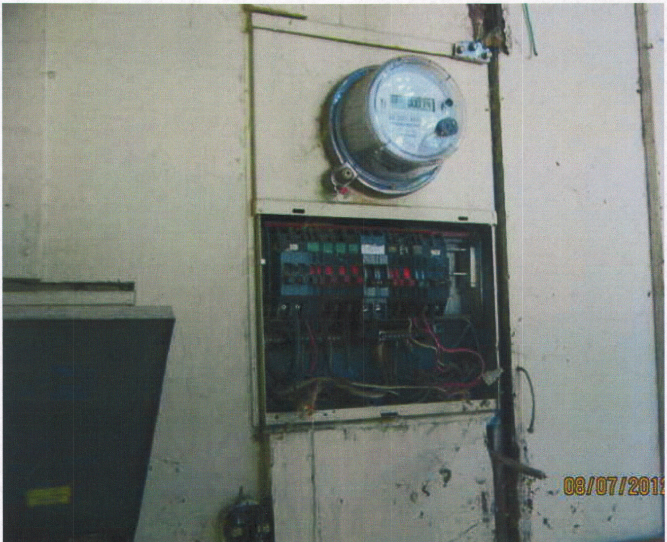
CForrey / Defect #6 - electric panel vandalized - 08/07/2012
