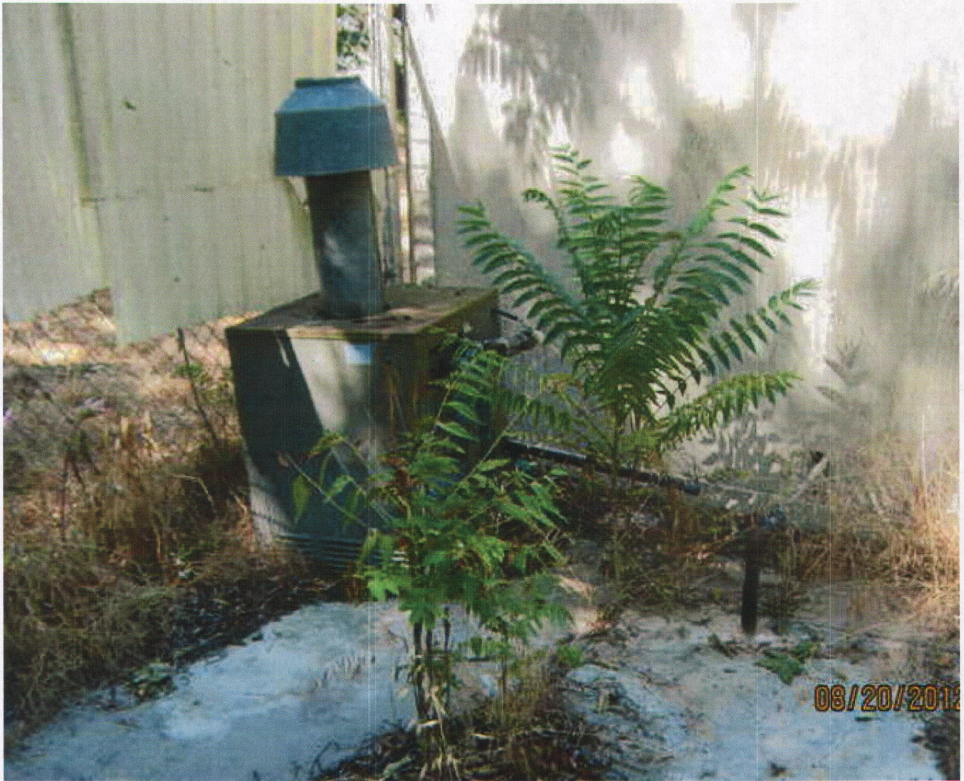
CForrey / Defect # 14 Pool equipment unmaintained - 08/20/2012
