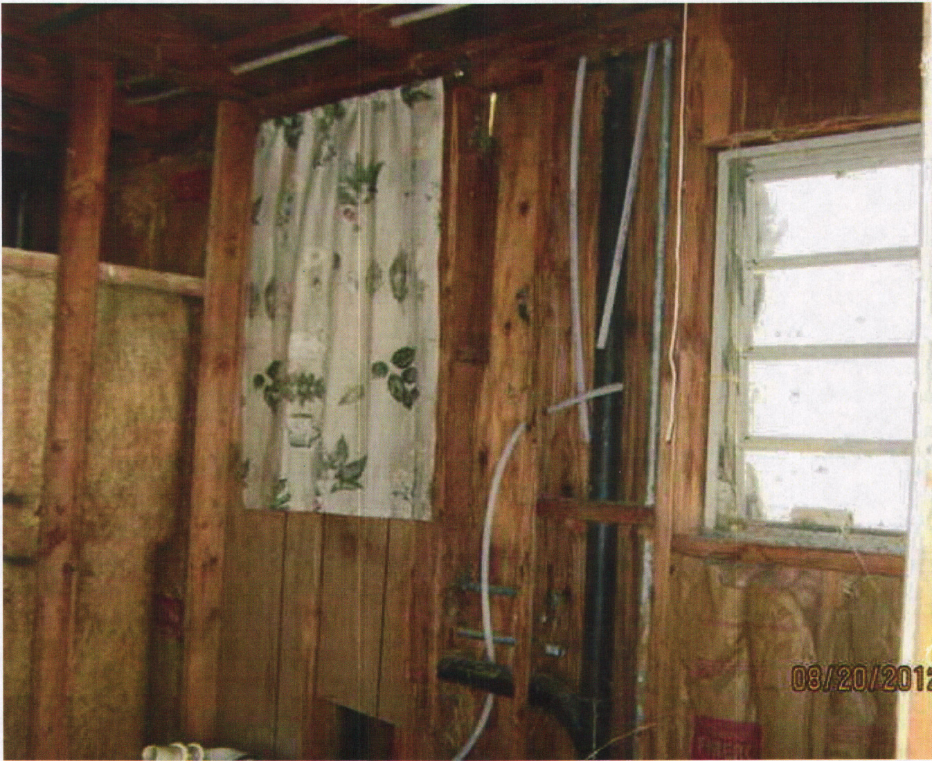
CForrey / C Forrey - Defect #6 Hazardous wiring - 08/20/2012
