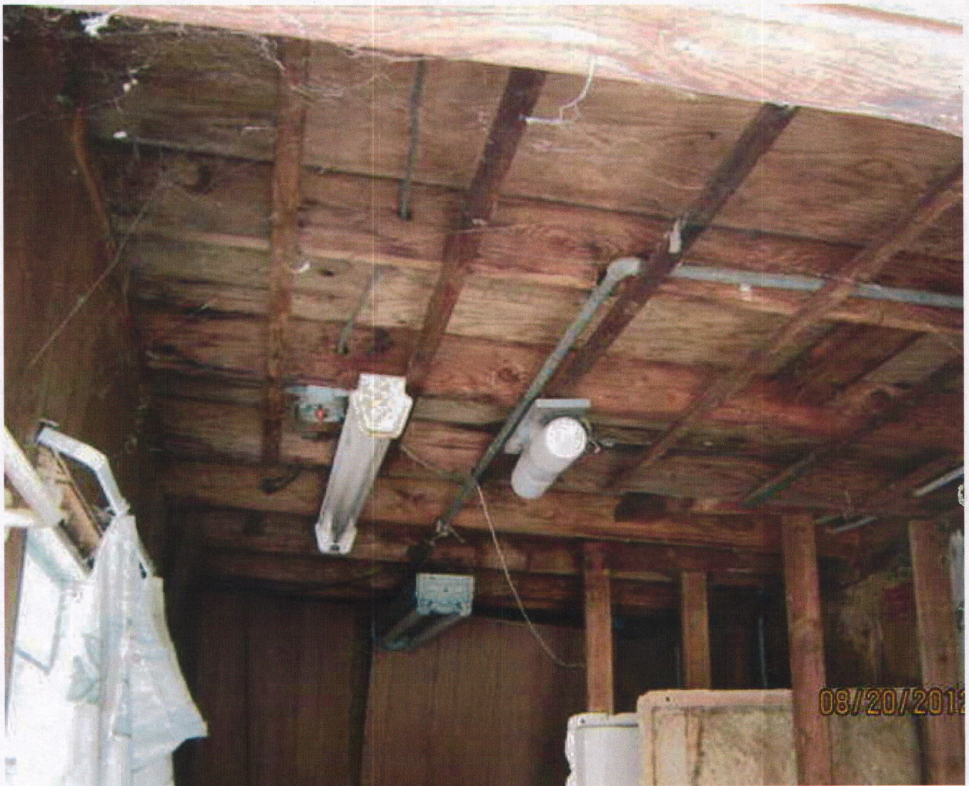
CForrey / Pool house - defect #10, 11, 12 - Dampness, deterioration - 08/20/2012
