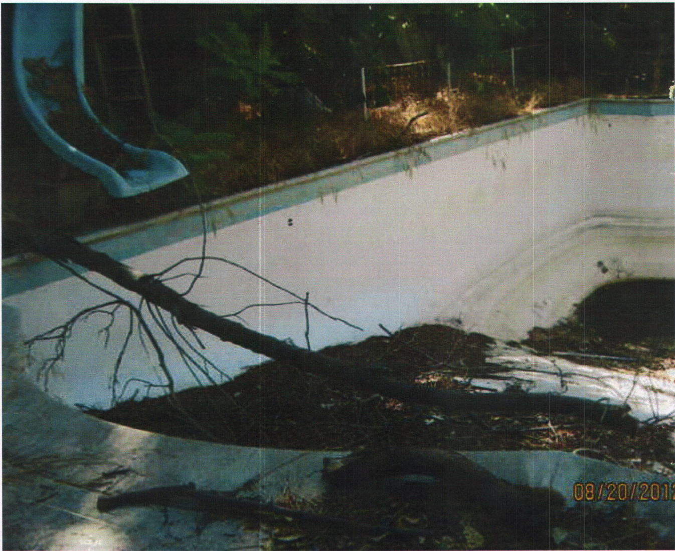
CForrey / Defects #17 - abandoned - 08/20/2012
