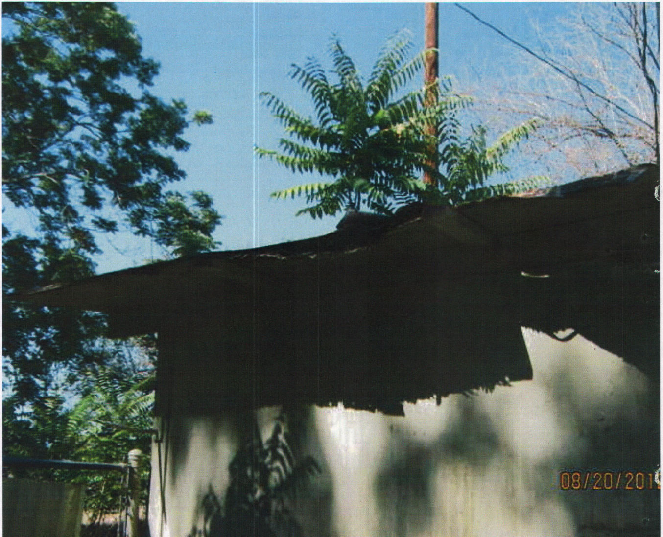
CForrey / Pool house - Defect # 11 - roof deteriorated - 08/20/2012
