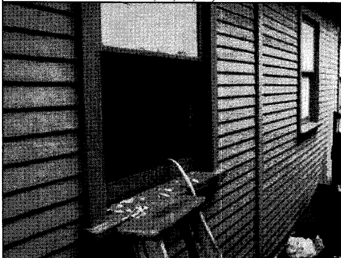
Structure #1- broken out window (Defect #14,13)
