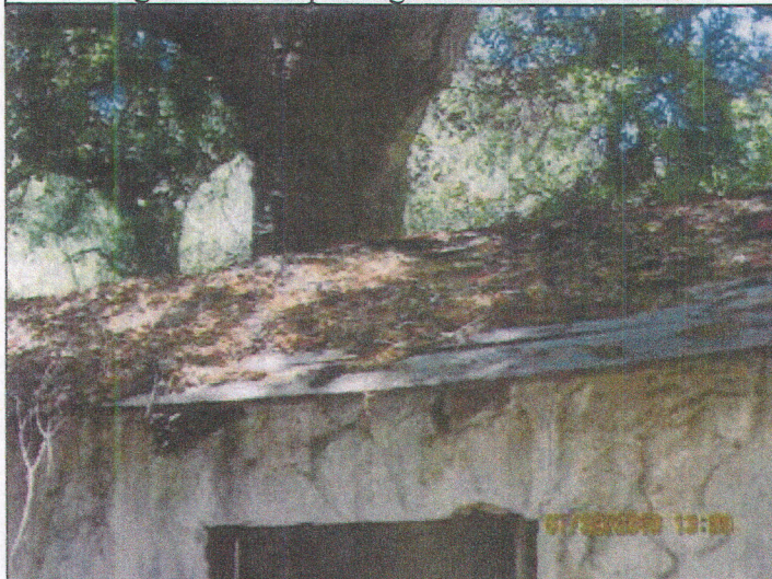
J.Wagner #80 Dilapidated roof
