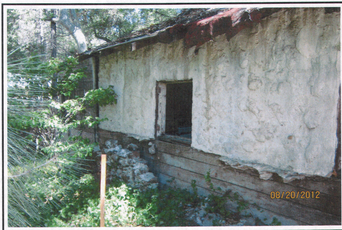
PHOTO # 8 NOTES: Faulty Weather Protection. Broken Window
