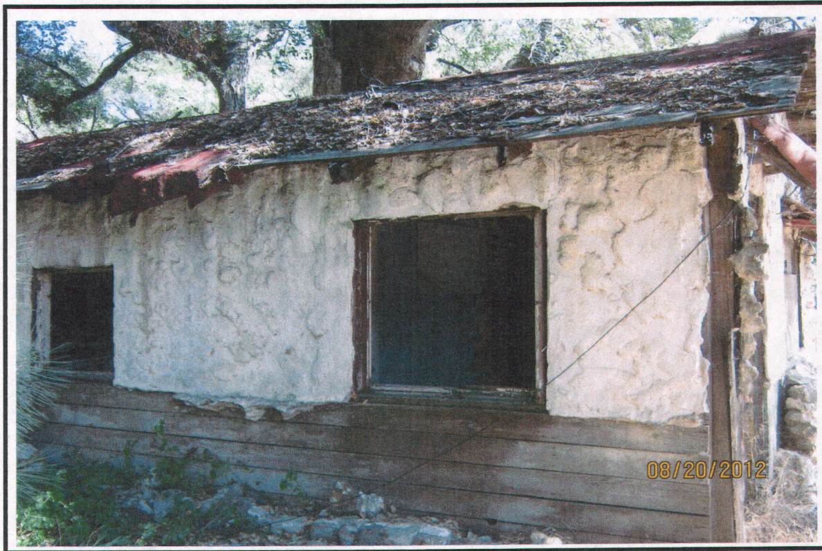
PHOTO # 7 NOTES: Faulty weather protection
