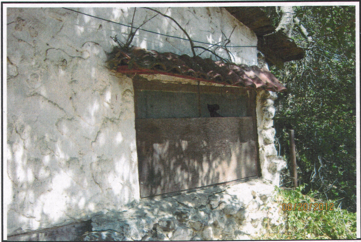
PHOTO # 5 NOTES: Front window partially boarded up. Window Broken #13, #17
