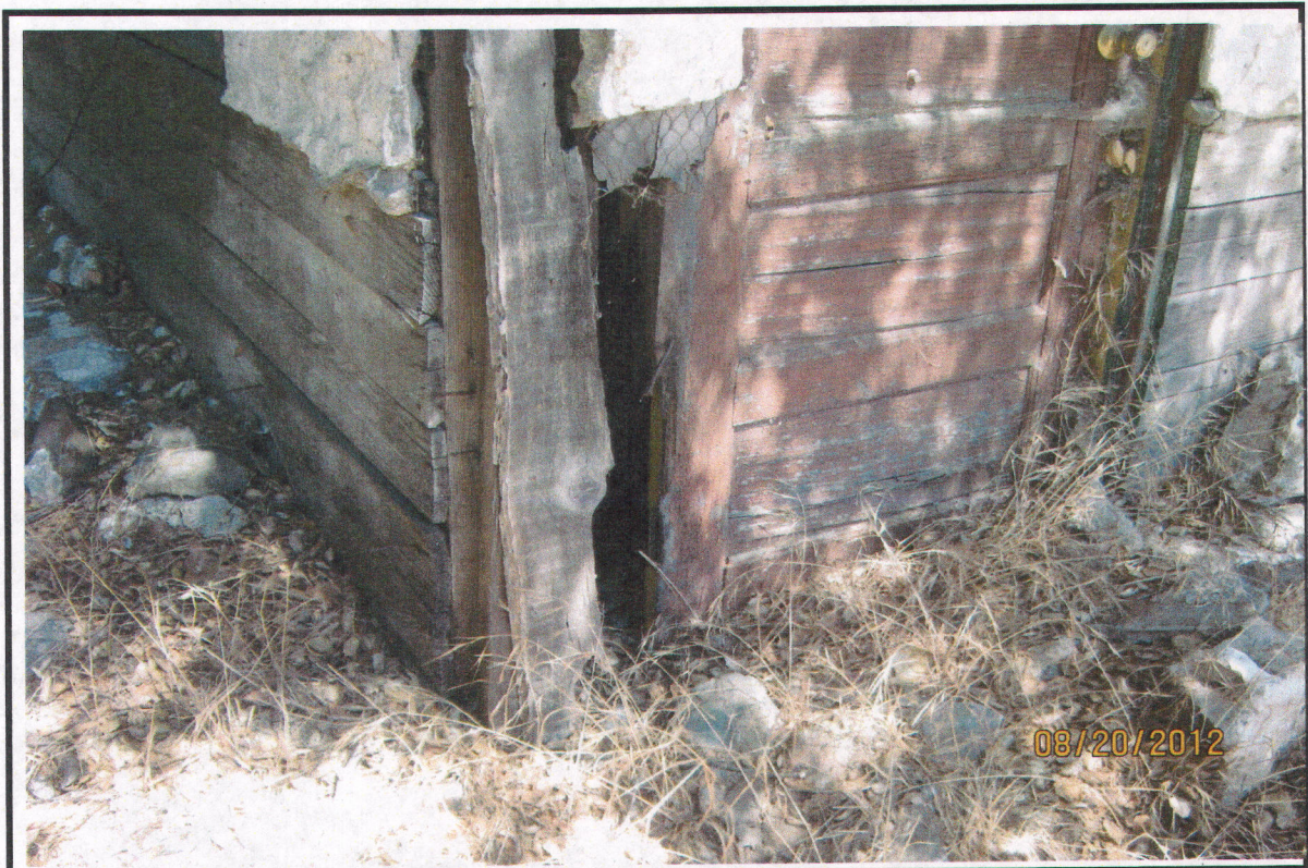
PHOTO # 6 NOTES: Large opening Near Front Door #10, #14
