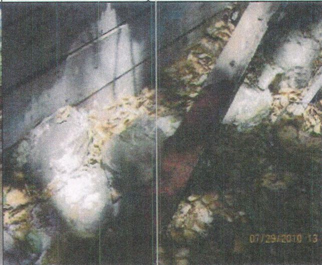
J.Wagner #80 Fallen roof material
