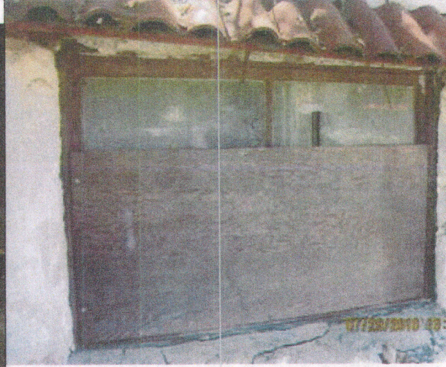
J.Wagner #80 Front window partially boarded up Window broken.
