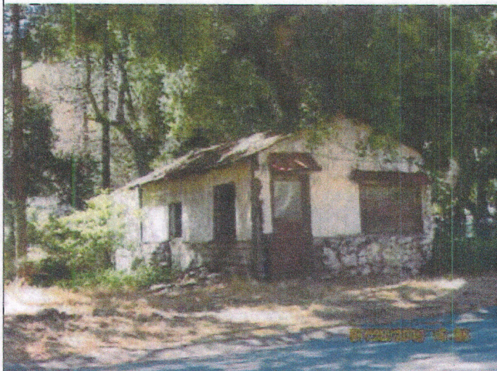
J.Wagner #80 Depicting substandard structure.
