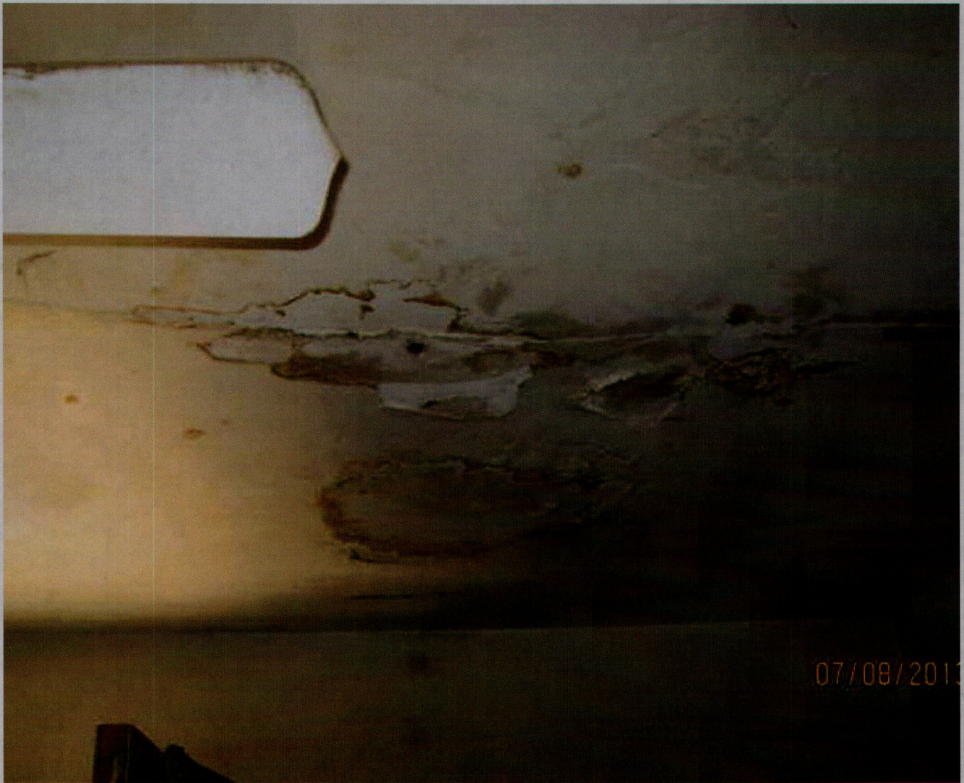
Photo #3 - defects 11,13 and 14 - 07/08/2013
