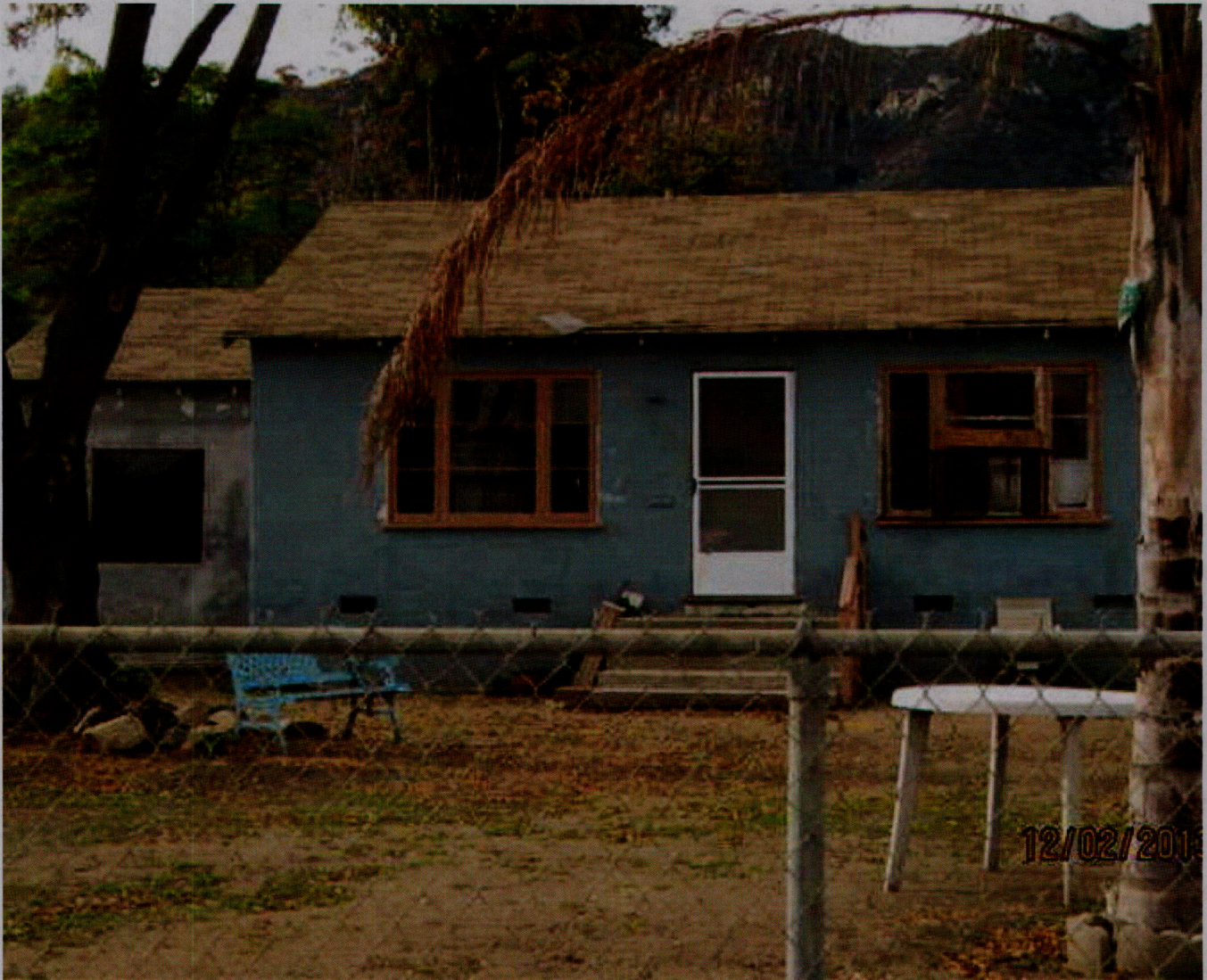
Photo #1 Substandard structure - 12/02/2013
