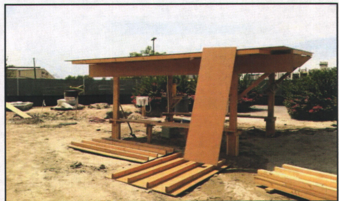
Figure 12. August 01, 2014: 115 Degree Weather requires Shade, Water and Misters for the MBC Construction Crew
