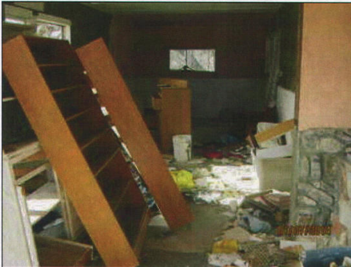
AR remains and structure substandard. 1 of 5.
