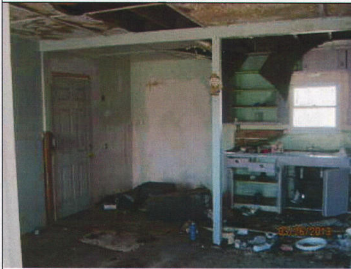
Substandard structure and AR remain. 1 of 7.
