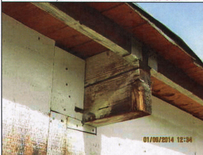
Cracked Roof Beam 1/9/14 J. Cole
