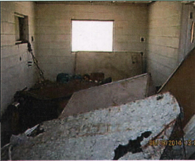
Rubbish Inside the Substandard Structure 6/19/14 Cole
