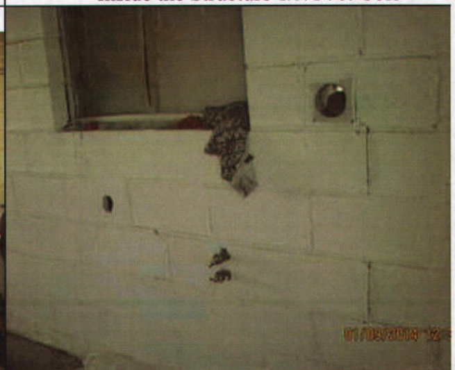
Inside the Structure, Missing Plumbing Fixture 1/9/14 J. Cole
