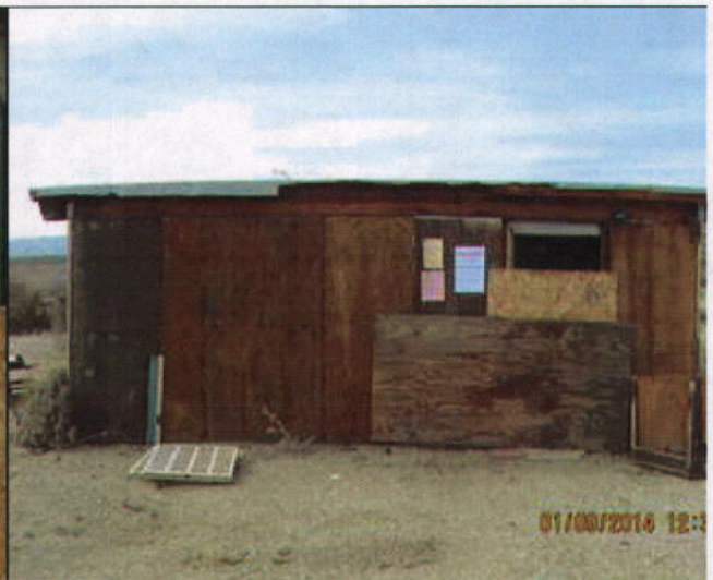
Substandard Structure 1/9/14 J. Cole
