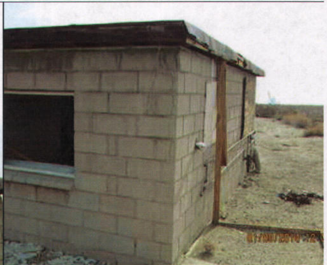
Damaged Exterior Walls, Northwest Corner 1/9/14 J. Cole
