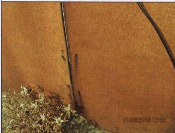
Warped Exterior Wall 1/9/14 J. Cole
