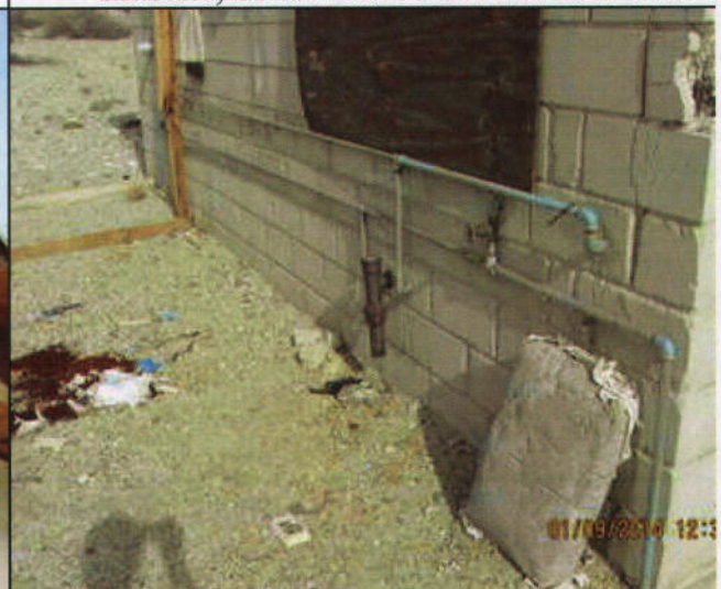
Damaged Exterior Wall (West Side) 1/9/14 J. C
