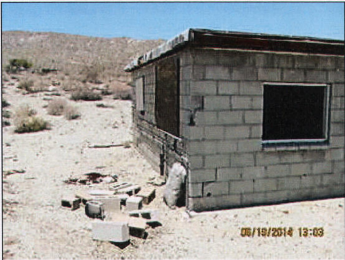
Southwest Corner of the Structure and rubbish 6/19/14 J. Cole
