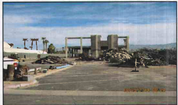
Figure 6. August 25, 2014: CAC Building - Partial Second and First Floor Remaining
