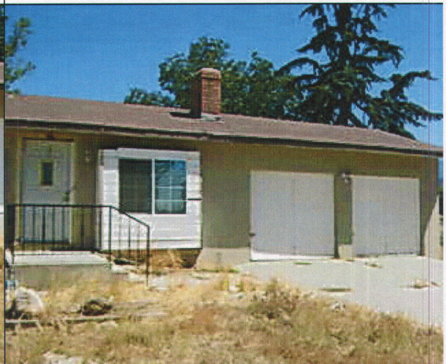
08/09/13 - Substandard Structure NOD# 11, 13, 17 - Pike
