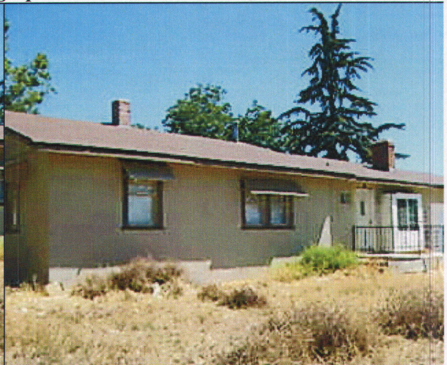
08/09/13 - Substandard Structure NOD# 11,13, 17 - Pike
