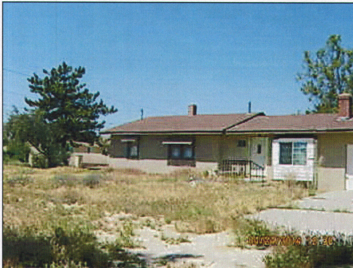
Substandard Structure remains. J. Palmer
