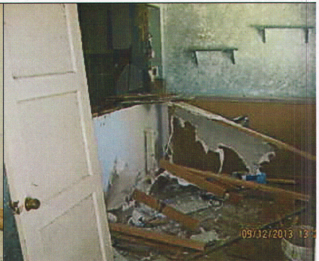
Substandard Structure, interior. J. Palmer
