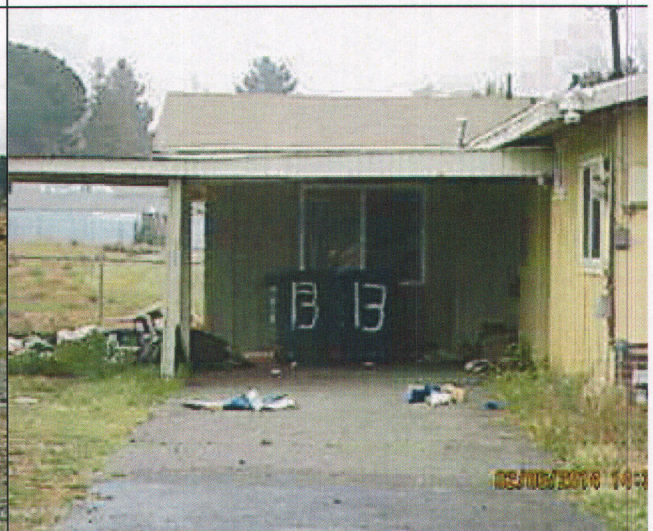
Accumulated Rubbish and CWP- Garage Conversion remain. J. Palmer
