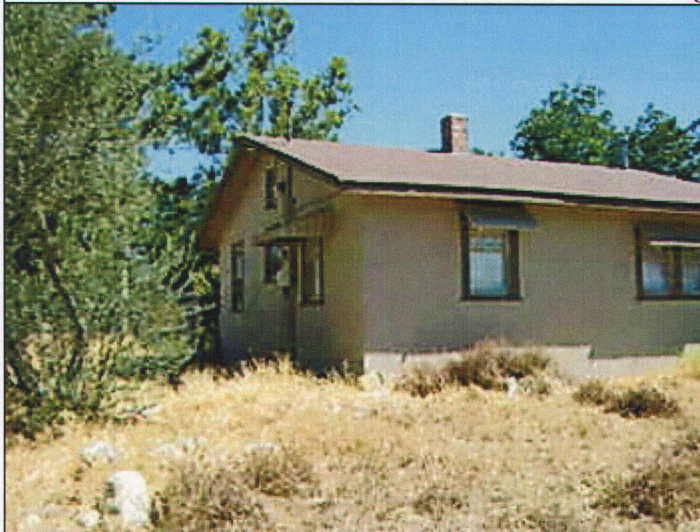
08/09/13 - Substandard Structure NOD# 11,13, 17 - Pike
