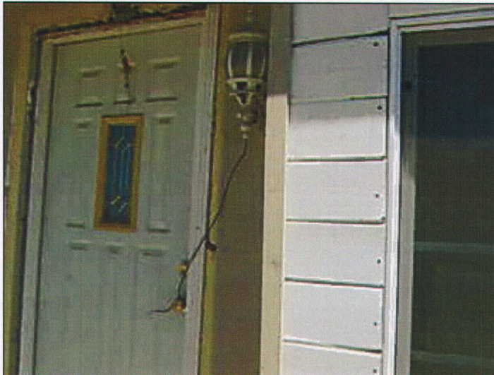
08/09/13 - Substandard Structure NOD# 17 - Pike
