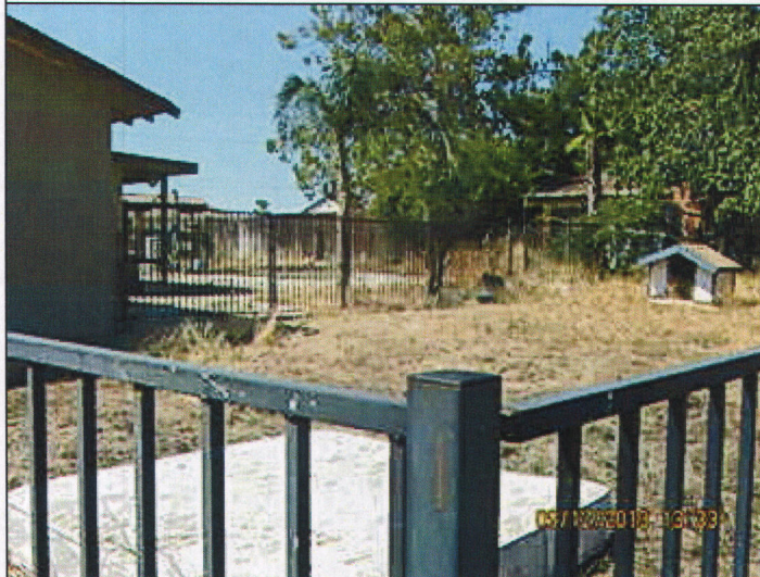
Substandard Structure/Accumulated Rubbish remains. J. Palmer
