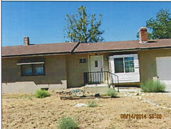
007.JPG Rubbish removed, Substandard Structure remains. J. Palmer
