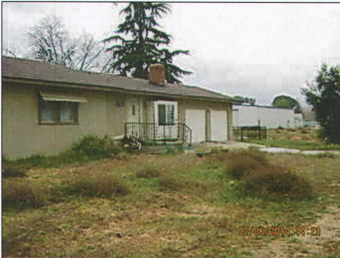
Substandard Structure remains. J. Palmer
