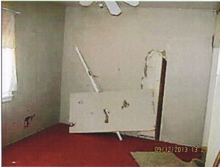
Substandard Structure, interior. J. Palmer
