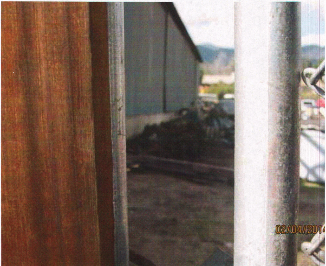
Photo #2 - accumulated rubbish/outdoor storage - 02/04/2014
