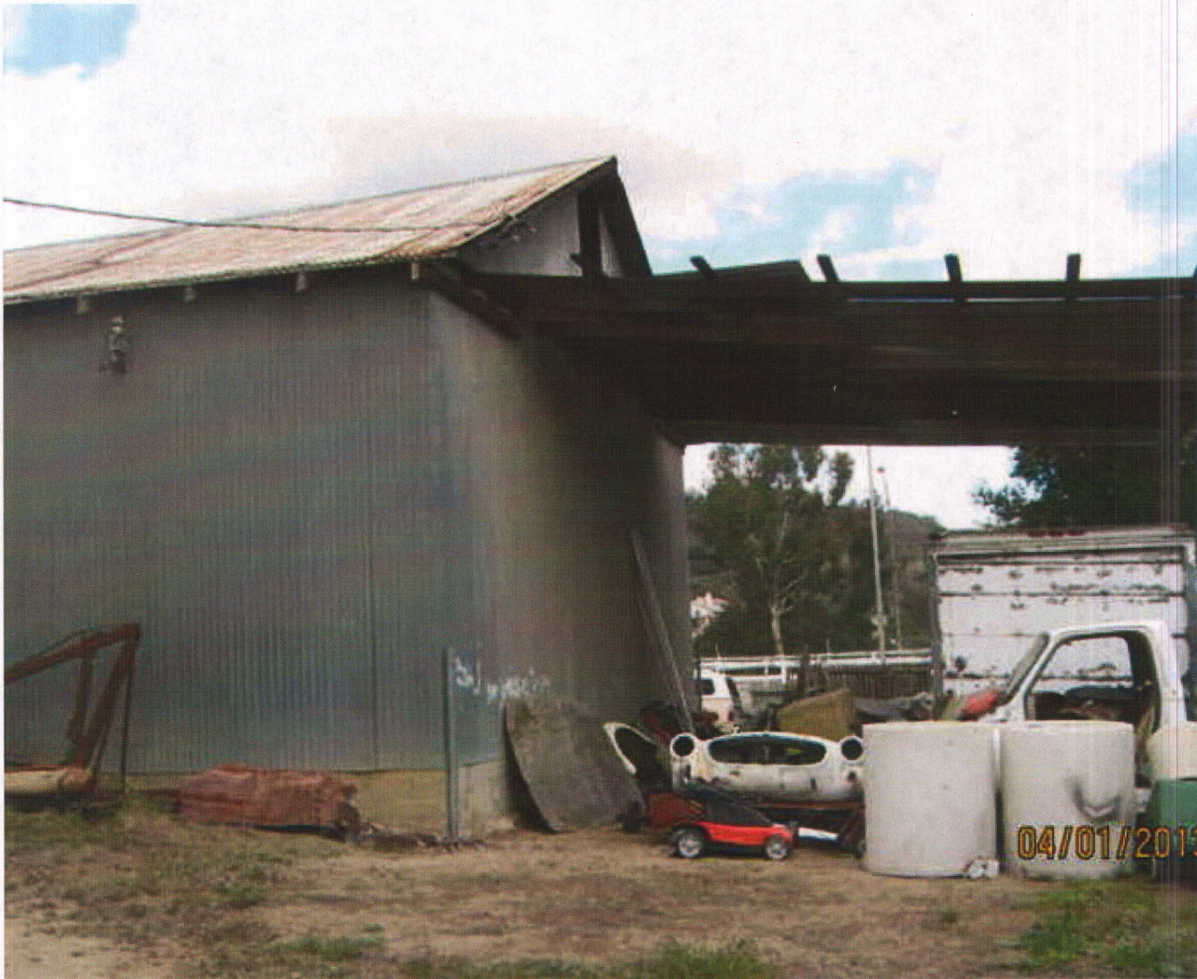
Photo #5 - accumulated rubbish/outdoor storage - 04/01/2013
