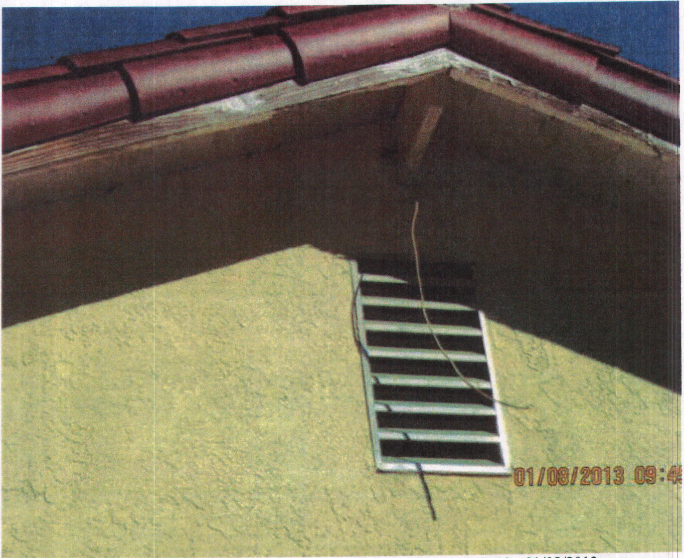
E. Torres; substandard structure #3- defects 6, 14, 17, 19 - 01/08/2013
