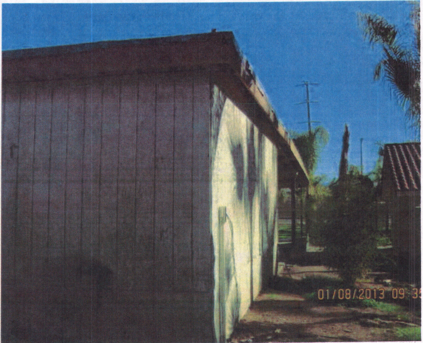
E. Torres; substandard structure #4- defects 6, 14, 17, 19 - 01/08/2013
