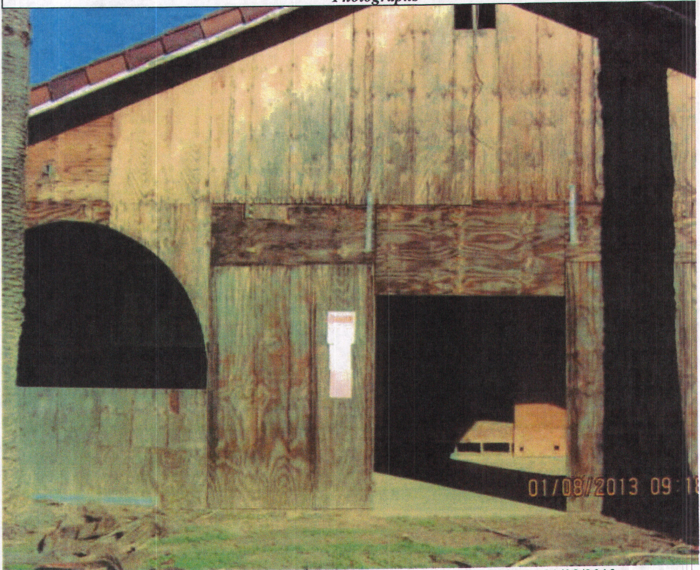
E. Torres; substandard structure #1- defects 12, 13, 14, 17 - 01/08/2013
