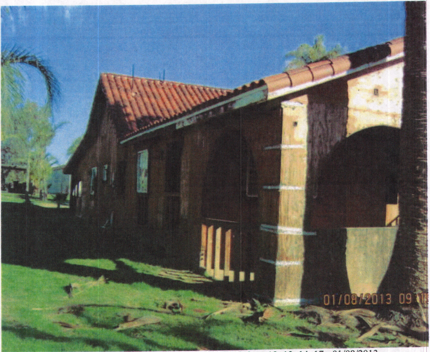
E. Torres; substandard structure #1- defects 12, 13, 14, 17 - 01/08/2013
