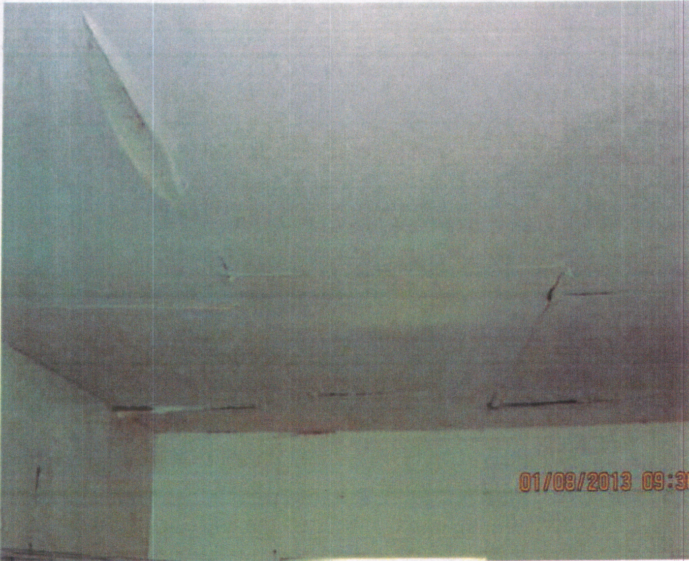
E. Torres; substandard structure #4- defects 11, 13, 14, 17, 19 - 01/08/2013
