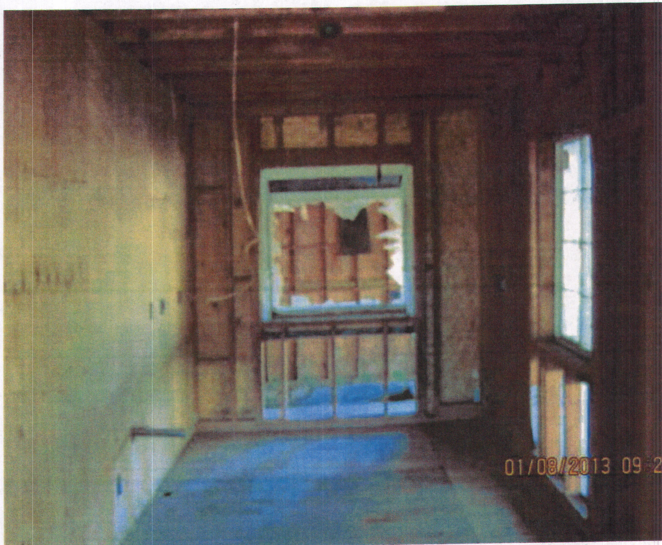
E. Torres; substandard structure #1- defects 12, 13, 14, 17 - 01/08/2013
