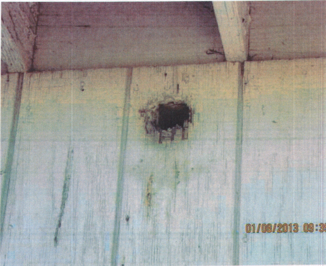
E. Torres; substandard structure #4- defects 13, 14, 17, 19 - 01/08/2013
