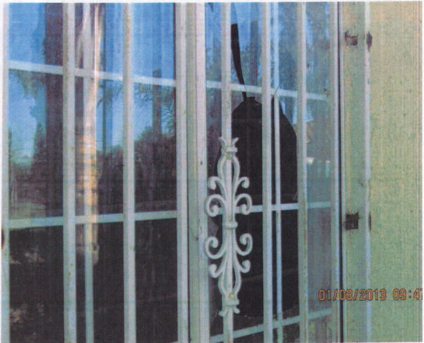
E. Torres; substandard structure #3- defects 12, 13, 14, 17, 19 - 01/08/2013
