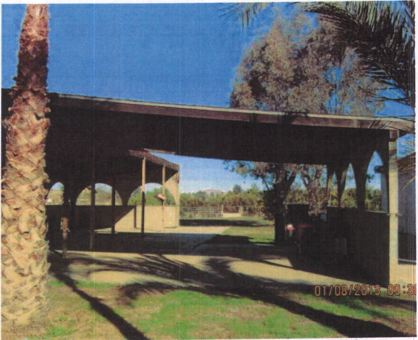
E. Torres; substandard structure #2- defects14, 17, 19 - 01/08/2013
