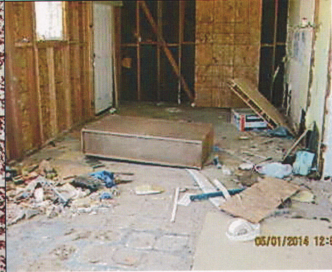
Damaged Interior Walls 5/1/14 J. Cole
