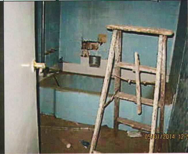
No Plumbing Fixtures 5/1/14 J. Cole
