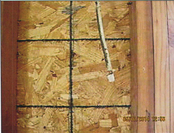
Electrical Wire 5/1/14 J. Cole
