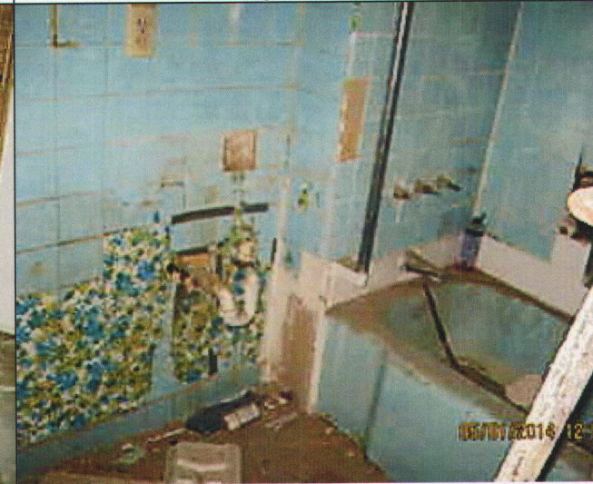
No Plumbing Fixtures 5/1/14 J. Cole
