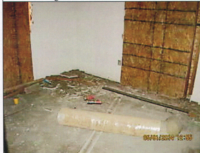
Damaged Interior Walls 5/1/14 J. Cole
