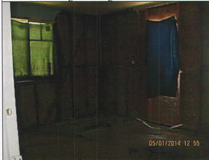
Damaged Interior Walls 5/1/14 J. Cole
