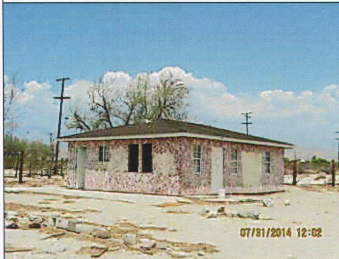
Substandard Structure 7/31/14 J. Cole
