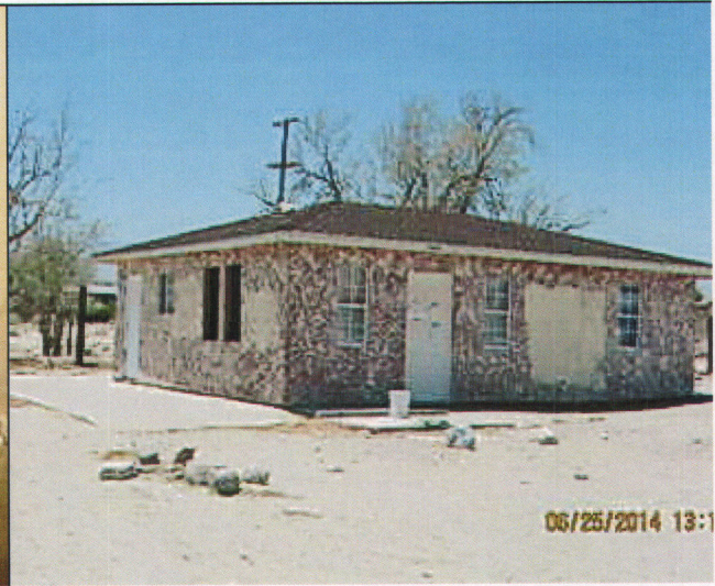
Substandard Structure 6/25/14 J. Cole
