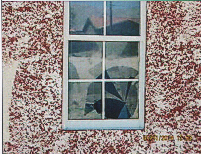
Broken Front Window 5/1/14 J. Cole
