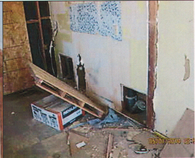
Damaged Interior Walls 5/1/14 J. Cole
