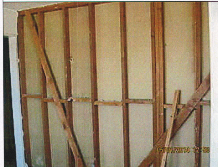
Damaged Interior Walls 5/1/14 J. Cole
