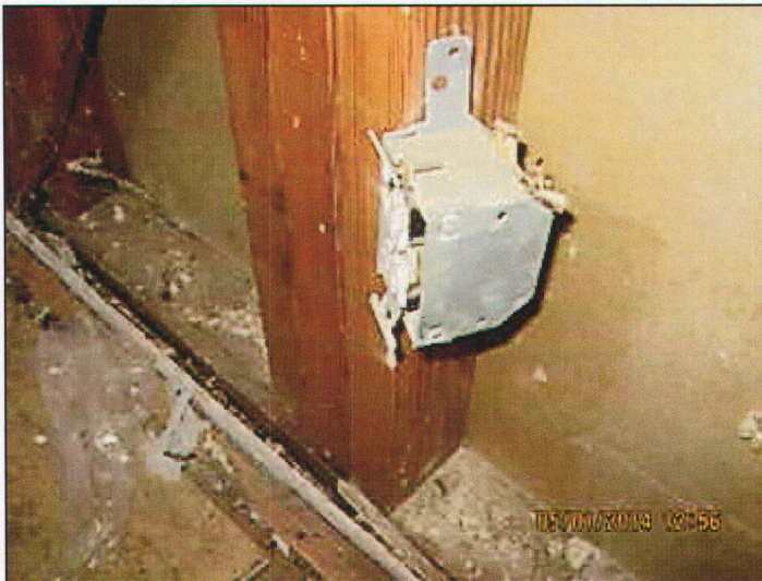
Electrical Outlet 5/1/14 J. Cole
