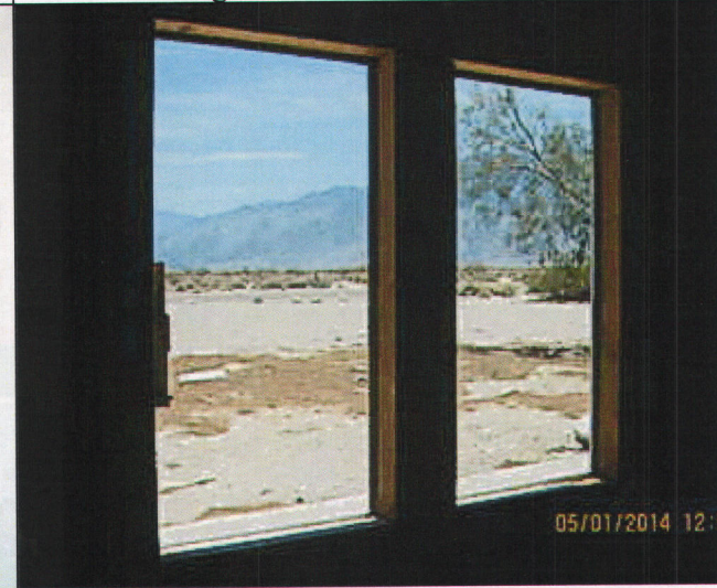
Missing Windows 5/1/14 J. Cole
