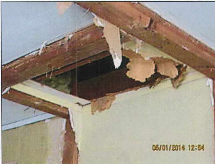
Damaged Ceiling 5/1/14 J. Cole
