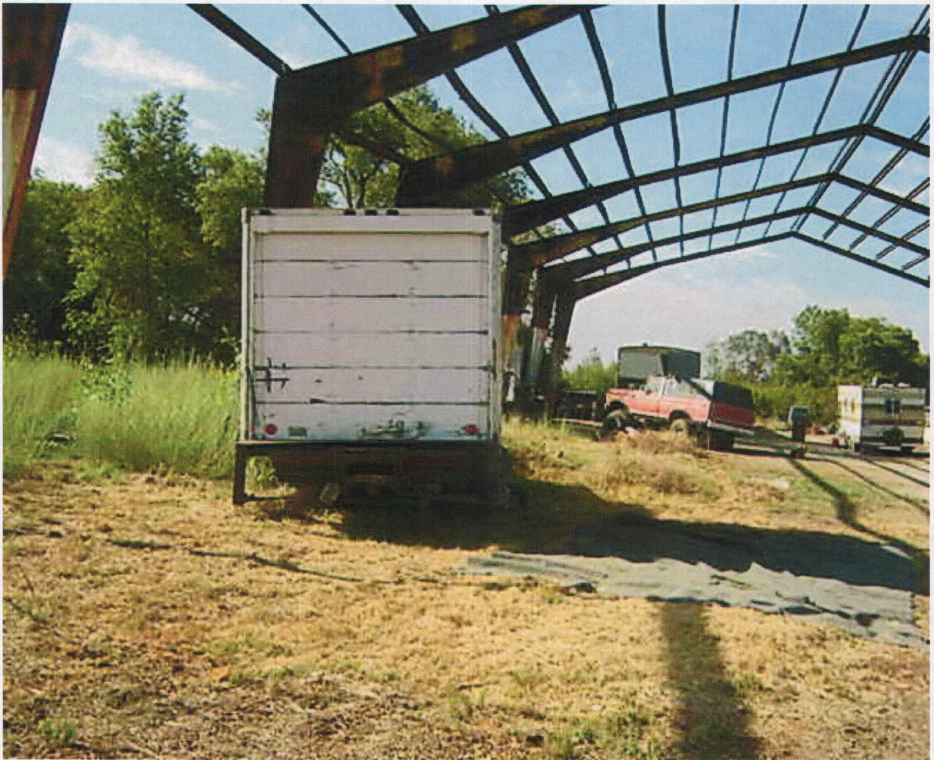
Excessive outside storage-JMorris 8/2/13 - 08/02/2013
